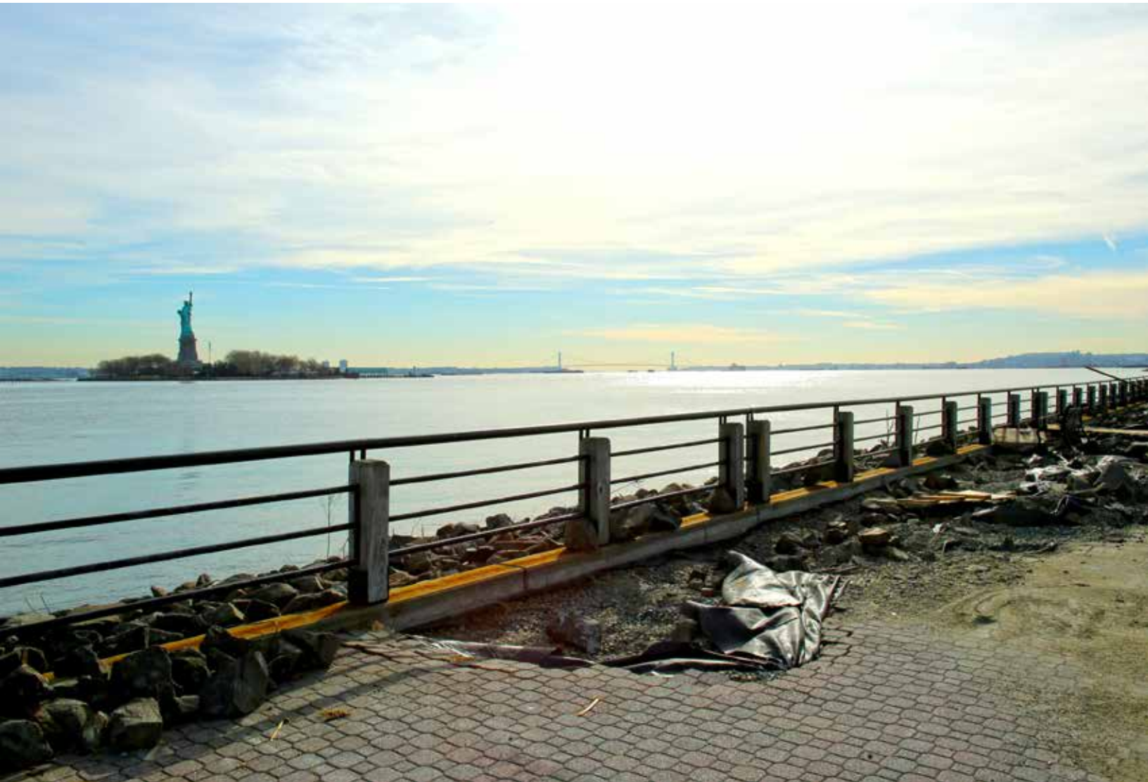
Damage caused by storm surge, Jersey City, NJ, 2012.
