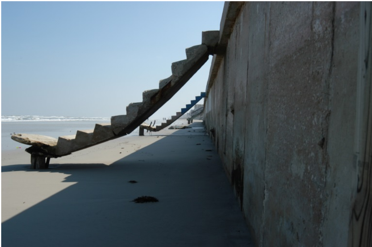
Figure 3-15: Seawall. This seawall on New Smyrna Beach, Florida, was mostly hidden by sand prior to the arrival of Hurricane Jeanne in 2004. FEMA Photo/Mark Wolf.
