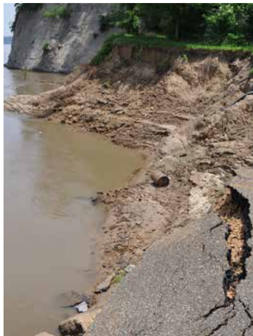
Washed-out landing in Tipton County, TN, 2011.
