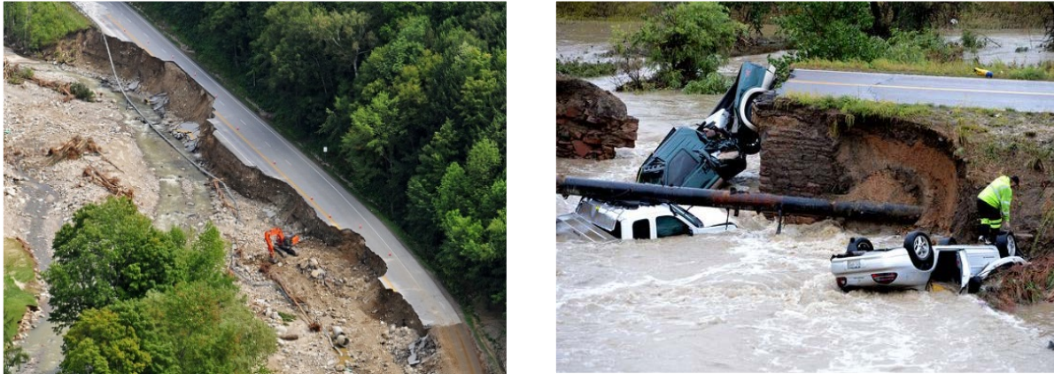
Figure 3-1: Channel Changes, Erosion, and Deposition. Left shows channel changes on Vermont Route 107 resulting from Hurricane Irene (Photo: Vermont Agency of Transportation). Right shows changes after flash flooding at the in Colorado (Photo: Cliff Grassmick, AP).
