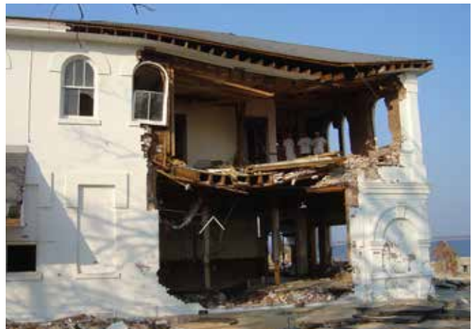
Hurricane damage, Mississippi, 2005.
