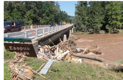
Figure 3-32: Debris on a Bridge
