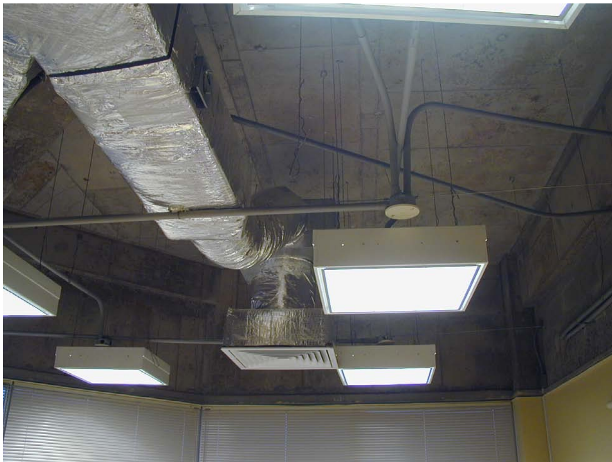
Figure 6.4.9.1-2 Overhead lights with four vertical hangers to the structure. Unbraced acoustic ceiling system was damaged beyond repair in the 2001 magnitude-8.4 Peru Earthquake but none of the diffusers or lights fell because they had independent supports. Ceiling was demolished prior to photo (Photo courtesy of Eduardo Fierro, BFP Engineers).
