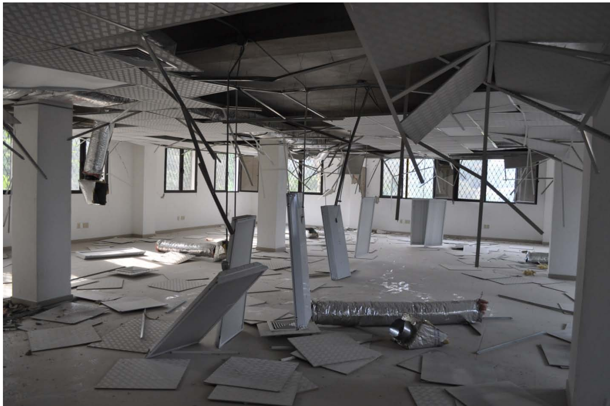
Figure 6.4.9.1-1 Numerous fluorescent fixtures dangling from electrical conduit; installed without safety wires in unbraced suspended acoustical ceiling and damaged in the 2010 magnitude-7 Haiti Earthquake. Loose bulbs, lenses, ceiling panels, diffusers and ducts also on the floor (Photo courtesy of Ayhan Irfanoglu, Purdue University).
