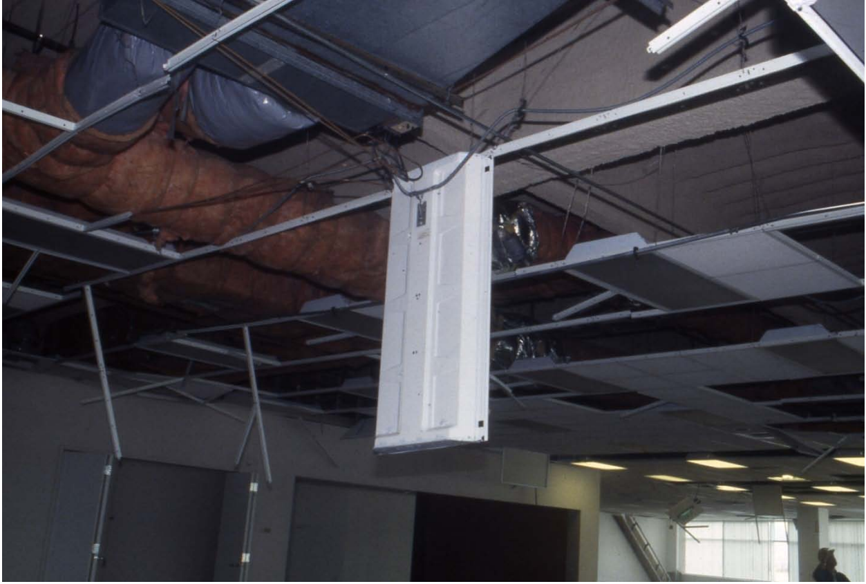
Figure 6.4.9.1-3 Light fixture without adequate independent support dangling along one edge from ceiling grid, damaged in the 1994 magnitude-6.7 Northridge Earthquake (Photo courtesy of Degenkolb Engineers).
