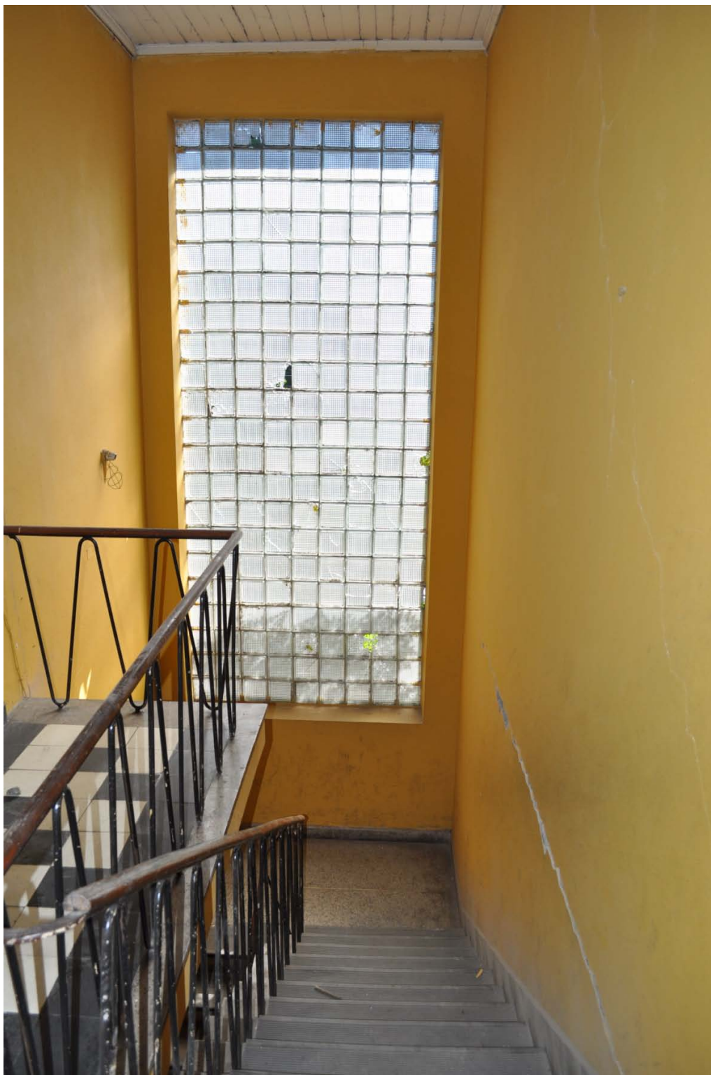
Figure 6.3.1.5-2 Damage to glass block with rigid mortar on all sides and in all joints in the 2010 Chile Earthquake (Photo courtesy of Eduardo Fierro, BFP Engineers). About 25% of the glass block units are cracked or broken but entire panel will need to be removed and replaced.
