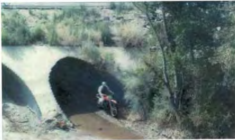
CYC Access Road Culverts circa 1978 -- wash silted in more than 8 feet
