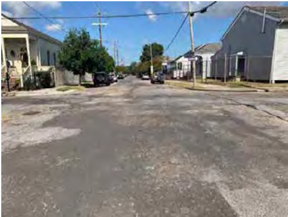
Figure 20: Typical conditions of Philip Street, as seen from its intersection with Chippawa Street facing north, where the road reconstruction with bioswales is proposed
