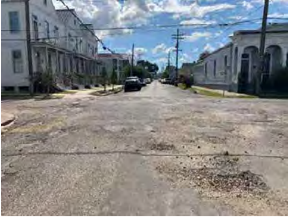
Figure 21: Typical conditions of Philip Street, as seen from its intersection with Chippewa Street facing south, where the road reconstruction with bioswales is proposed
