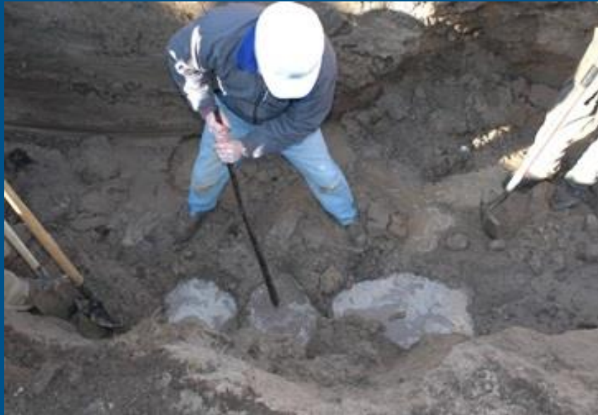
Steel rod used to break through the hardpan layer exposed in a trench. Note upward flowing water under pressure.
