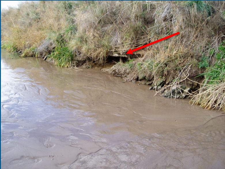
Hardpan layer several inches thick in the incident area on the dam side of South Drain
