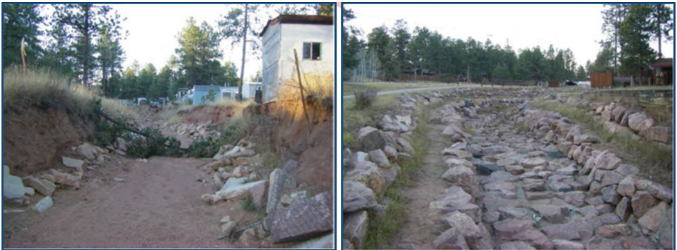
Figure 2. Example of project site photos of a streambank stabilization project along Fountain Creek, Woodland Park, Colorado. The photo to the left shows the eroded downstream reach while the photo to the right shows the already stabilized upstream reach.
