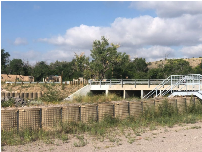
Figure 3. An example of a bridge project along Santa Clara Creek. The wider span of the bridge will allow for higher volumes of water flow in future flood events. In addition, angled bridge components will redirect water flow to protect vulnerable infrastructure. Hesco bastions were also added and are visible in the foreground of this photo. These flood control barriers can help protect residential areas from dangerous floodwaters. Source: FEMA Interagency Coordination Division (ICD).
