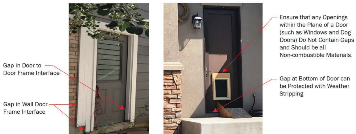
Figure 18. Examples of door-to-wall joints. Where openings in the plane of a door exist, such as dog doors or windows, the gaps around the openings should be filled caulking, mineral wool, or similar non-combustible material. In addition, the opening itself should be protected from ember intrusion that can be deployed during a wildfire incident (e.g., provide a noncombustible shutter).
