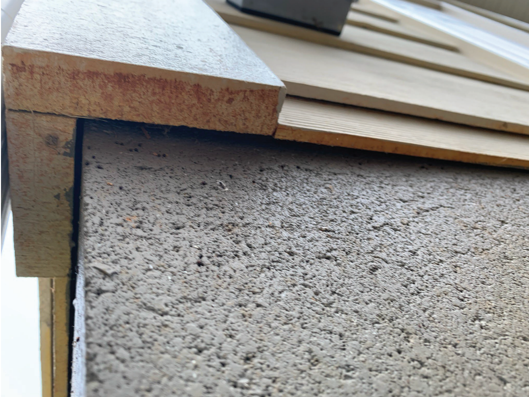
Figure 4. Homeowners should block gaps between siding and foundations (such as the one pictured here) using firestopping materials such as mineral wool or fire-resistant sealants to prevent embers, hot gases, and flames from entering and becoming trapped.
