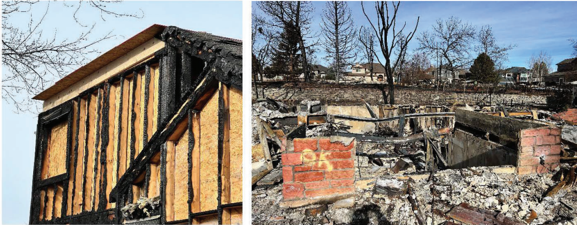
Figure 1. Examples of damaged wall assemblies.
