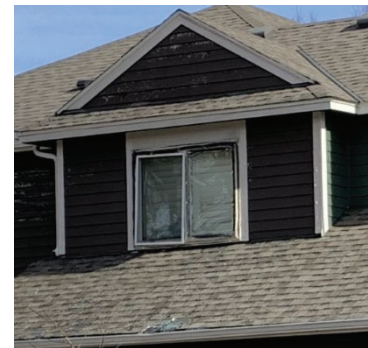
Figure 5. Example of glazing system failures.
