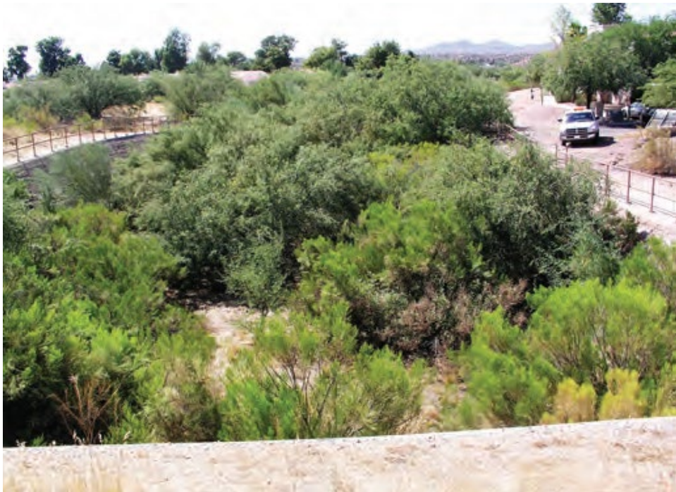
Figure 13. Picture of a constructed channel in Arizona that is overgrown with vegetation (from U.S. Geological Survey Scientific Investigations Report 2006-5108)
