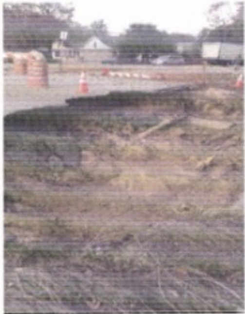
Figure 2 - Erosion of Eastern Dam Section
