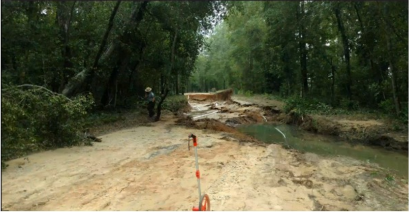
Figure 7 – 2018 Damage Photos showing scour along access road
