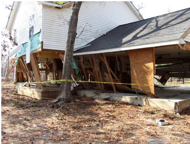
Figure 5-2: Wave and surge damage to load-bearing walls atop stem wall foundation approximately 0.5 mile from shoreline
