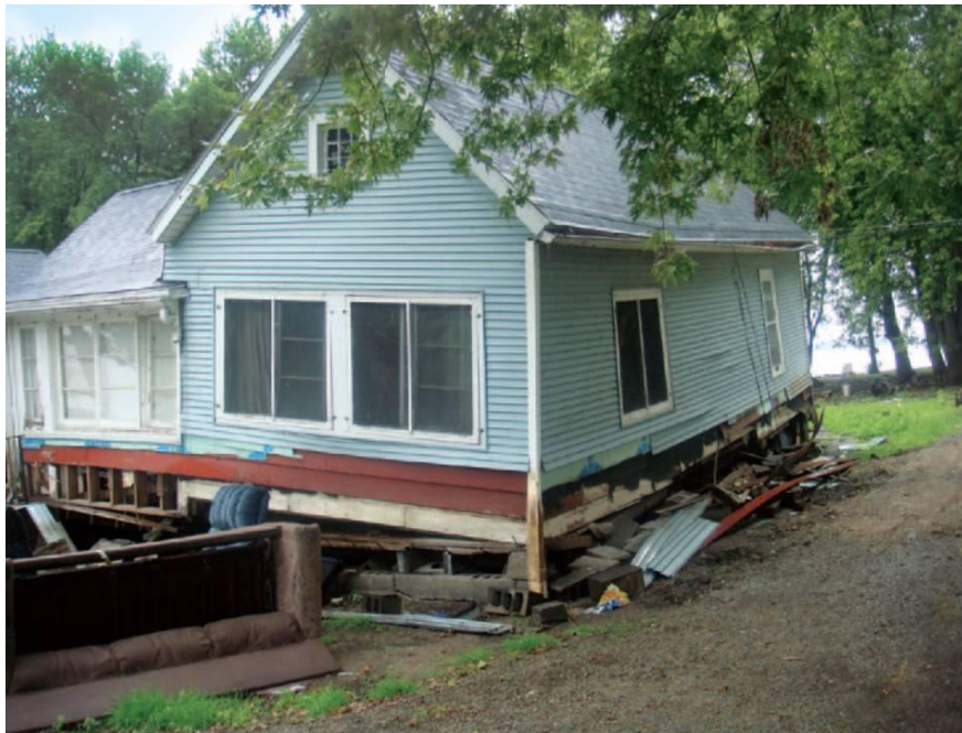
Figure 5-1: Pre-FIRM foundation that was exposed to hydrodynamic forces as wind-driven waves flowed from a lake into a nearby river
