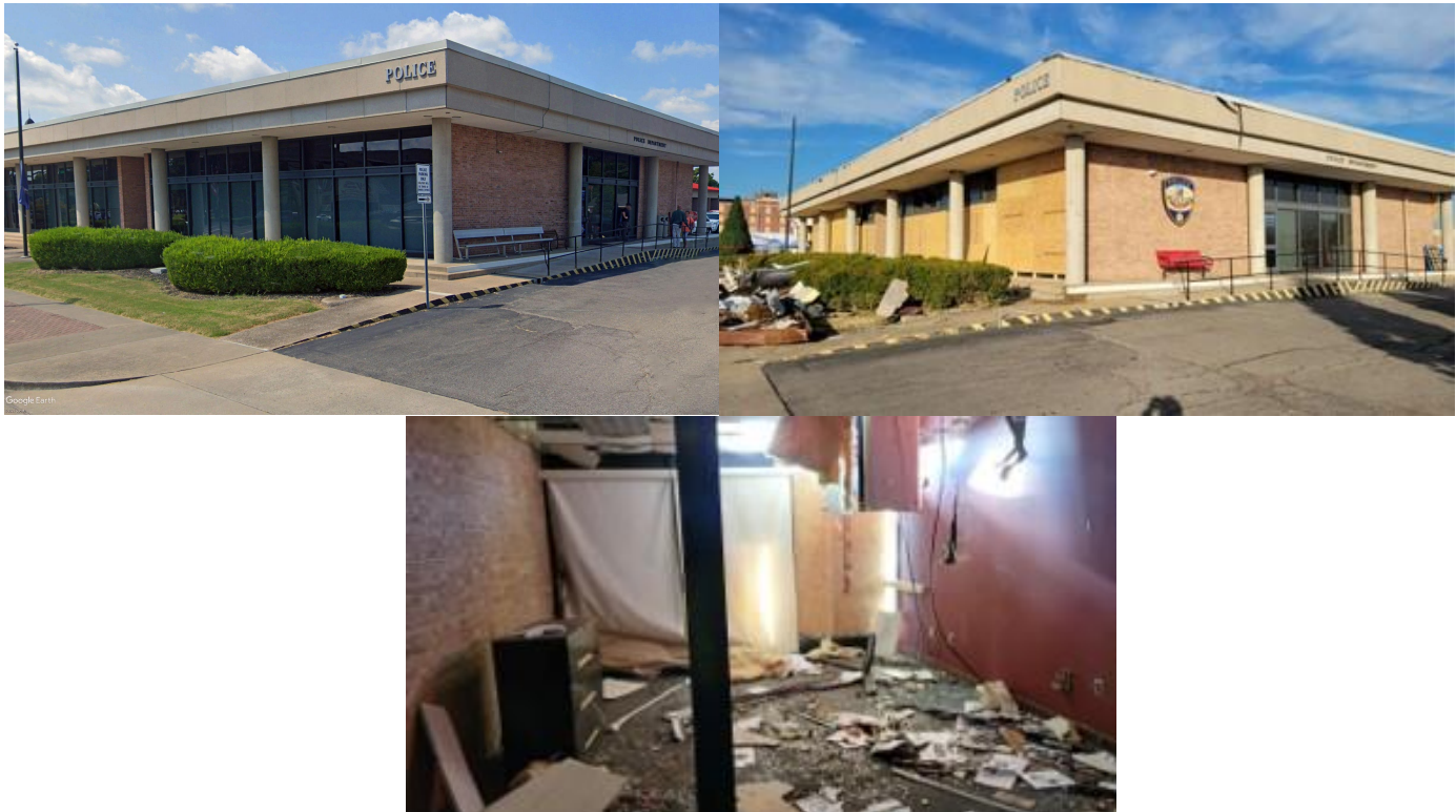
Figure 1: Mayfield, KY Police Station – Concrete building performed well structurally, but glazing failed in many locations; 75 people took shelter in the basement and communications were lost. Top left: Before tornado (Source: Google Earth Pro, www.google.com/earth/ [used with license, accessed January 2023]); Top right: After tornado; note damaged glazing boarded up along front of building. Bottom: After tornado; interior damage.
