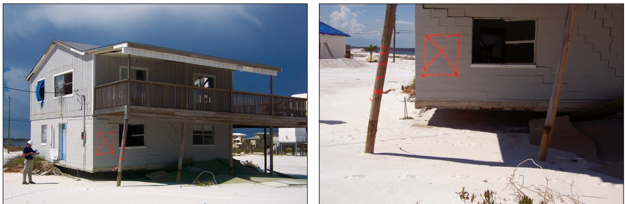
Figure 2-2. Slab-on-grade foundation failure due to erosion and scour undermining and closeup of the foundation failure from Hurricane Dennis, 2005 (Navarre Beach, Florida).
