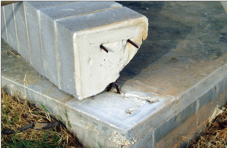
Figure 2-6. Column connection failure (Belle Fontaine Point, Jackson County, Mississippi).
