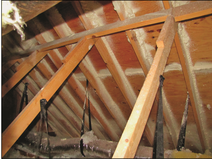
Figure 10: Example of SPF adhesive application to secure and seal roof deck panels
