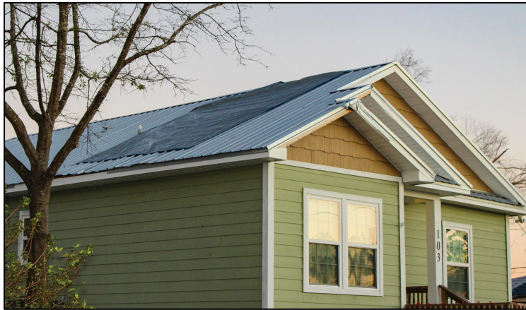
Figure 6: House with a sealed roof deck that successfully prevented the entry of wind-driven rain during Hurricane Michael after windborne debris punctured the metal roof covering.
