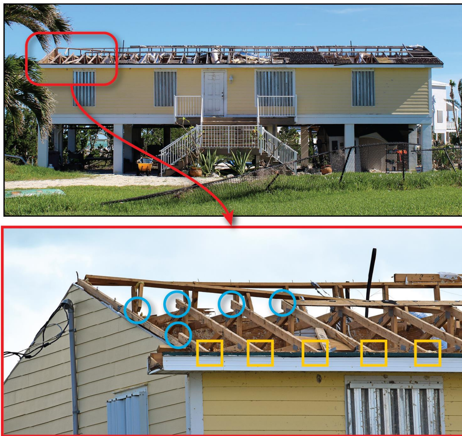
Figure 5: House with structural damage to roof system from Hurricane Irma where the estimated wind speed was 113 mph. This is far less than the design wind speed of 180 mph for the structure at that location. The close-up shows severed truss upper chords (blue circles) and intact connection of lower top chord and top of wall (yellow rectangles).
