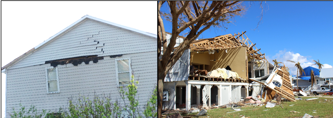
Figure 12: Typical gable end wall failure due to wind loads
