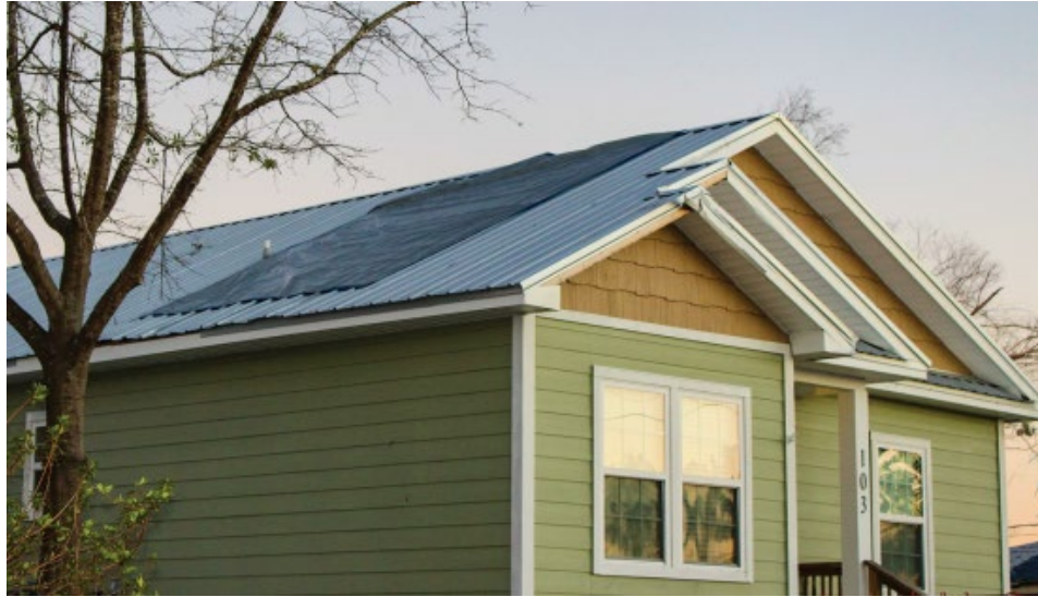
Figure 2: House with a sealed roof deck that successfully prevented the entry of wind-driven rain during Hurricane Michael after windborne debris punctured the metal roof covering.
