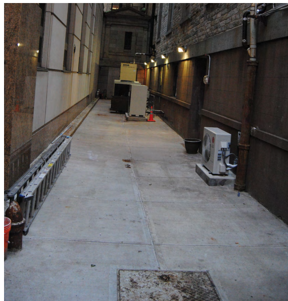
Figure 5-4. Exterior mechanical and electrical equipment
