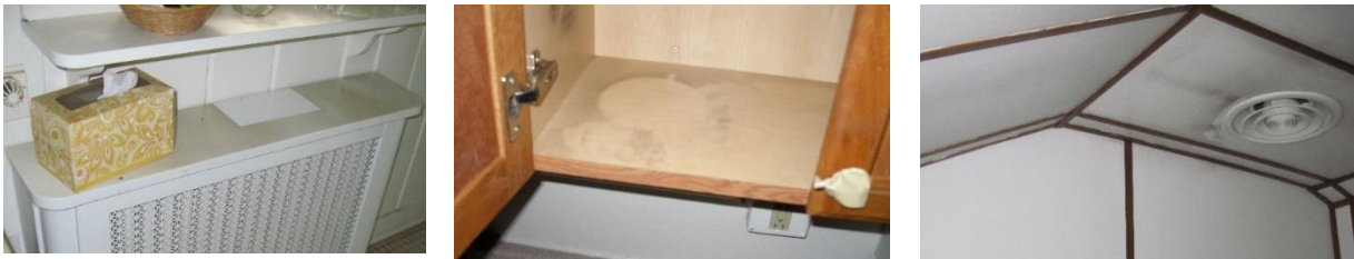
Figure 1. Photos of light soot levels associated with moderate smoke and ash damage. (Photos provided by John DiMenno of Romualdi Davidson & Associates and used with permission.)
