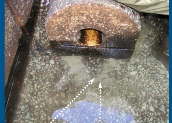
Underdrain outfall in chute block & drain filter deposit.
