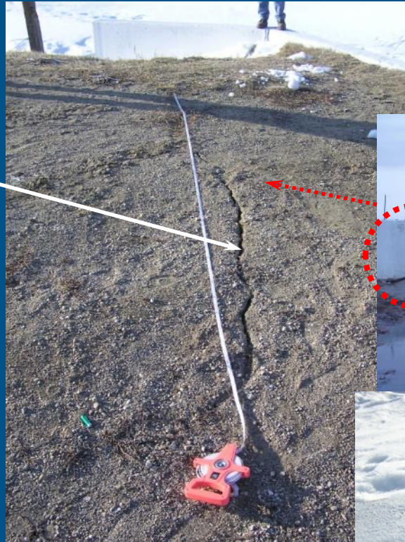
Tension crack in backfill behind spillway wall
