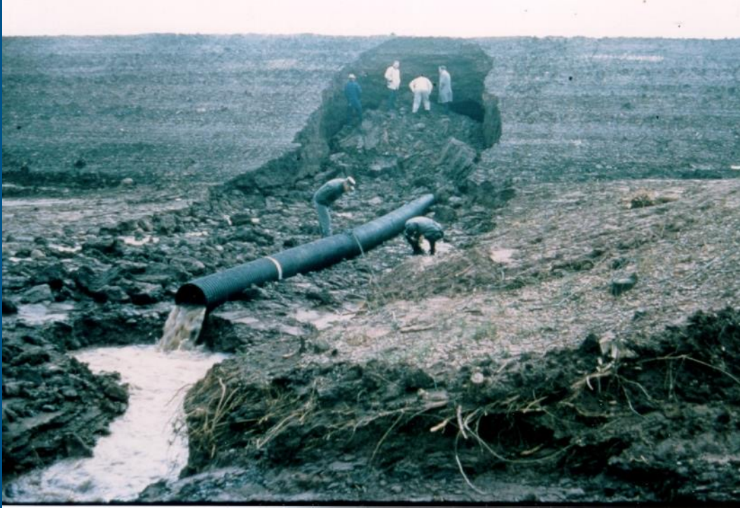
Corrugated metal pipe (CMP) outlet
