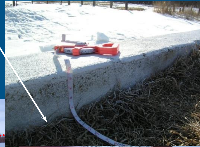
Settlement of backfill adjacent to spillway wall
