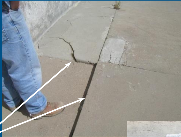
Spalling/cracking of flow surfaces
