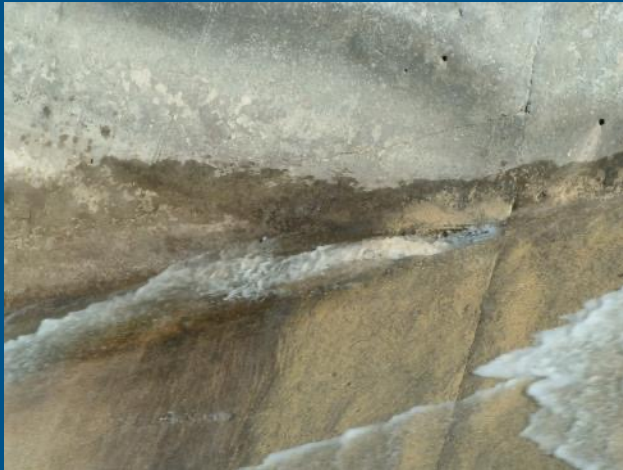
Underdrain discharge transporting sediment (foundation material)
