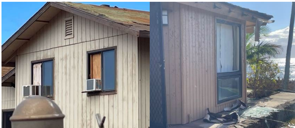
Figure 16. Examples of residential window damages from the Maui wildfires in Lahaina.
