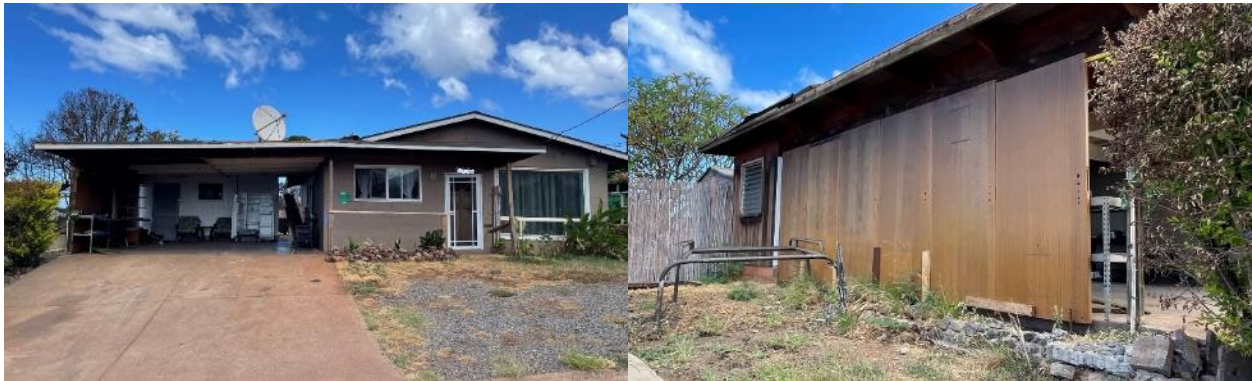
Figure 20. House with attached carport in Lahaina, with carport side support wall constructed or repaired using leftover door panels.
