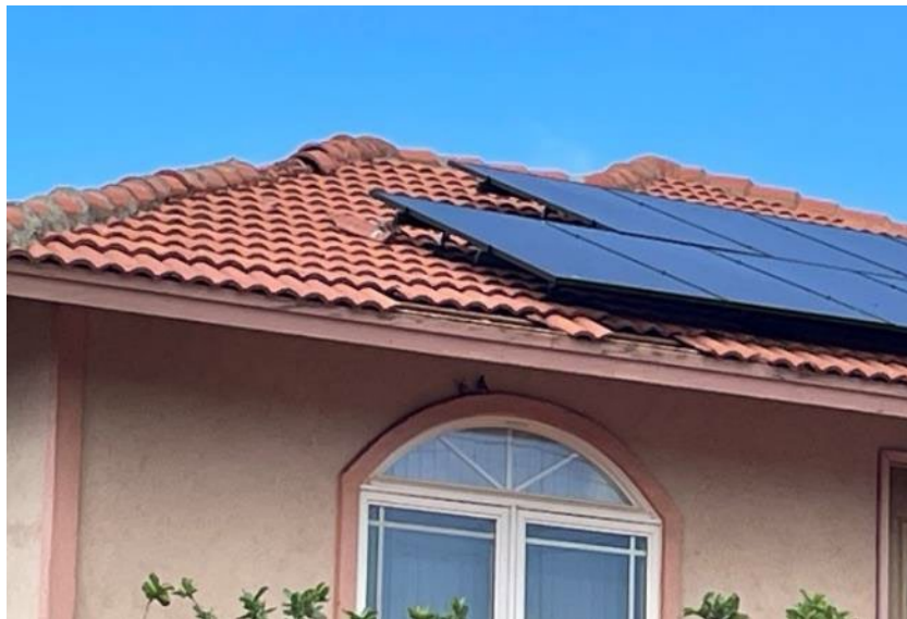
Figure 8. Missing clay roof tiles along roof ridge and edge of residential building in Lahaina.
