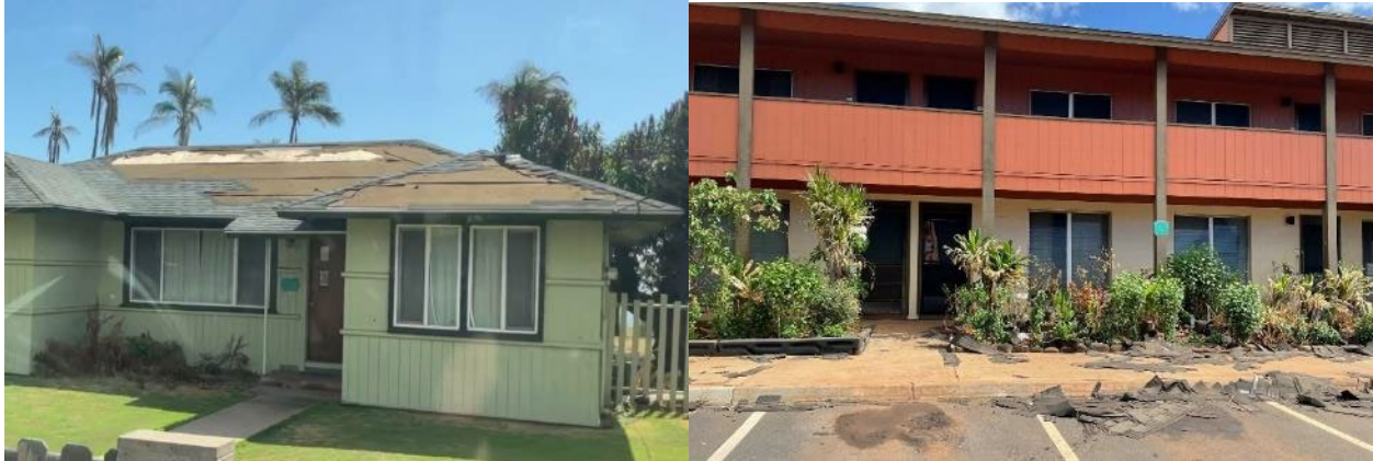
Figure 7. Missing asphalt roof shingles were observed on an intact residential building in Lahaina (left). Asphalt shingles were scattered on the foreground adjacent to an intact multi-family residential building in Lahaina (right).
