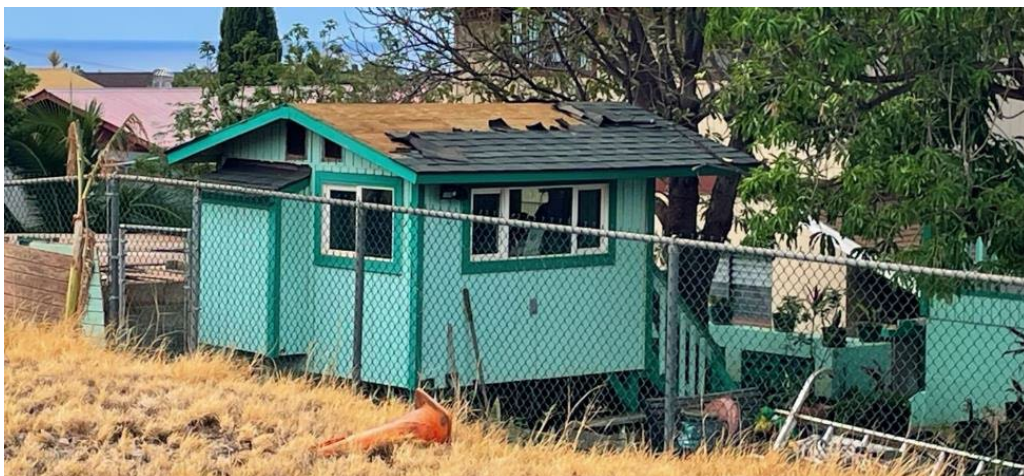
Figure 19. Accessory dwelling unit (‘ohana) behind main residence in Lahaina damaged by high winds during wildfire.
