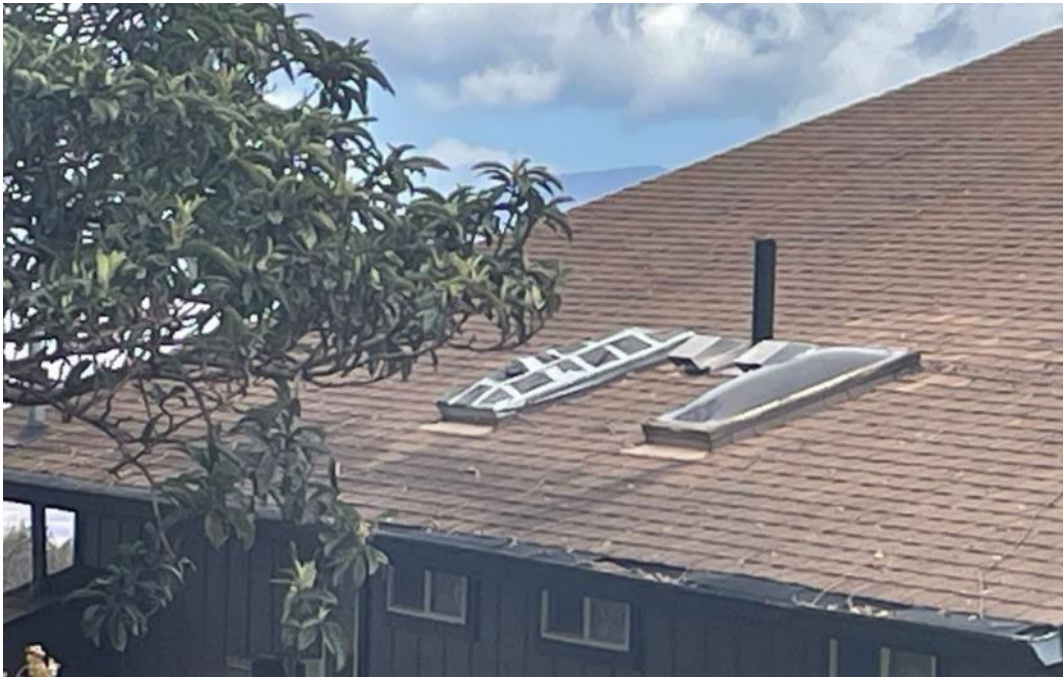
Figure 18. Older plastic skylight on a residential building in Kula damaged by wildfire.
