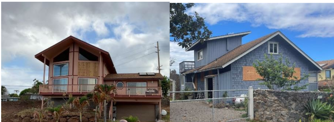
Figure 17. Large broken windows covered by plywood sheathing on residences in Lahaina (left) and Kula (right).
