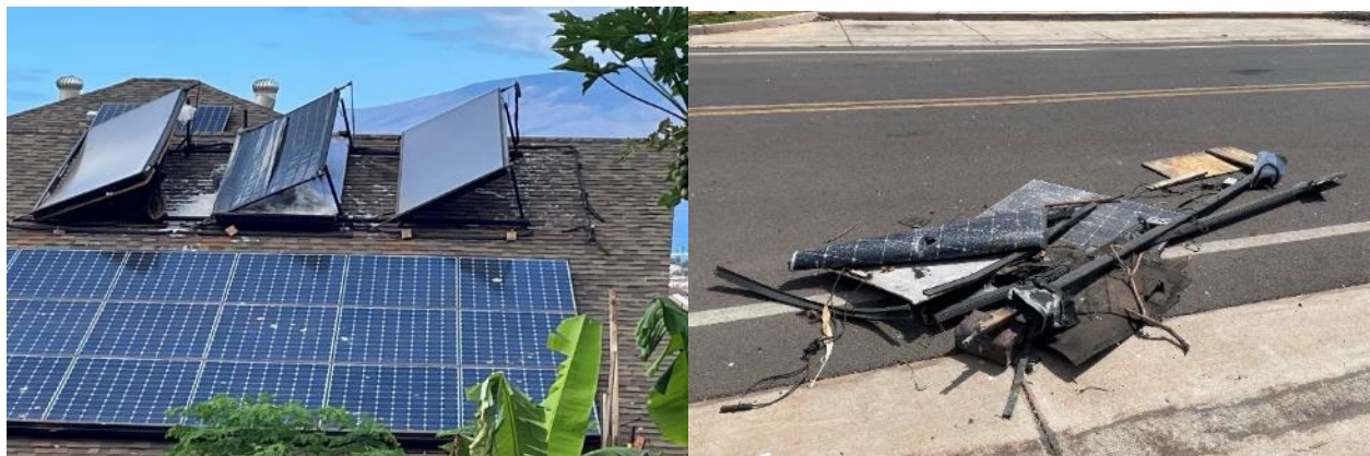
Figure 11. Damaged solar water heaters observed on a residential building in Lahaina (left). PV panels found on the ground along a street lined with single-family residential buildings in Lahaina (right).
