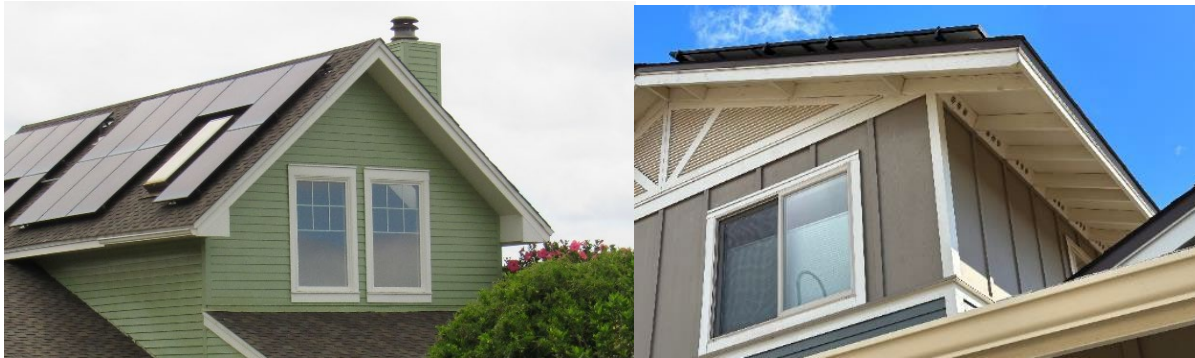
Figure 12. Typical closed Soffit on Maui residential building (left). Open soffits with small “birdhole” vents on residential units in Lahaina created by an extension of roof framing (right).
