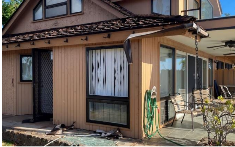
Figure 10. Melted vinyl gutters and melted window frame with lost glass pane on a residential building in Lahaina.
