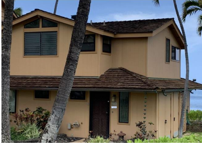
Figure 9. Wood shake roof on a residential building in Lahaina, showing evidence of some surface shakes charred by fire.
