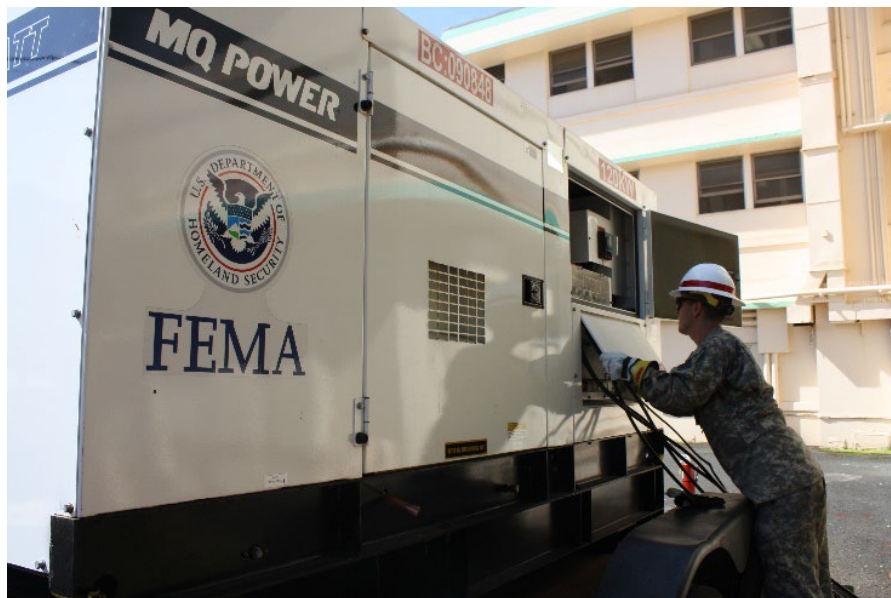
Figure 1. A backup generator is being connected to a building.
