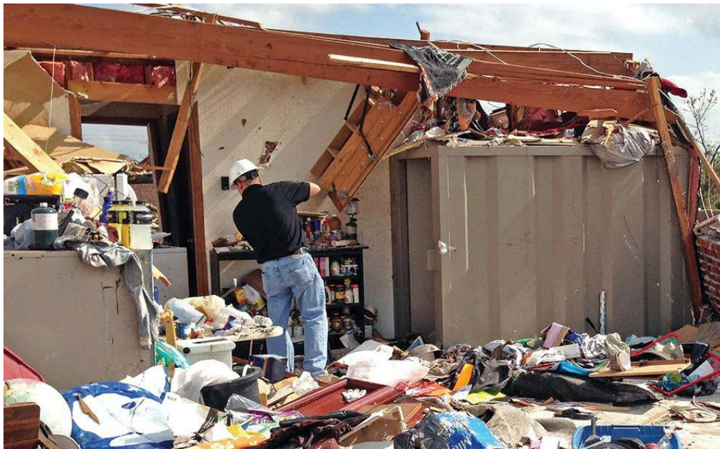
Figure 6. A local building code inspector inspects an above-ground shelter that performed well in a heavily damaged area
