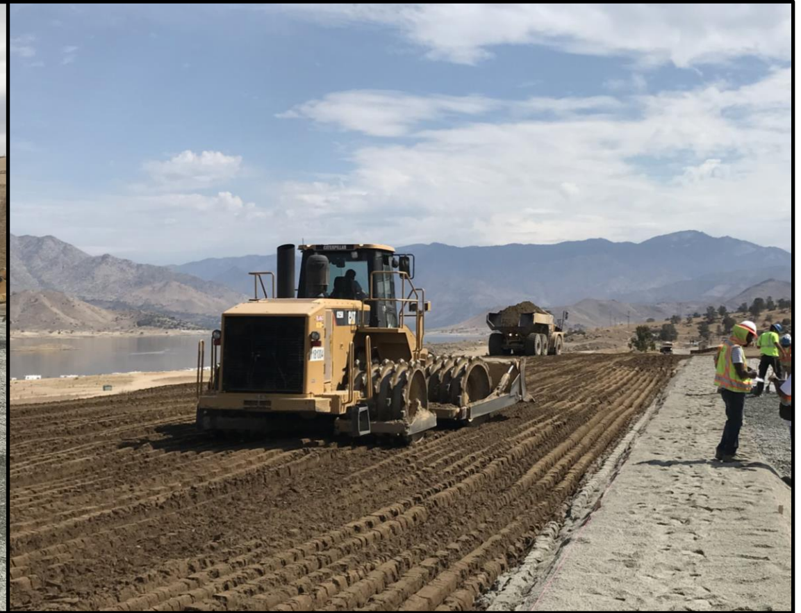
Sheepsfoot Roller for Fine-Grained (Plastic) Materials in Embankment Zones Such as the Dam Core [Thinner Lifts]
