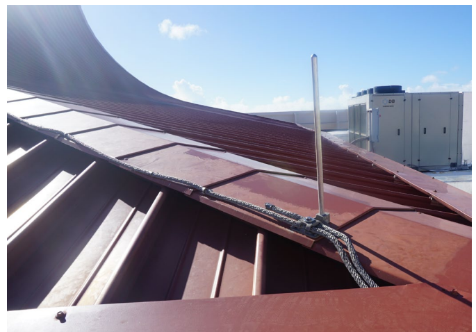
Figure 5. Well-attached lightning protection system at Saipan Airport.
