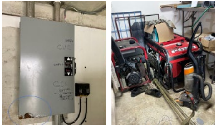
Figure 3. Examples of electrical system damage: corrosion on electrical panel (left) and non-functioning generators (right) see recommendation 3.
