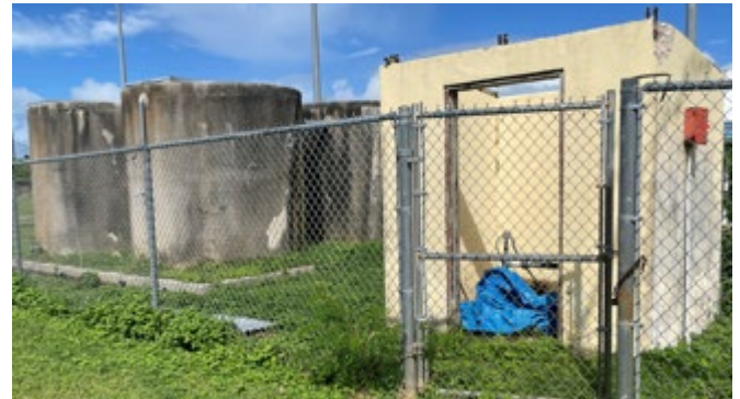
Figure 5. Examples of critical building system damage: water pump enclosure damage and water reservoir in need of maintenance.
