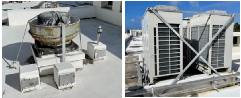
Figure 2. Examples of correctly braced HVAC rooftop units and equipment with little or no damage.
