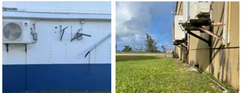
Figure 1. Examples of HVAC damage: blown off mini-split system (left) and corroded wall bracket (right).
