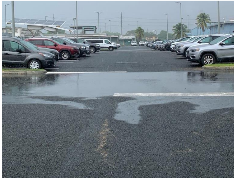
Figure 2-5. Permeable parking lot at the GSA Guaynabo Center after an afternoon rain, showing the water slowly infiltrating into the pavement, recharging the groundwater and reducing runoff at the site. Wet area corresponds to standard pavement placed to sustain more intense traffic, while the remaining parking lot was covered with permeable pavement.
