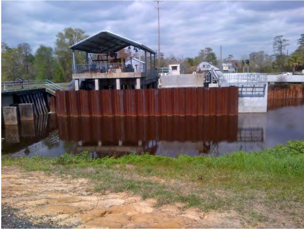
Looking north from the levee at Bayou Patassat, at the sheet pile and bar screen and ramp on the pump station.
