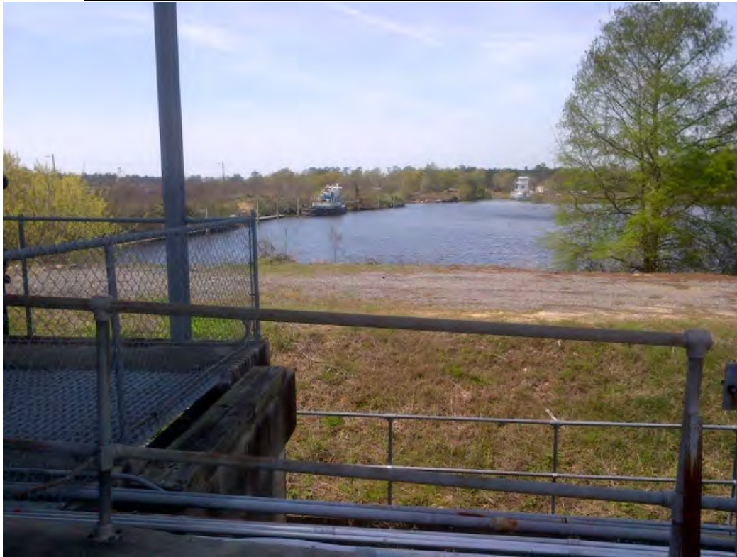
Looking west at Bayou Bonfouca. Note the earthen levee dam between the pump station and Bayou Bonfouca. City of Slidell flows from Bayou Patassat are pumped into Bayou Bonfouca, which flows into Lake Ponchartrain.
