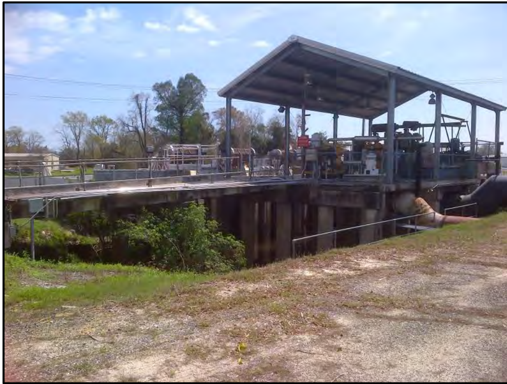
Figure 4. View of outlet pipes from pumping station for City Barn Drainage on Bayou Pattosat through earthen embankment facing southwest.
