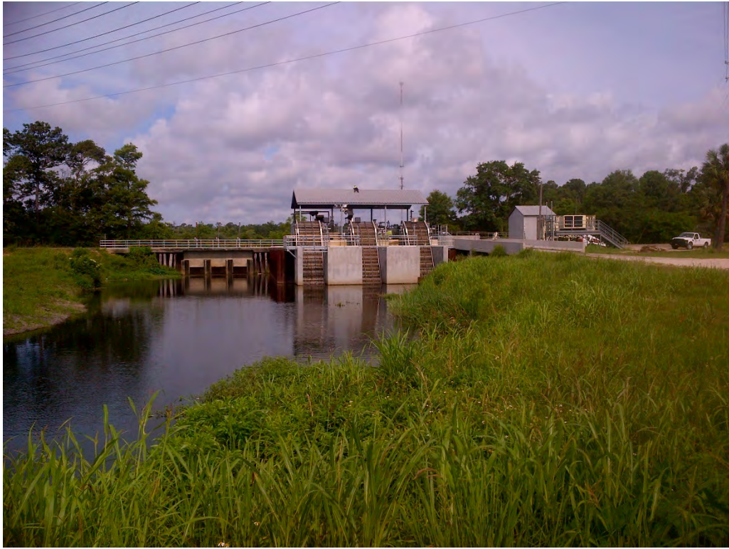
Overview of pumping station area.
