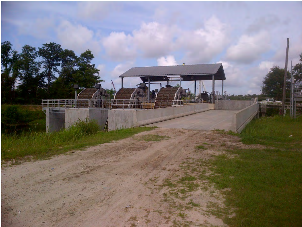
Bar screen mechanism and access ramp with roof covering pumping station in background.
