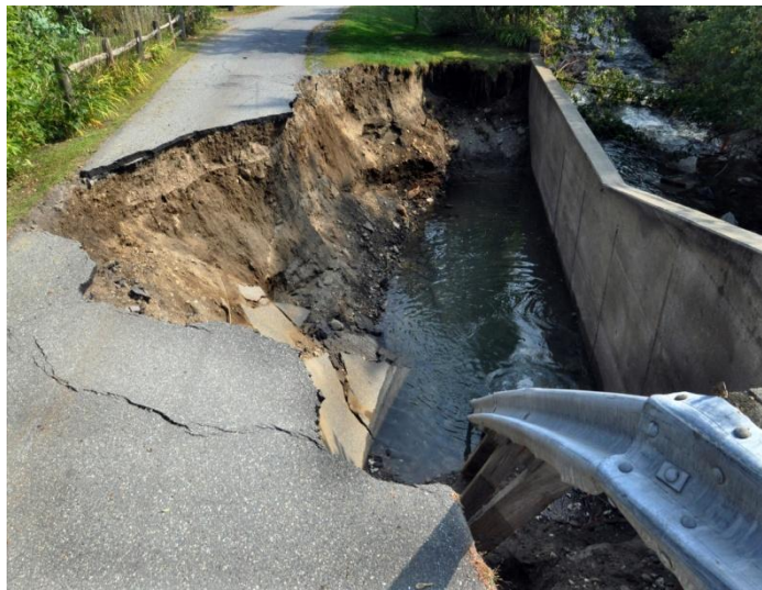
Woodstock, Vt., September 4, 2011 -- Tropical storm Irene caved in many roads after dropping more than 11 inches of rain. This caused floods which destroyed much of Vermont’s infrastructure. Photo by Wendell A. Davis Jr.
