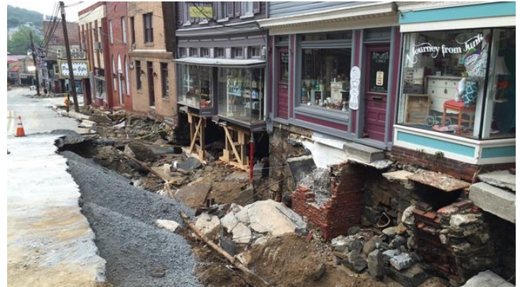
Figure 1. Damage to historic storefronts downtown after the flash flood. Source: FOX5 DC.
