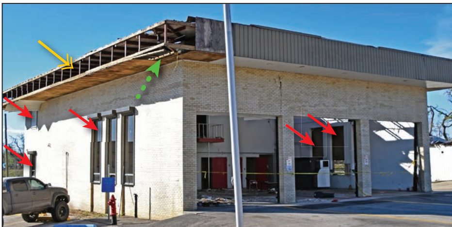
The red arrows indicate the retrofitted storm shutters. Wind-driven rain entered the building at the damaged fascia and soffit (yellow and green arrows).
