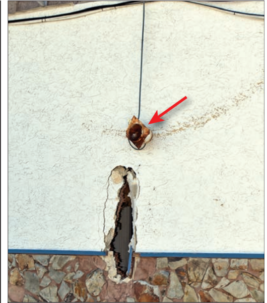
The white portion of the wall was stucco over metal lath over plywood over studs. The debris penetrated the interior gypsum board sheathing. The red arrow indicates a dangling light fixture that fell from the soffit.
