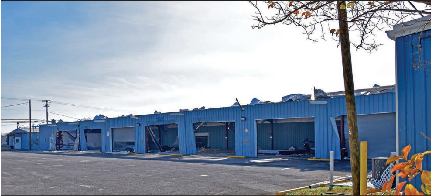
Figure 6: General view of the damaged retrofitted rolling doors and roof panel damage
