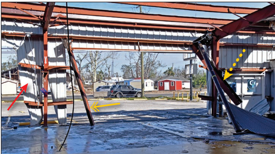
Figure 7: View of door failure caused by inadequate wind resistance of rough opening members
