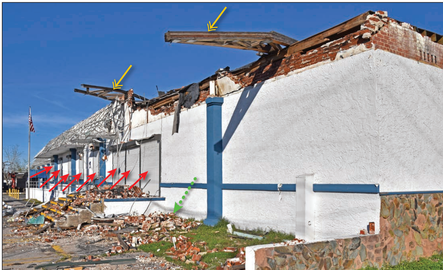
The red arrows indicate the retrofitted storm shutters. Two roof trusses are indicated by the yellow double arrows; the other trusses were blown off the roof. The green dashed arrow indicates collapsed brick.
