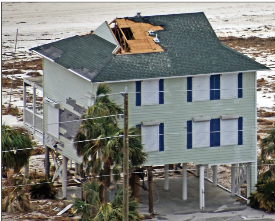
Figure 13: Residence where retrofitted shutters performed well, but significant damage was sustained when rain entered at blown-off roof deck panels (Port St. Joe, FL)
