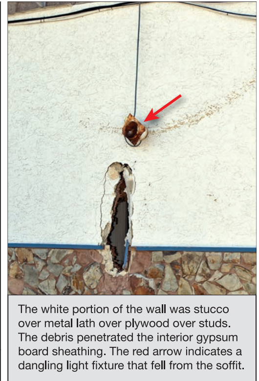
Figure 12: Wall penetrated by wind-borne debris
