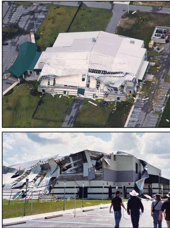
Figure 3. Severely damaged hurricane shelter at Turner Agri-Civic Center, Arcadia, Florida (2004)
