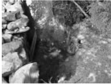
View of breach immediately below masonry wall
