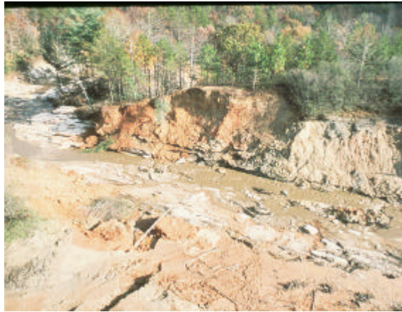
Kelly Barnes Dam Failure Toccoa Georgia
