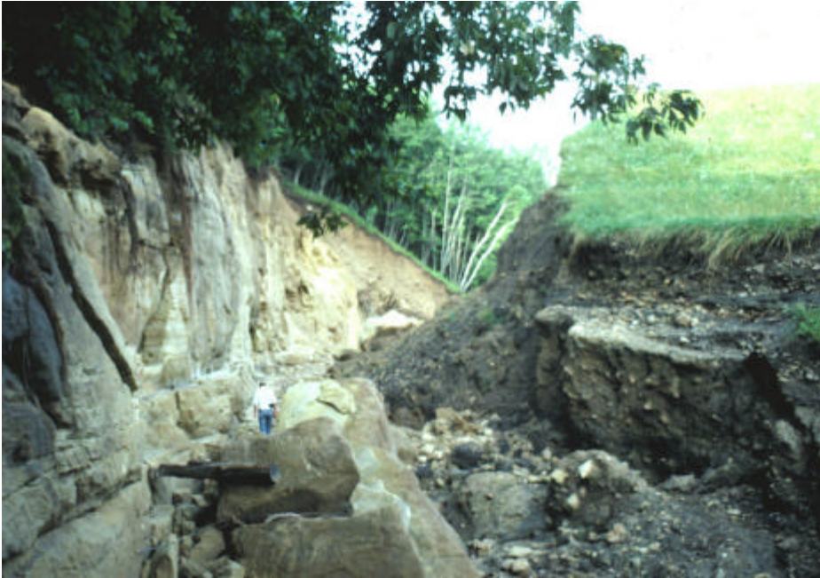
Figure 4 – Coon Creek #41 – note remaining embankment in upper right
