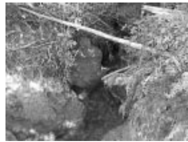
View of breach through earthen embankment
