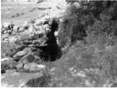
View of breach across crest with masonry wall on upstream face
