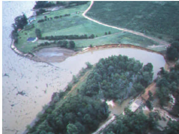
Lake Collins Dam Sumter County Tropical Storm Alberto July 1994
