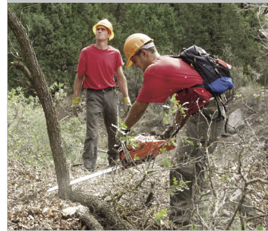
A work crew from Fire Ready, a local fire mitigation company, was hired by the railroad to clear brush and cut trees along the right of way
