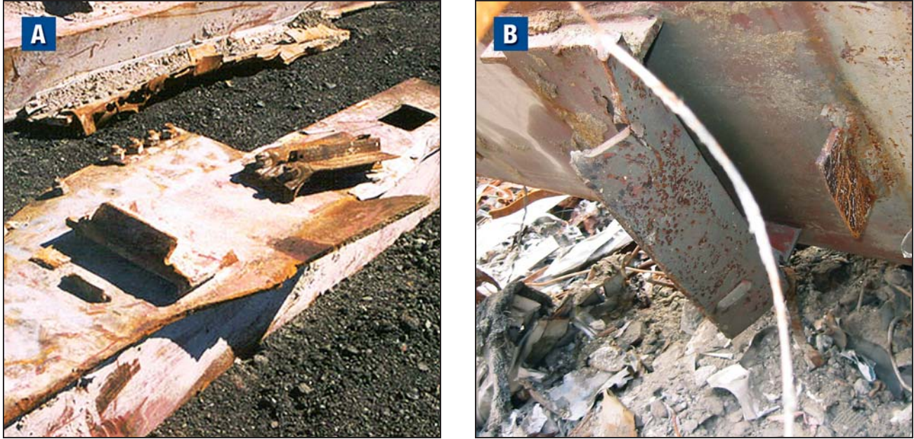
Figure B-9 (A) Visco-elastic damper angles bolted to angle welded to spandrel plate and (B) failed bearing seat connection.
