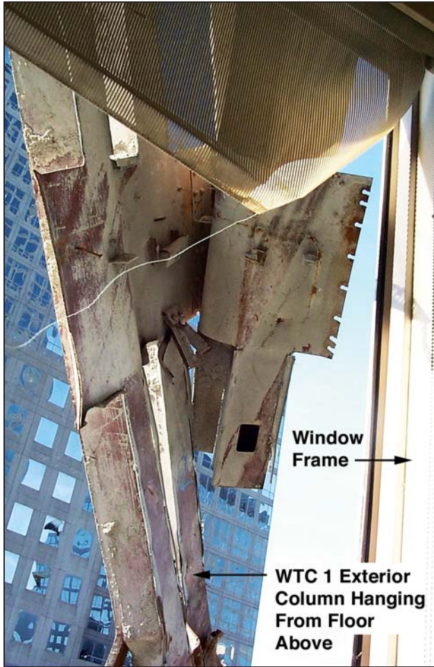
Figure B-5 Column tree showing bolt bearing shear failures of spandrel connection.
