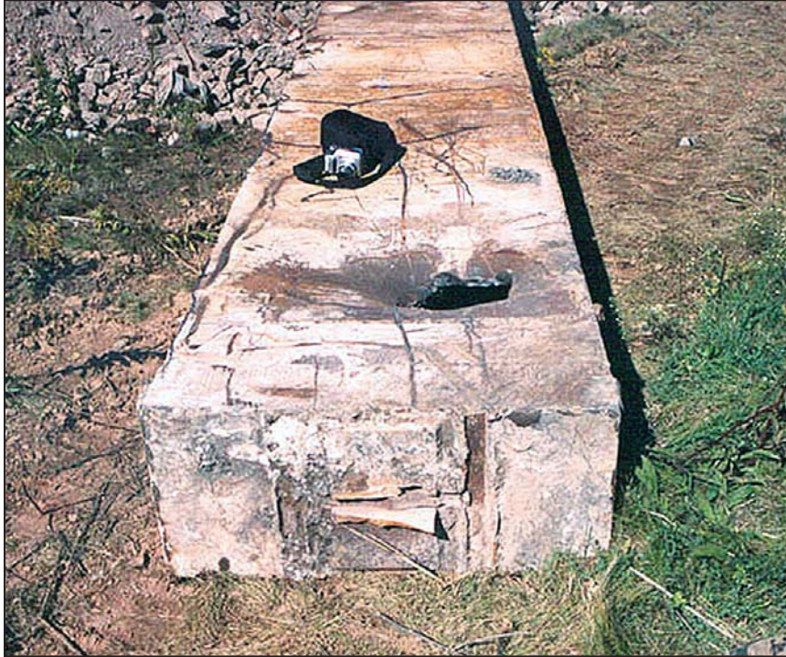
Figure B-6 Shear fracture failure of fillet welds connecting a W-shape column to a box core column.
