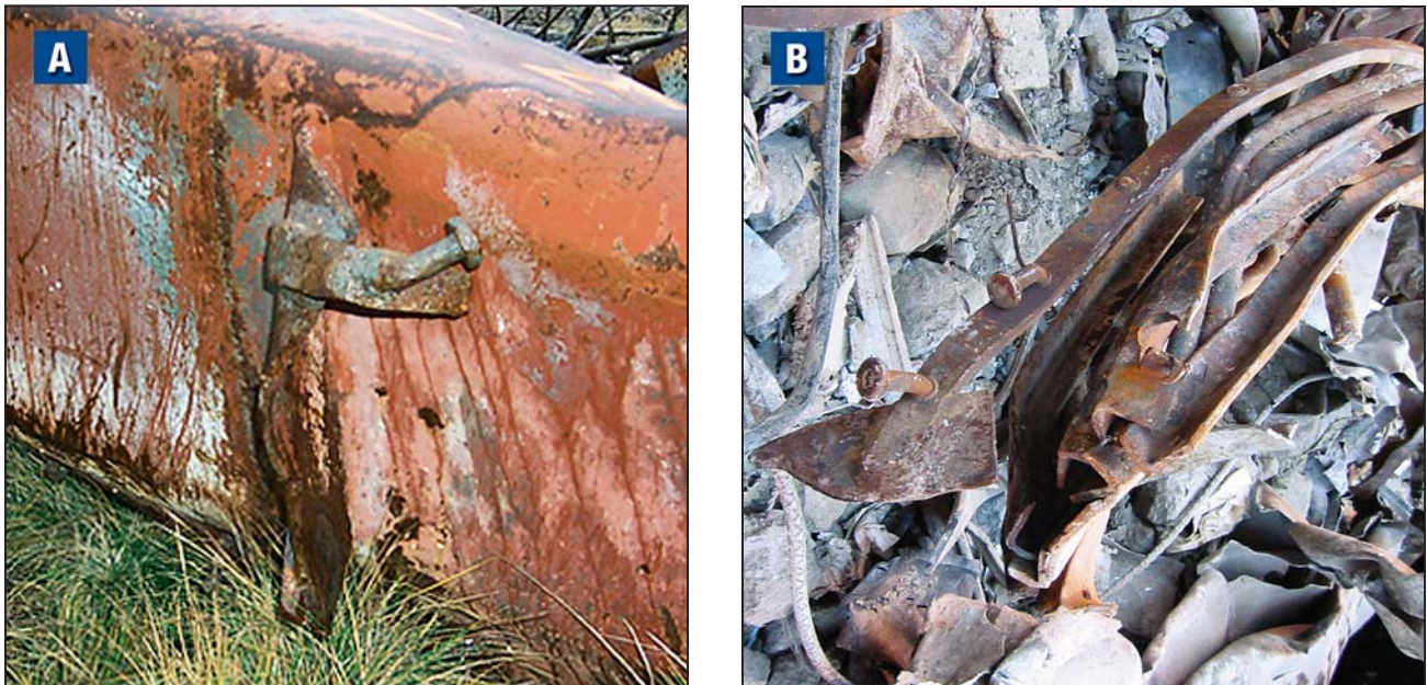
Figure B-10 (A) Bracket plate welded to the column/spandrel plate and (B) horizontal plate brace with shear connectors welded to the failed bracket.
