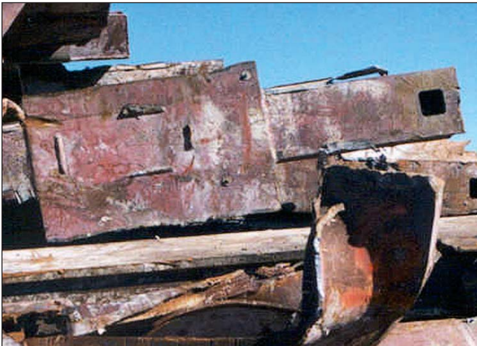
Figure B-11 Shear failure of floor truss connections from column/spandrel plate.
