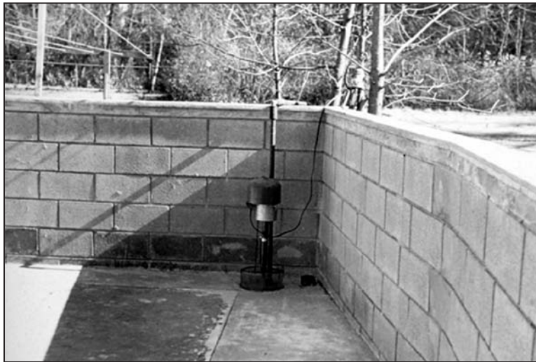
Figure 6-54. Interior sump pump for a residential floodwall
