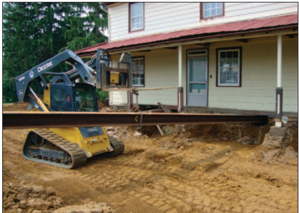
Figure 5R-6. Beams supported by cribbing are placed at critical lift points (photo courtesy of Wolfe House Movers)
