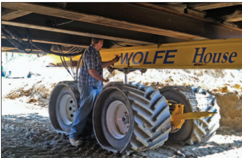
Figure 5R-11. Trailer wheel sets are placed beneath the lifting beams (photo courtesy of Wolfe House Movers)
