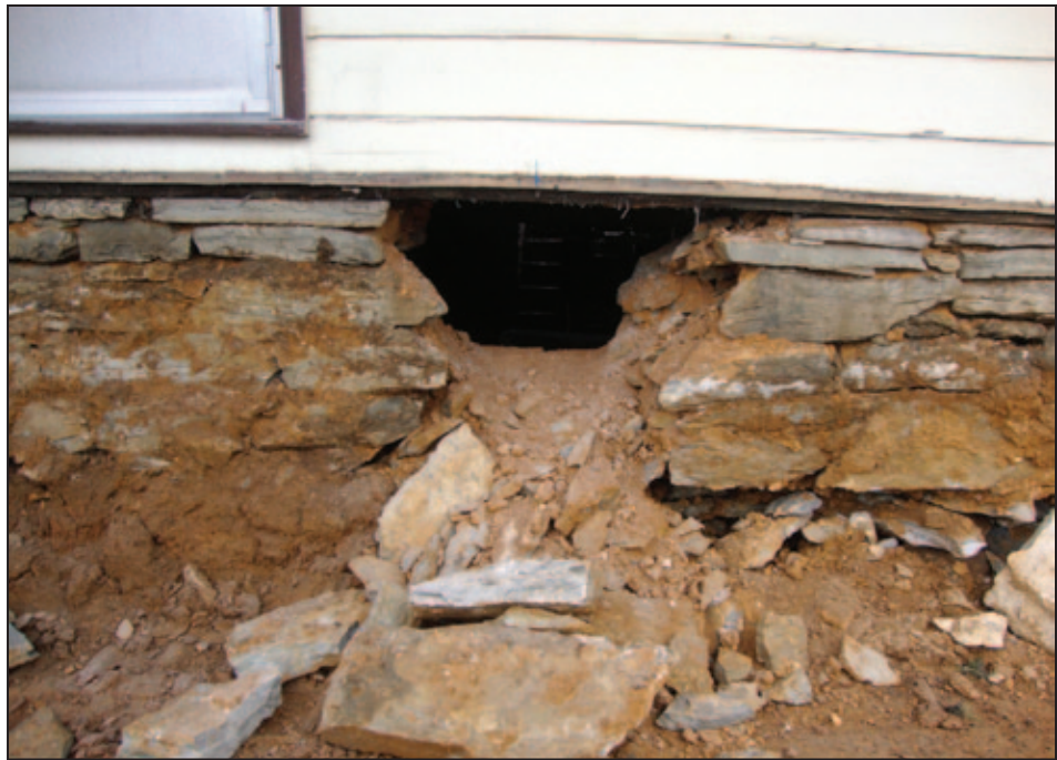
Figure 5R-4. Clearing pathways beneath the structure for lifting supports (photo courtesy of Wolfe House Movers)
