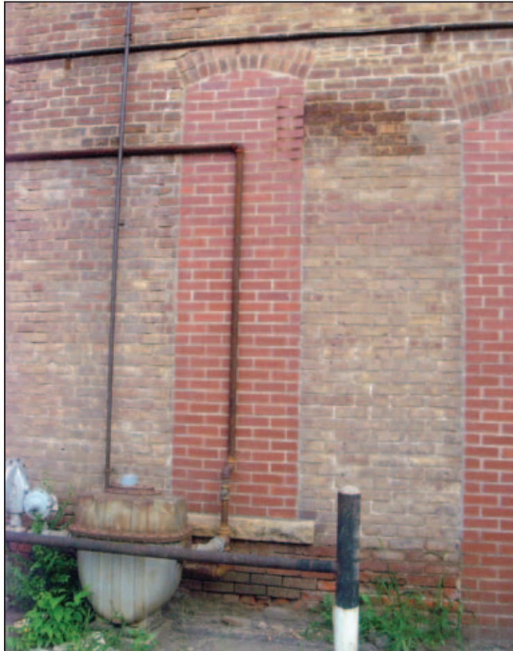
Figure 5D-37. Permanent closure of an opening to prevent floodwaters from entering the building
