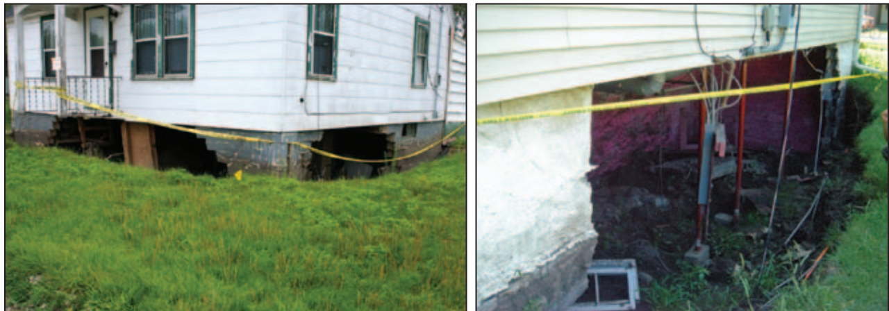
Figure 5D-14. This house’s foundation walls were not able to withstand the forces applied during or after the flood. Rebar would need to be added to help with reinforcement of the CMU foundation.
