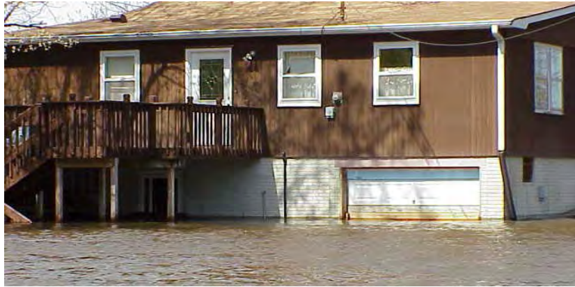
This house was properly elevated when built. Some time after the permit was issued, the owner improved the lower area and subsequently suffered flood damage. This shows the benefit of requiring lower areas to stay open.
