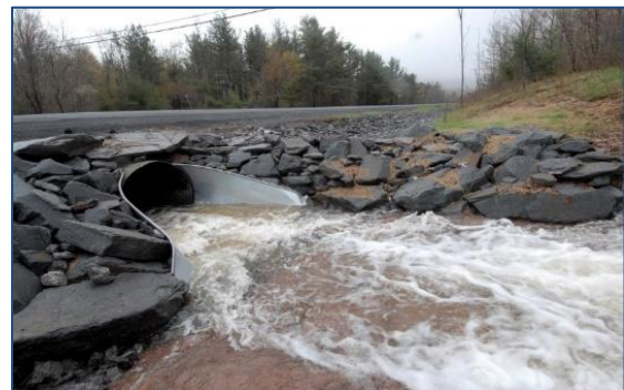
Enlarged culvert and added inlet walls to focus water flow away from roadway.
