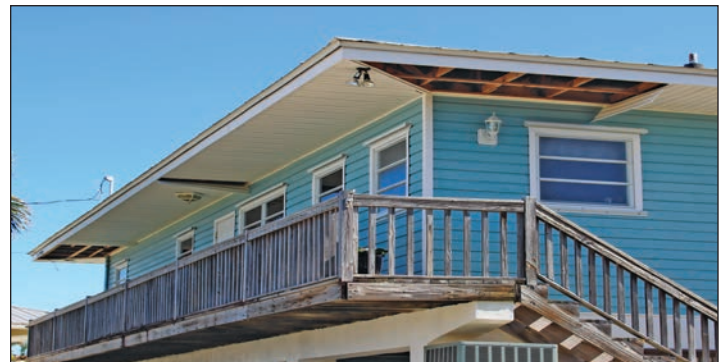
Figure 1: Vinyl soffit damage on a home in Sugarloaf Key
