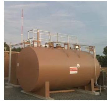
Fig 2 6,000 Gallon, Double-Walled Fuel Tank
