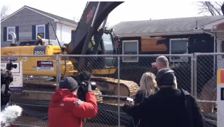
The Kuczynski family watches as their home is being demolished in Sayreville, New Jersey.
