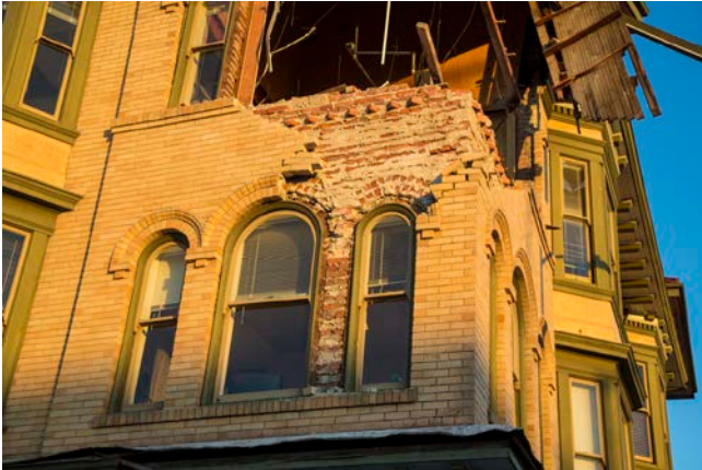
August 26, 2014, Napa, California. At least 103 structures were tagged "RED" by inspectors as unsafe to enter after the earthquake. Photo by Christopher Mardorf/FEMA
