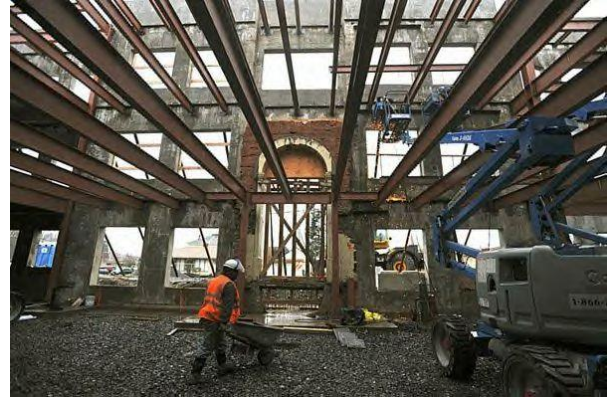
Whatcom Middle School in Bellingham, Washington, reopened in September 2011 after undergoing a seismic retrofit. ©2011 The Bellingham Herald.
