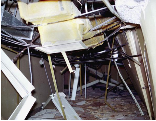
Non-structural damage to the basement of the Olive View Medical Treatment Building caused by the 1971 San Fernando earthquake. ©1971 by Earthquake Engineering Research Center and Regents of the University of California.
