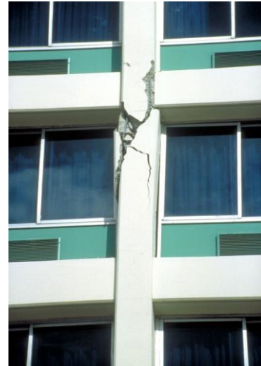
Damage to older, reinforced concrete building in the 1994 Northridge Earthquake. ©1994 by Peter W. Clark and Regents of the University of California.
