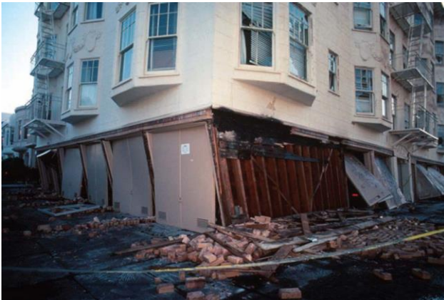
First story of an apartment building in San Francisco, California, leaning to the side after the 1989 Loma Prieta earthquake. U.S. Geological Survey Image.
