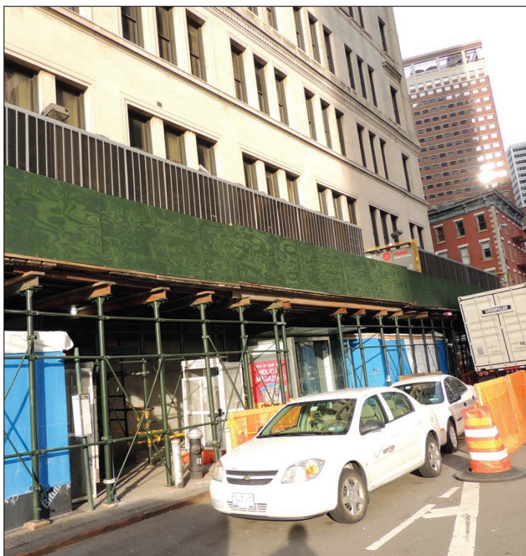
Figure 4: Temporary chillers elevated on scaffolding during repair of a high-rise building in lower Manhattan
