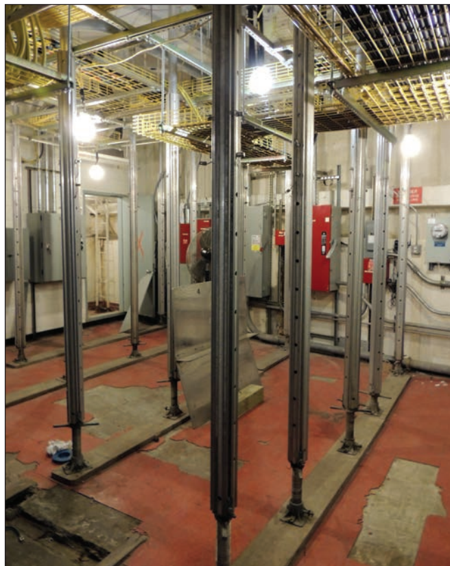
Figure 1: Temporary structural support system for electrical and mechanical room equipment being elevated from subgrade to a higher floor in a high-rise building in lower Manhattan. The temporary columns will eventually be replaced with a permanent support system.
