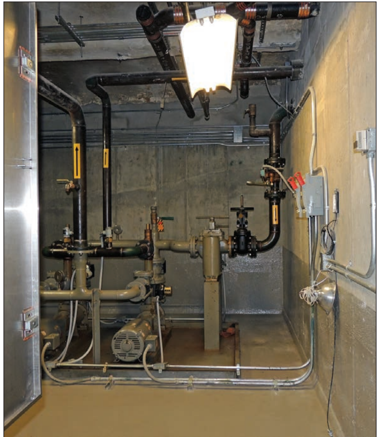
Figure 3: Dry floodproofed fuel pump room adjacent to generator fuel tank vault in lower Manhattan
