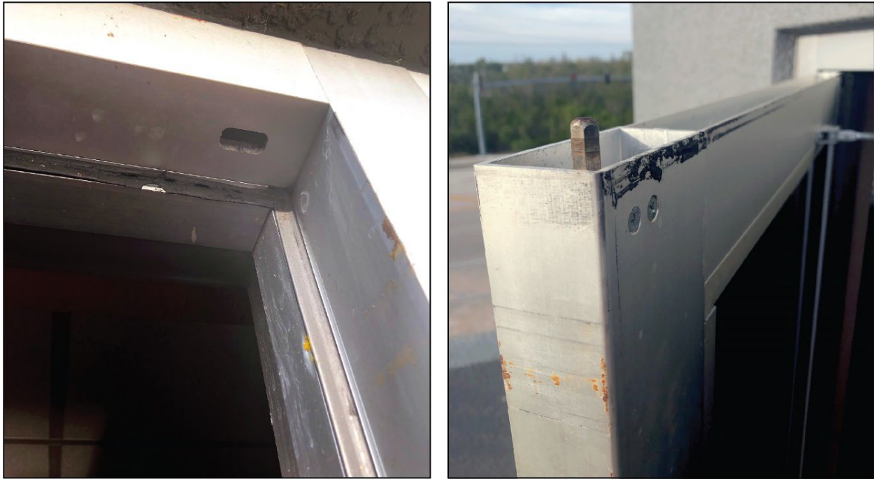
Figure 5-62: Receiving slot (left) is significantly larger than latching mechanism (right) (Lee County)
