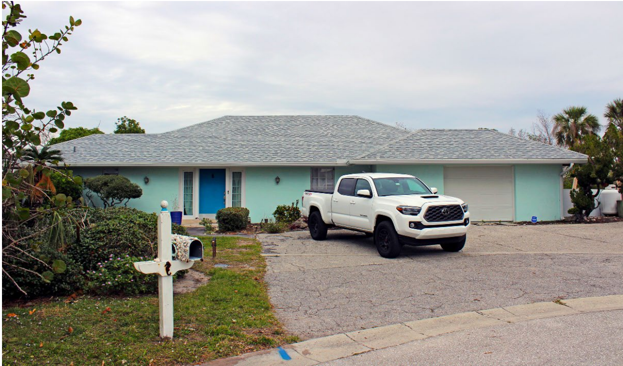
Figure 4-12: A house with an asphalt shingle roof that was replaced in December 2020, with no damage (EWS = 128 mph; DWS = 155 mph) (Placida)
