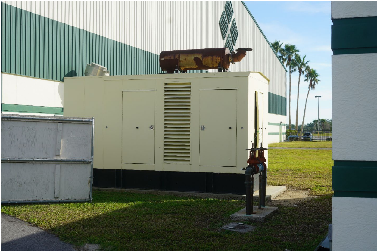
Figure 5-25: Generator at the Turner Center that failed during Hurricane Ian (DeSoto County)
