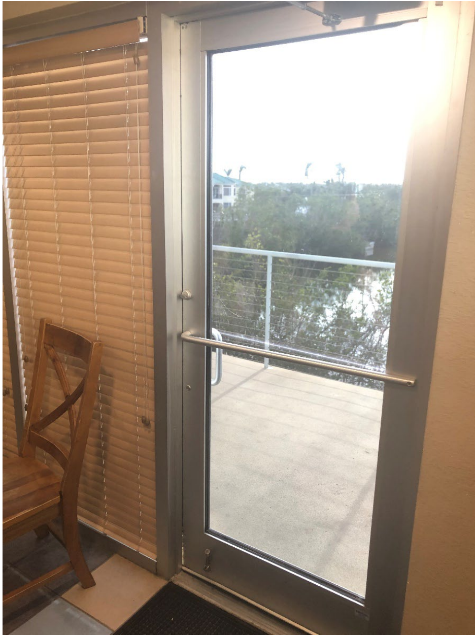
Figure 5-61: Door from dining area to balcony that blew open during Hurricane Ian (Lee County)
