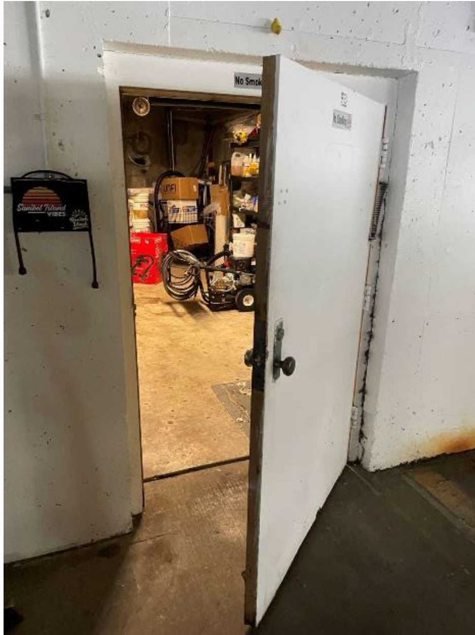
Figure 3-93: Ground level storage room was not floodproofed and sustained flood damage (Lee County, Zone AE)
