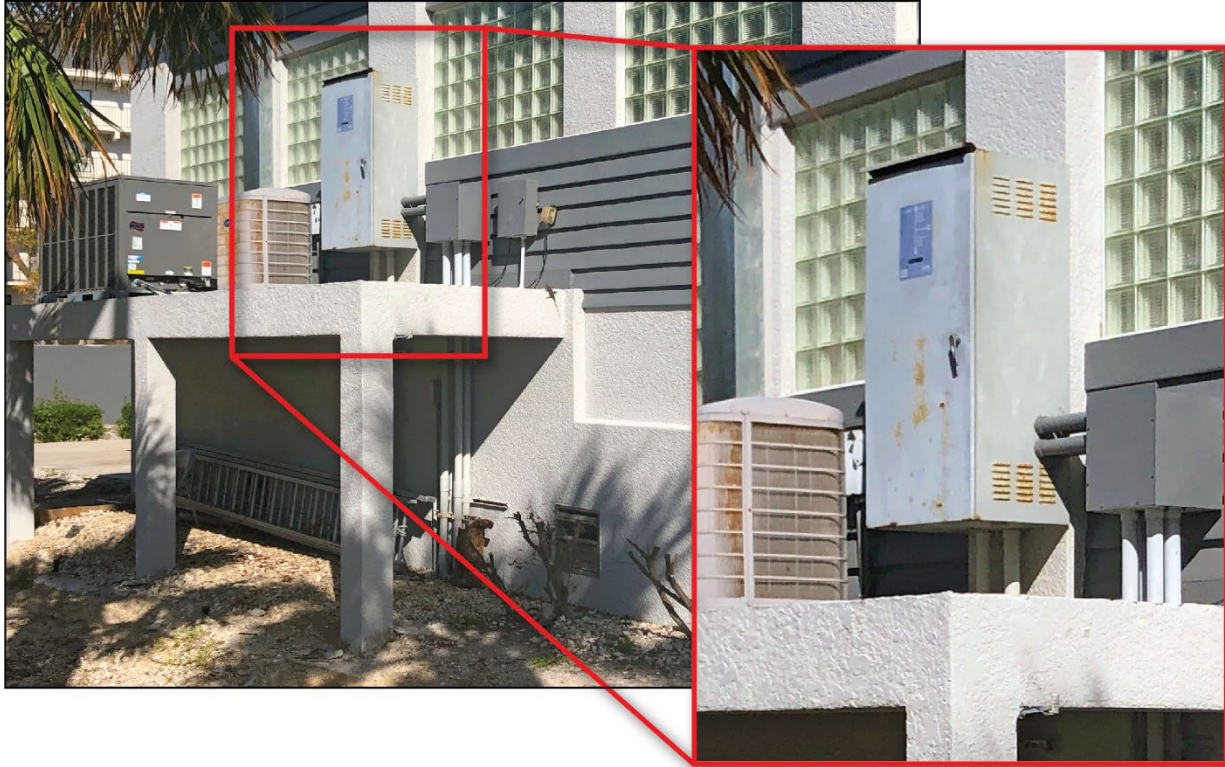
Figure 5-58: ATS damaged during Hurricane Ian (Lee County)
