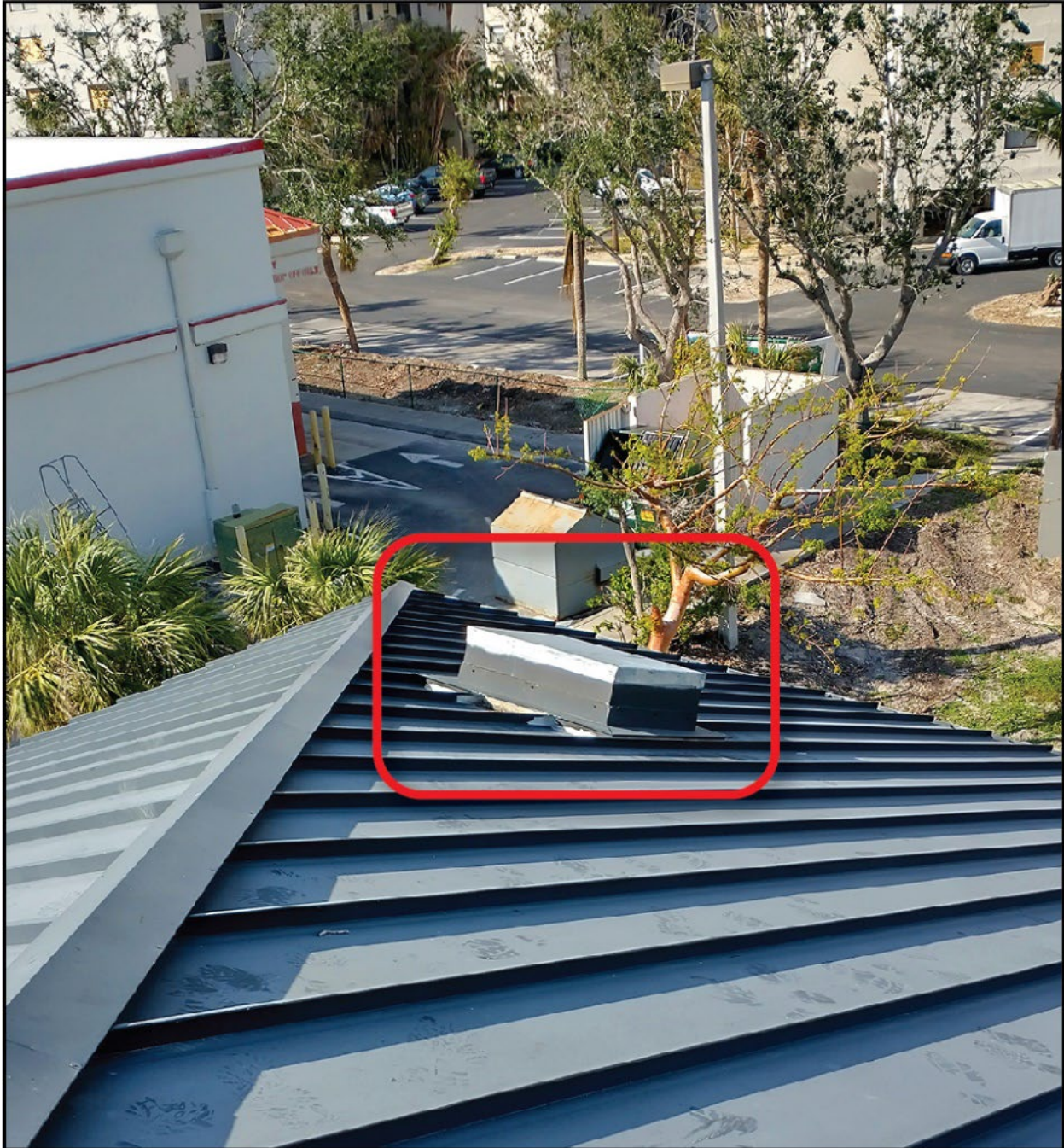
Figure 5-57: Roof-mounted exhaust fan lost during Hurricane Ian (Lee County)
