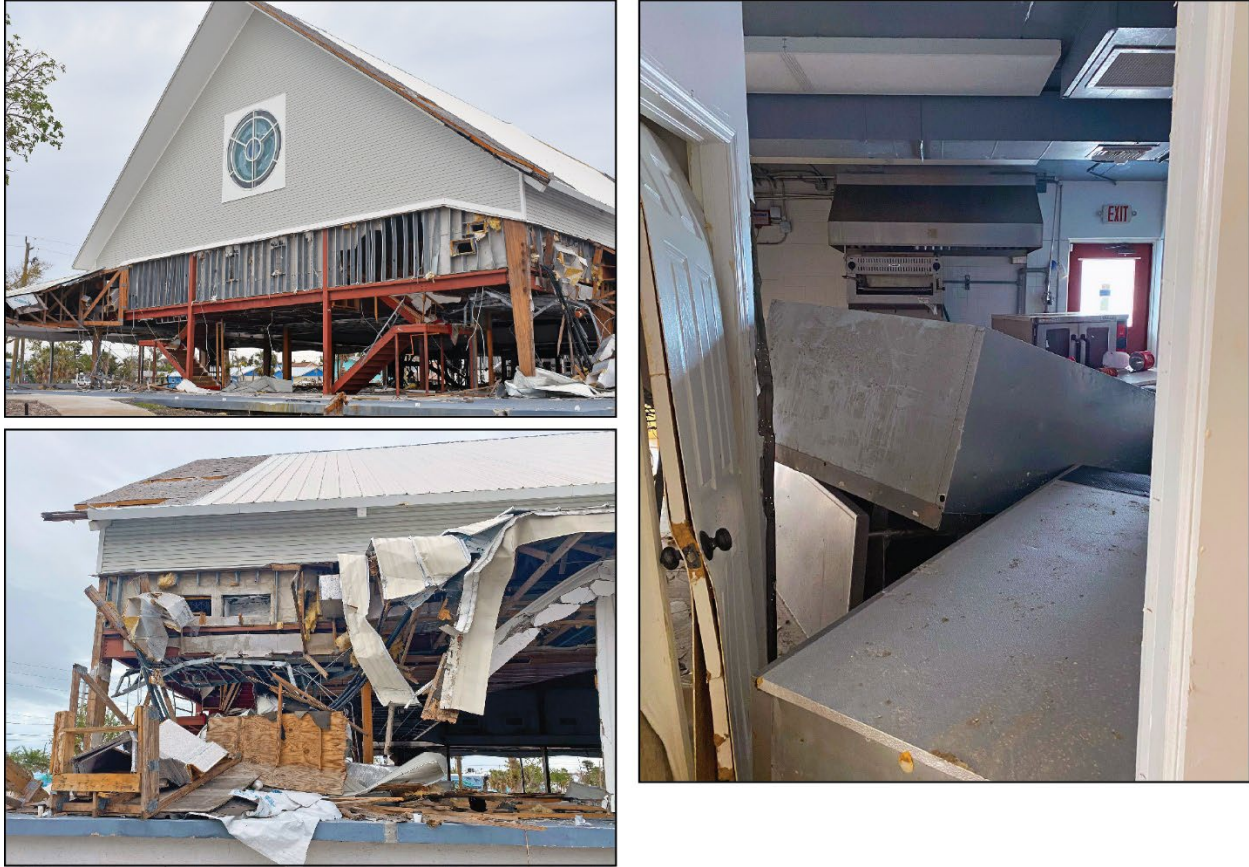
Figure 3-99: Examples of observed damage at Chapel by the Sea
