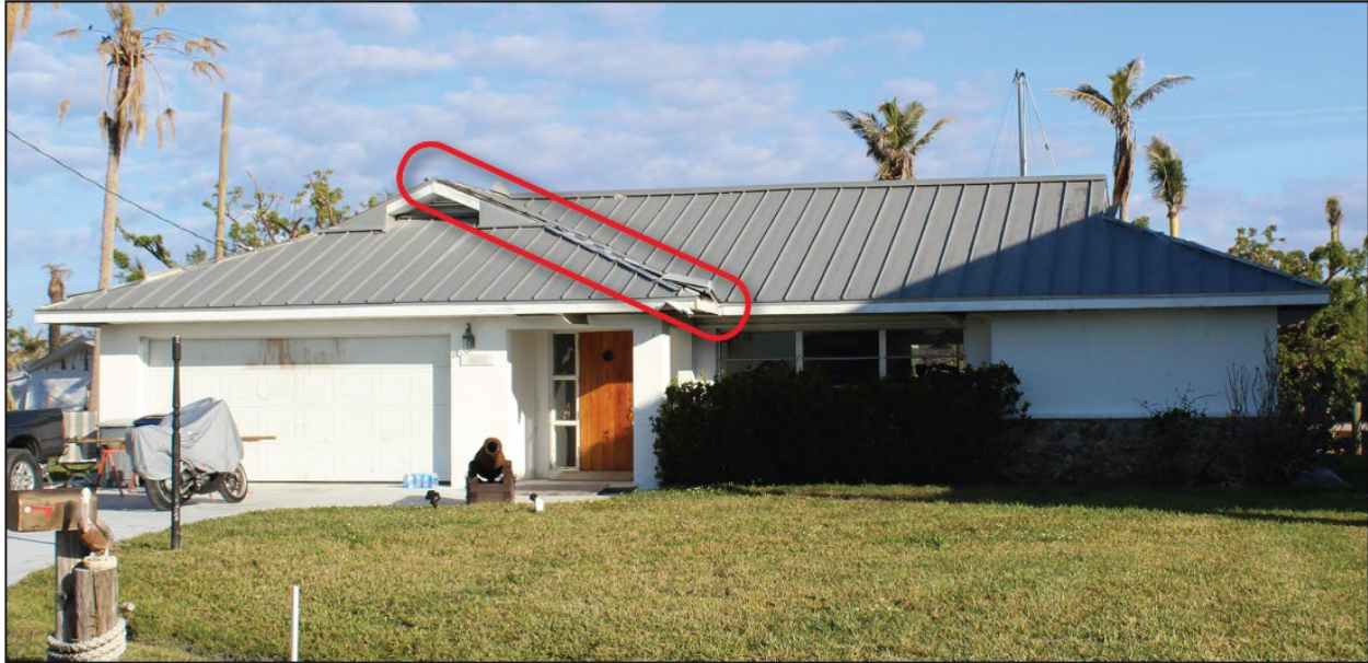
Figure 4-25: Typical hip cover damage on a metal panel roof (EWS: 115 mph; DWS: 161 mph) (St. James City)
