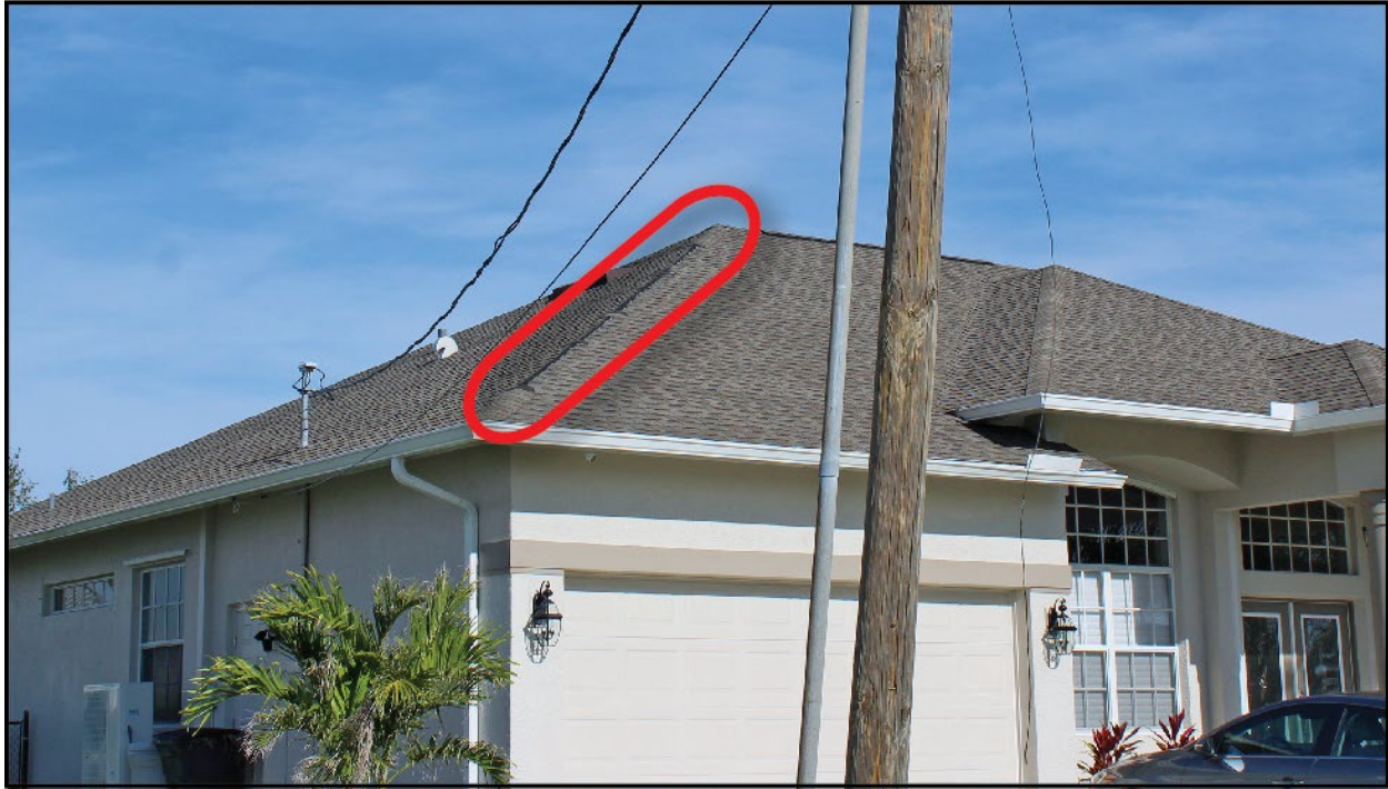
Figure 4-45: A house built in 2002 with an asphalt shingle roof replacement in 2019, with minor hip shingle damage, a “storm-related” roof replacement permit was issued post-Hurricane Ian (EWS = 128 mph) (Port Charlotte)
