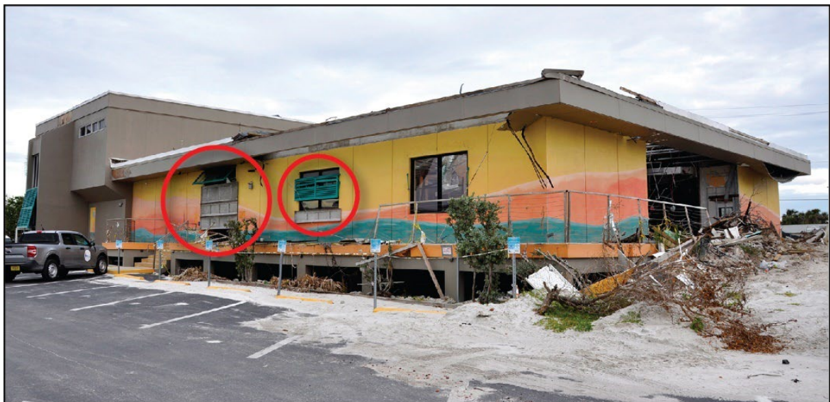
Figure 3-78: Dry floodproofing measures implemented (barriers circled) at Fort Myers Beach Town Hall (Lee County, Zone AE)
