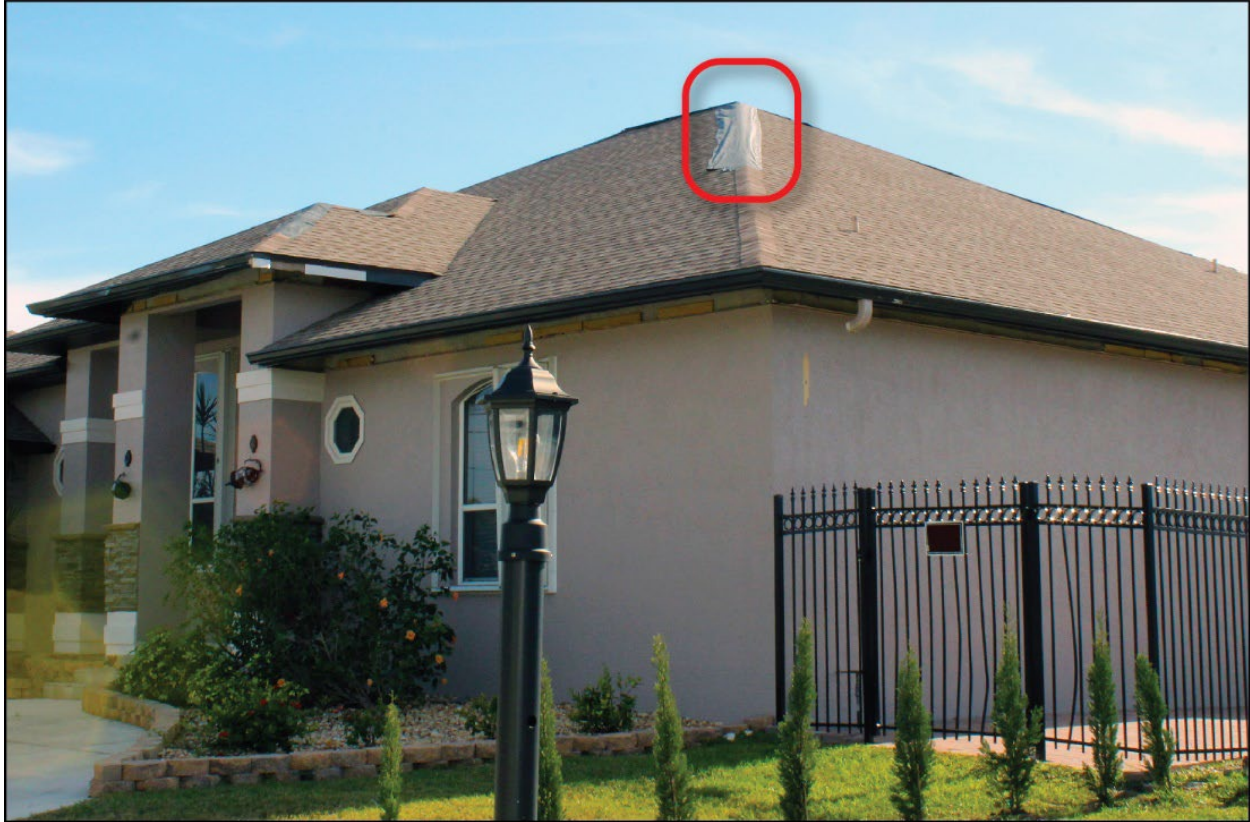
Figure 4-37: A house with asphalt shingle roof; built 1998 and reroofed August 2020 (minor hip shingle damage) (EWS = 128 mph) (Port Charlotte)
