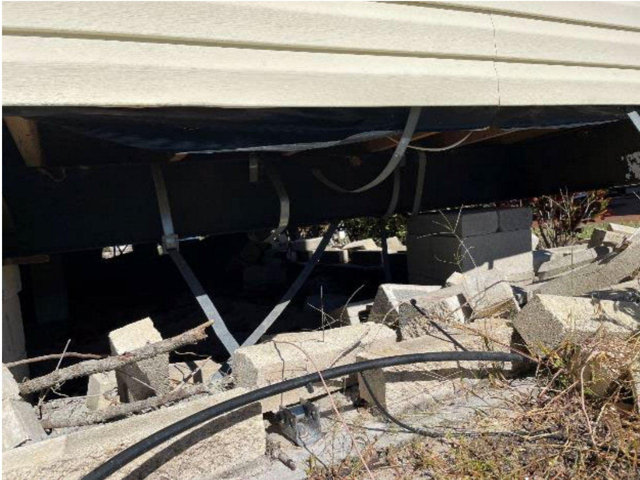
Figure 3-117: Damaged tie downs, unreinforced masonry piers, and skirting below a manufactured home in Old Bridge Village (Lee County, Zone AE)
