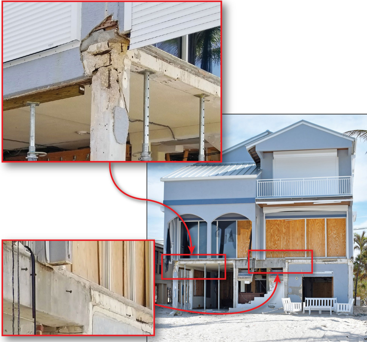
Bottom right: Post-event photo from January 2023. Top left: Corner column damage. Bottom left: Remaining anchors in the main structure.
