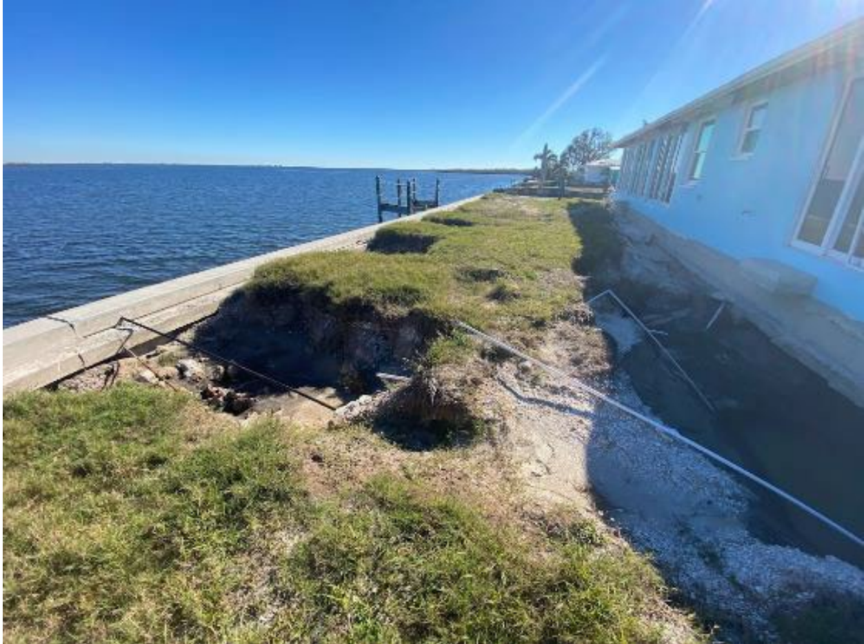
Figure 3-36: Example of exposed, newly installed, tie-back rods in Matlacha Isles (Lee County, Zone VE)
