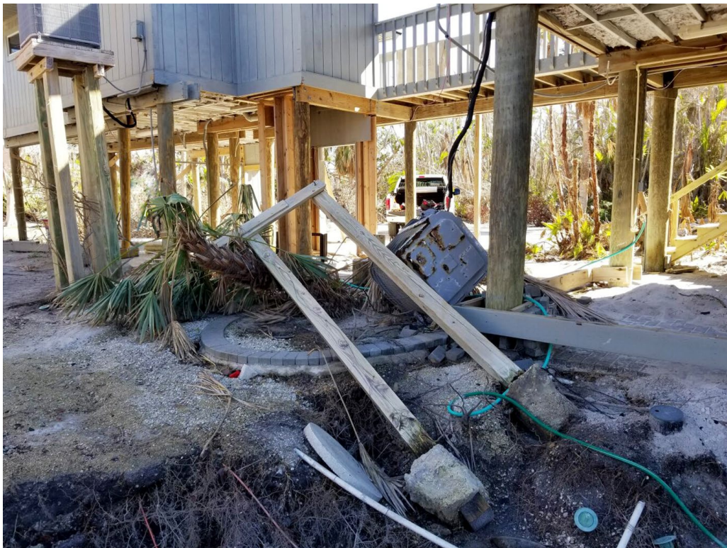
Figure 3-24: Scour resulting in the collapse of a platform supporting an air conditioning unit
