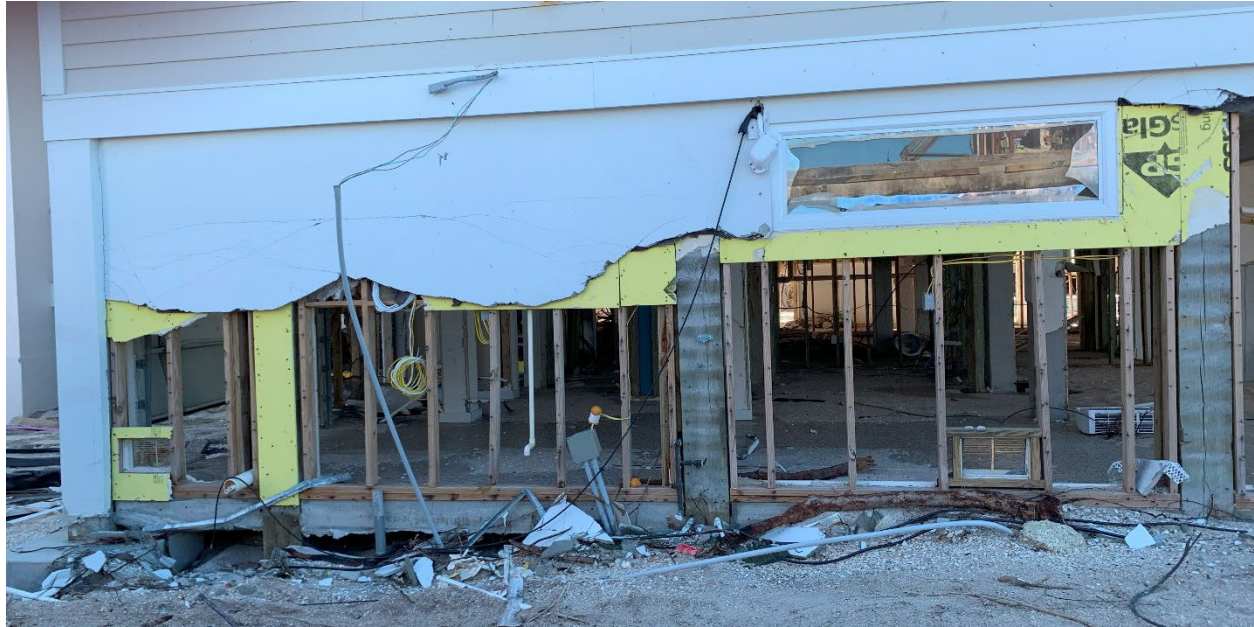
Figure 3-15: Partial failure of shore-perpendicular breakaway wall on Sanibel Island (Lee County, Zone VE, Seaward of CCCL)
