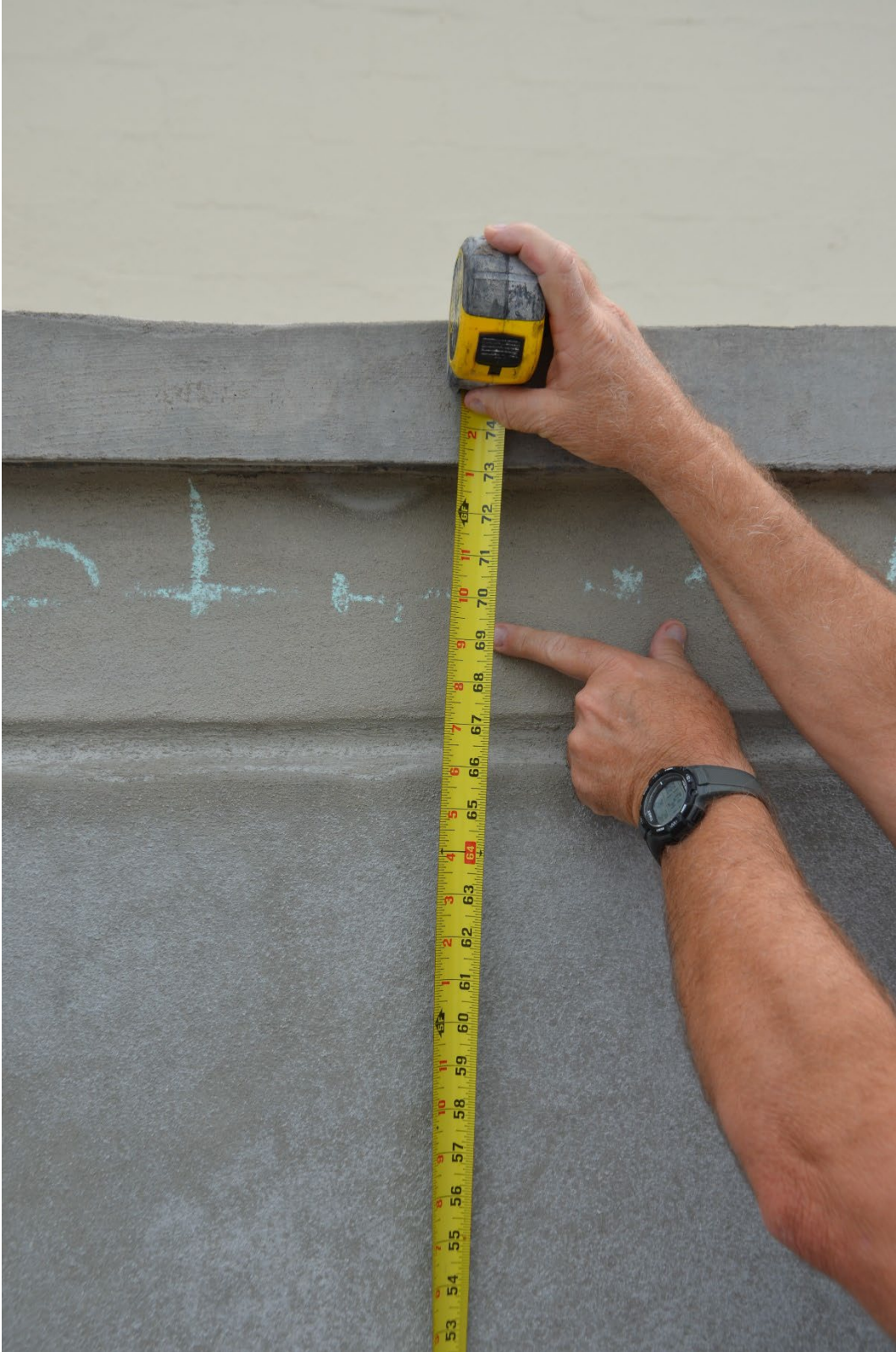
Figure 5-78: Hurricane Ian HWM along the west side of Everglades City School (Collier County, Zone AE)
