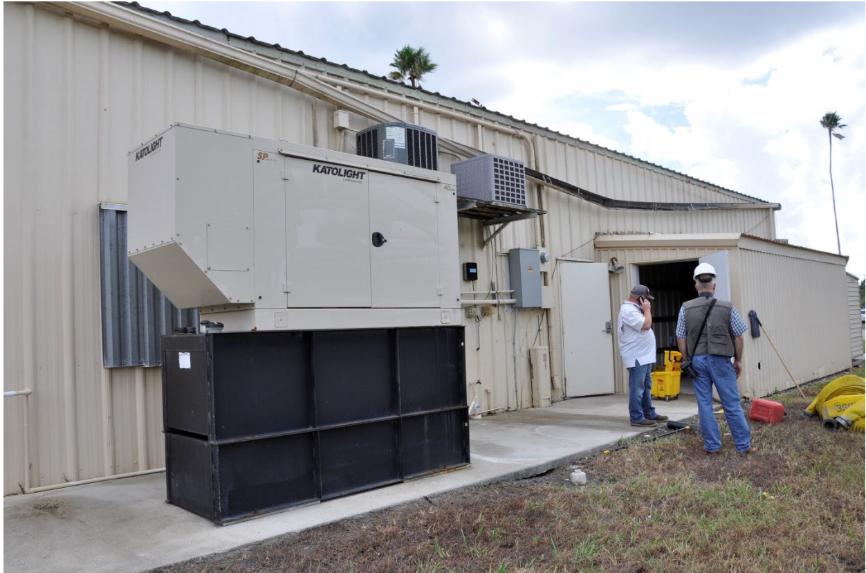
Figure 5-53: Everglades City Fire Station #60 with an elevated generator in the foreground (Collier County, Zone AE)
