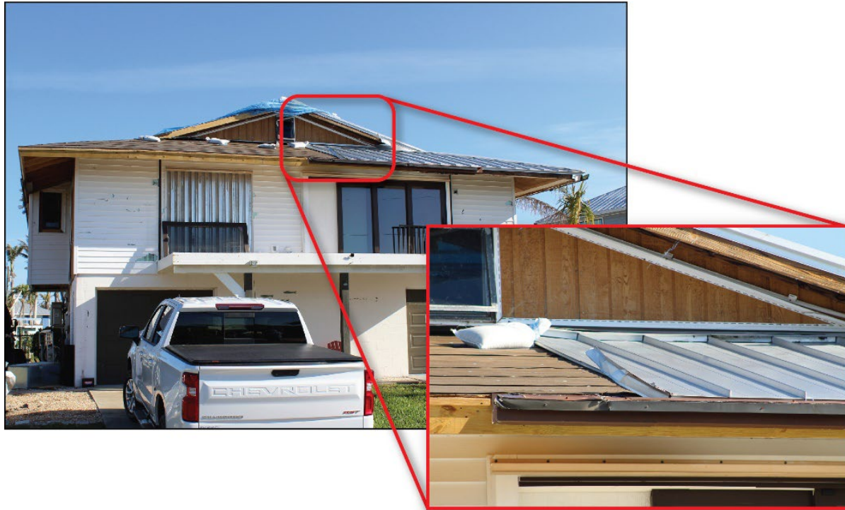
Figure 4-27: A house with a standing seam metal panel roof that was replaced in 2018 with severe damage (EWS = 115 mph; DWS = 161 mph) (St. James City)
