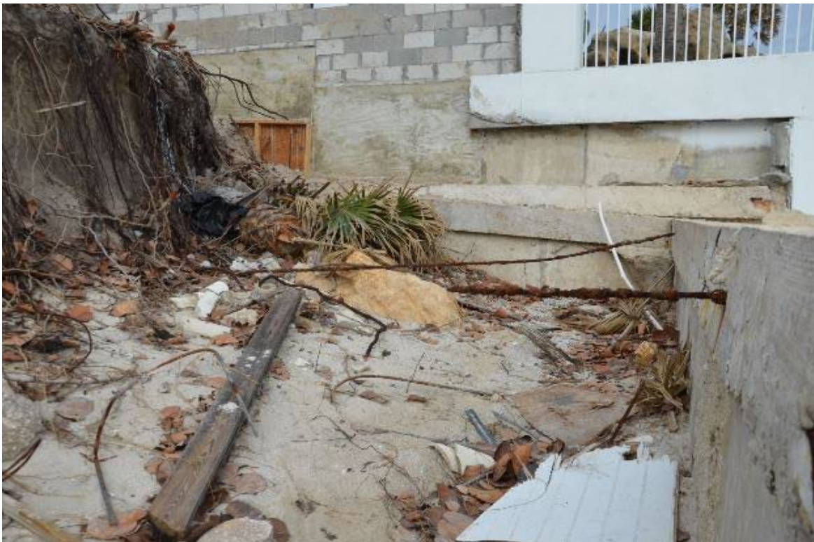
Figure 3-35: Corroded tie-back system of a coastal protection structure (Volusia County, Zone VE)
