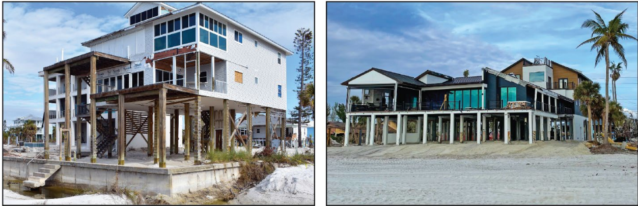
Figure 3-19: Single-family houses built in 2000 (left) and 1994 (right) in Fort Myers Beach with intact decks and porches (Lee County, Zone VE, Seaward of the CCCL)
