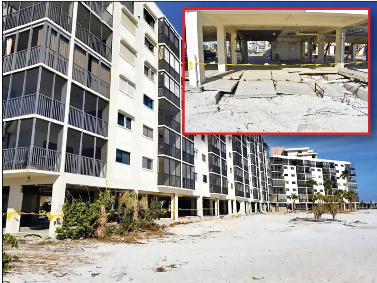
Figure 3-20: Frangible concrete slabs breaking up as intended due to the erosion of sand supporting them on Fort Myers Beach (Lee County, Zone AE, Seaward of CCCL)
