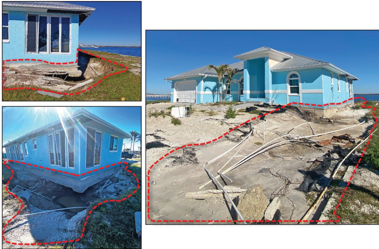
Figure 3-27: Scour surrounding a house and undermining the foundation in Matlacha (Lee County, Zone AE)
