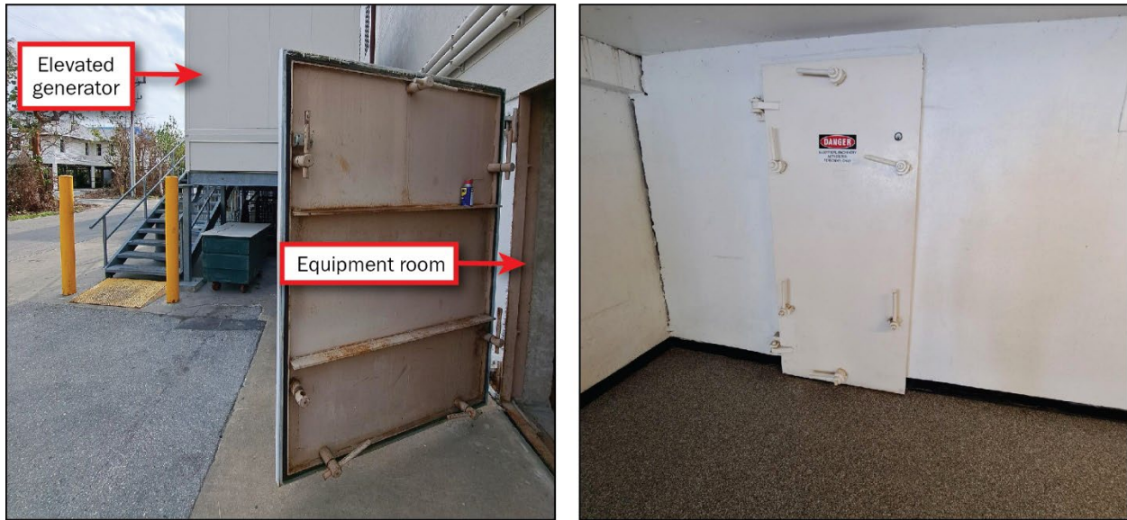
Figure 3-92: Vaulted doors prevented floodwater from entering the equipment rooms (Lee County, Zone AE)
