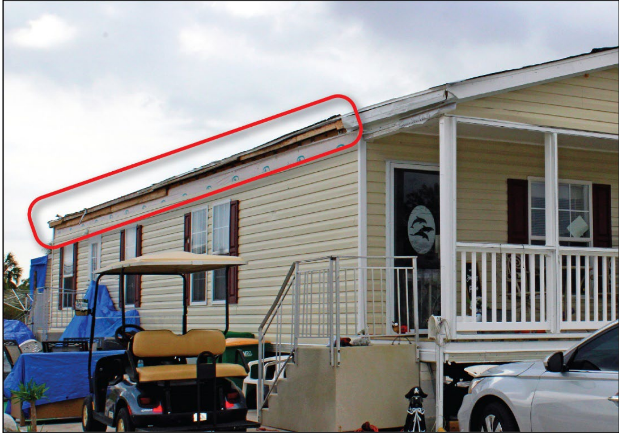
Figure 4-54: A 2019 manufactured home where the loss of the carport damaged the main unit where it was attached, as indicated by the red rectangle (EWS = 126 mph) (Charlotte County)
