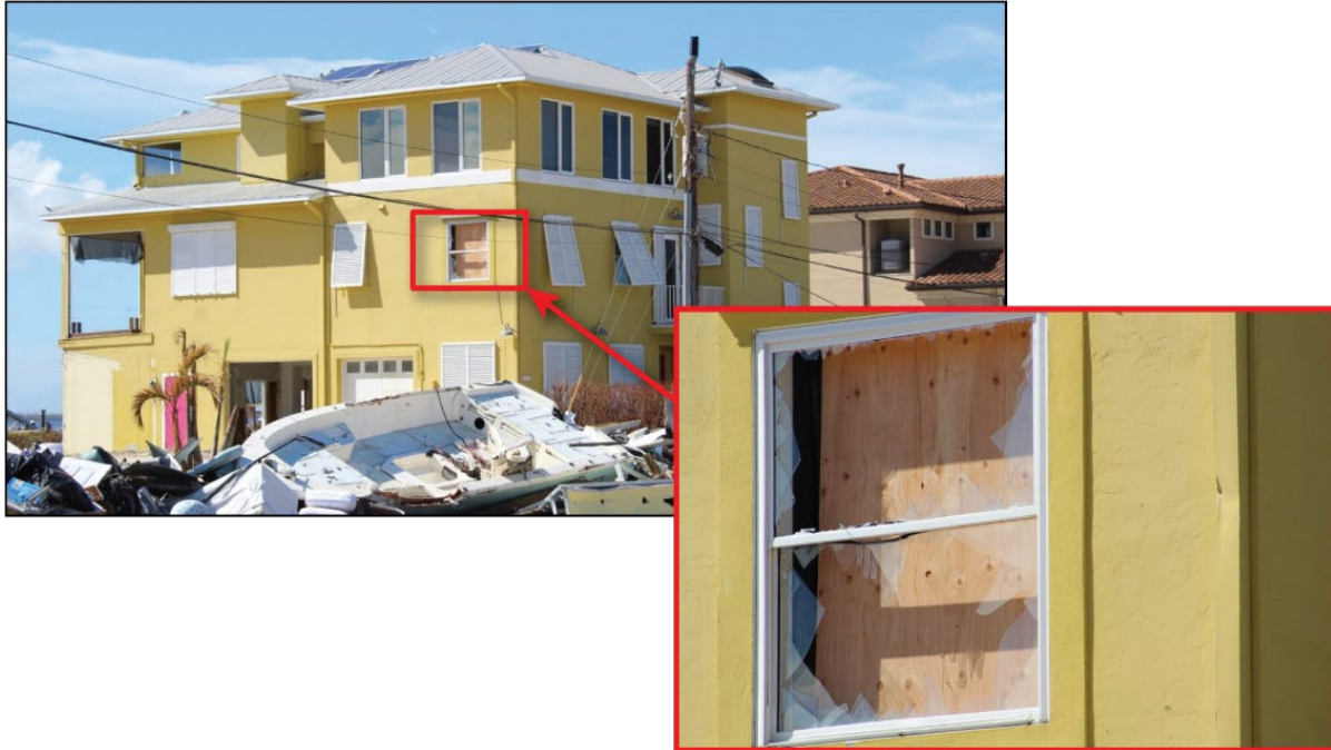
Figure 4-7: A house built in 2003 with glazed opening damage (EWS = 114 mph; DWS = 160 mph) (St. James City)
