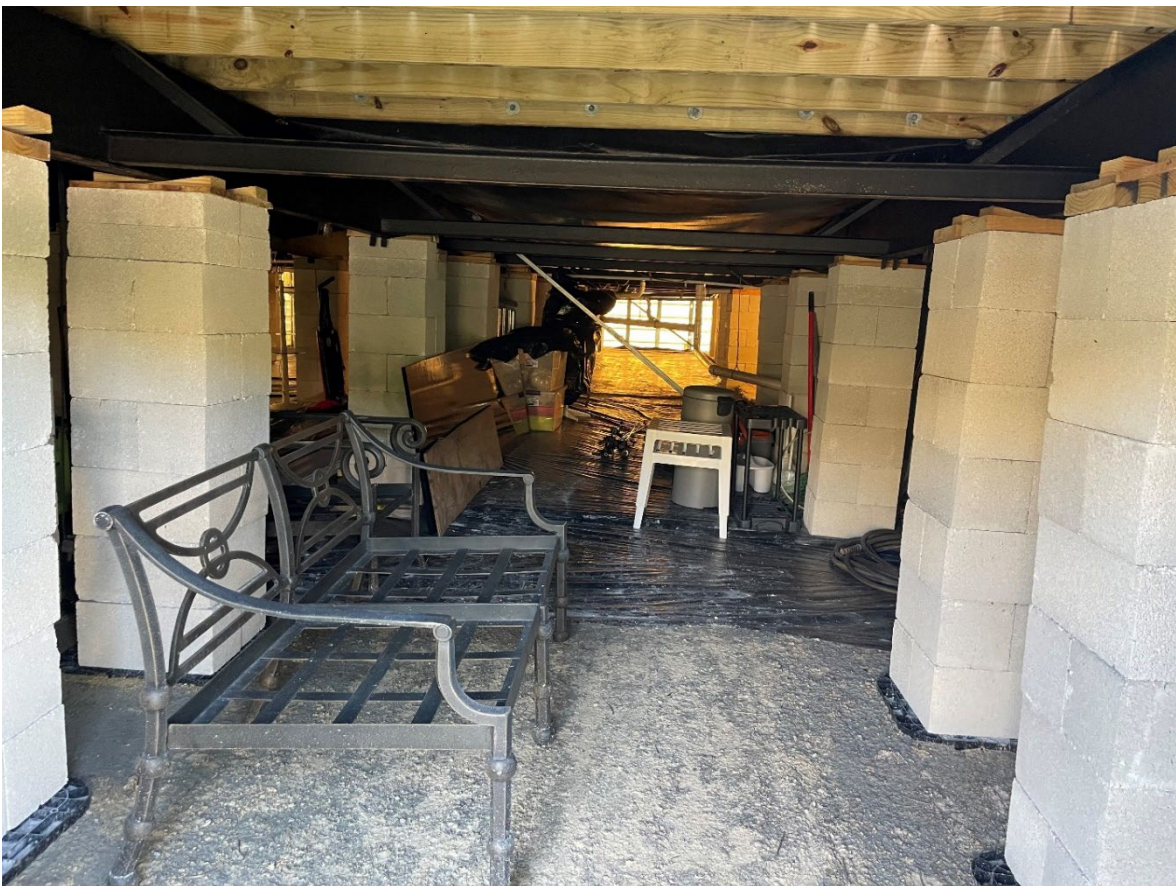
Figure 3-138: Representative foundation for newer elevated manufactured home in the Naples Land Yacht Harbor Community (Collier County, Zone AE)
