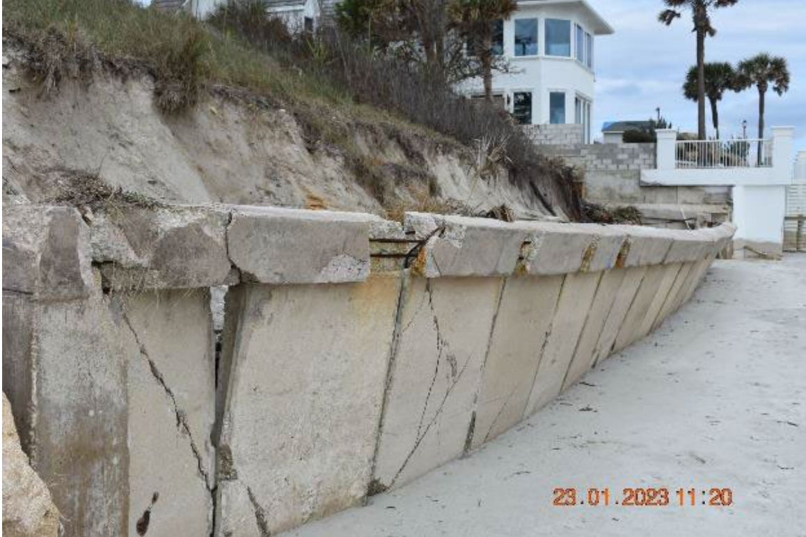
Figure 3-34: Failed coastal protection wall rotating seaward (Volusia County, Zone VE)
