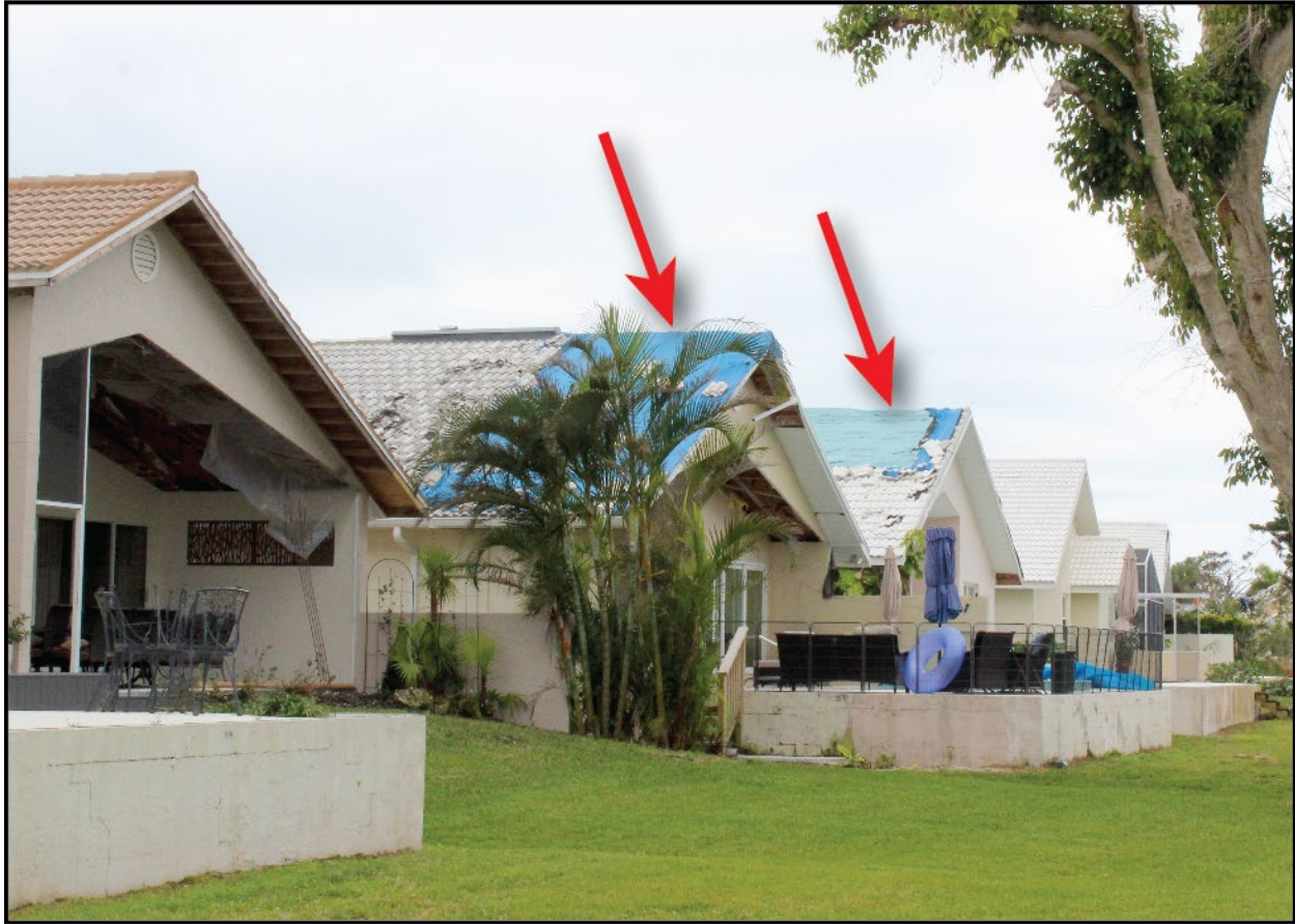
Figure 4-41: Roof tile damage to older tile roofs in Placida (EWS = 126 mph)
