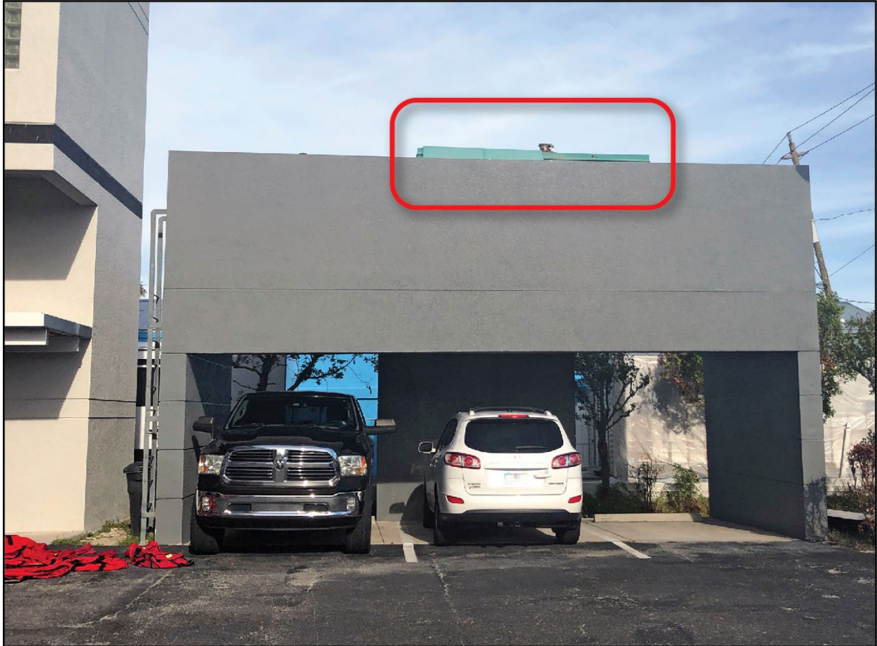
Figure 5-39: Elevated standby generator (behind wall) (Lee County, Zone AE)
