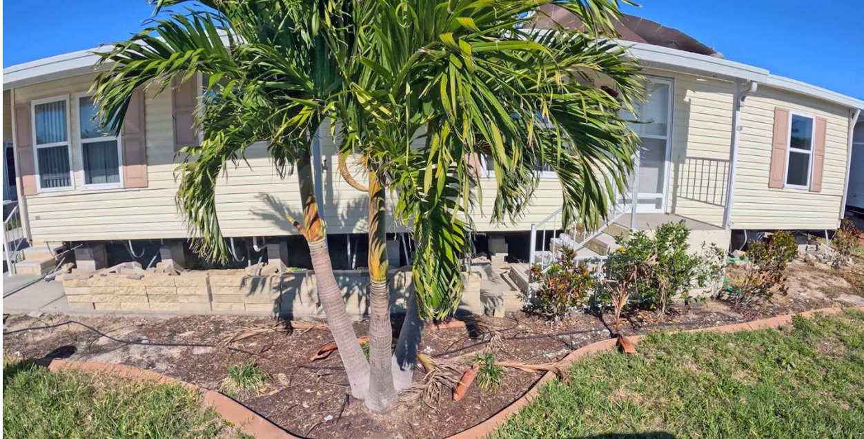
Figure 3-122: Representative manufactured home along Adam Drive that had interior flood damage, elevated approximately 2 feet above ground (Lee County, Zone AE)
