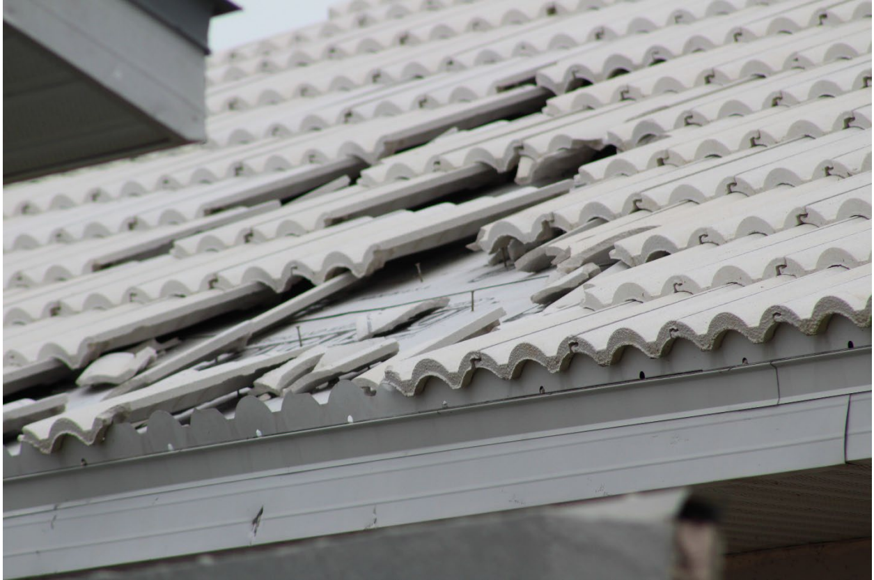
Figure 4-40: Mechanically fastened tile roof in Placida that was replaced in August 2021 (EWS = 126 mph)
