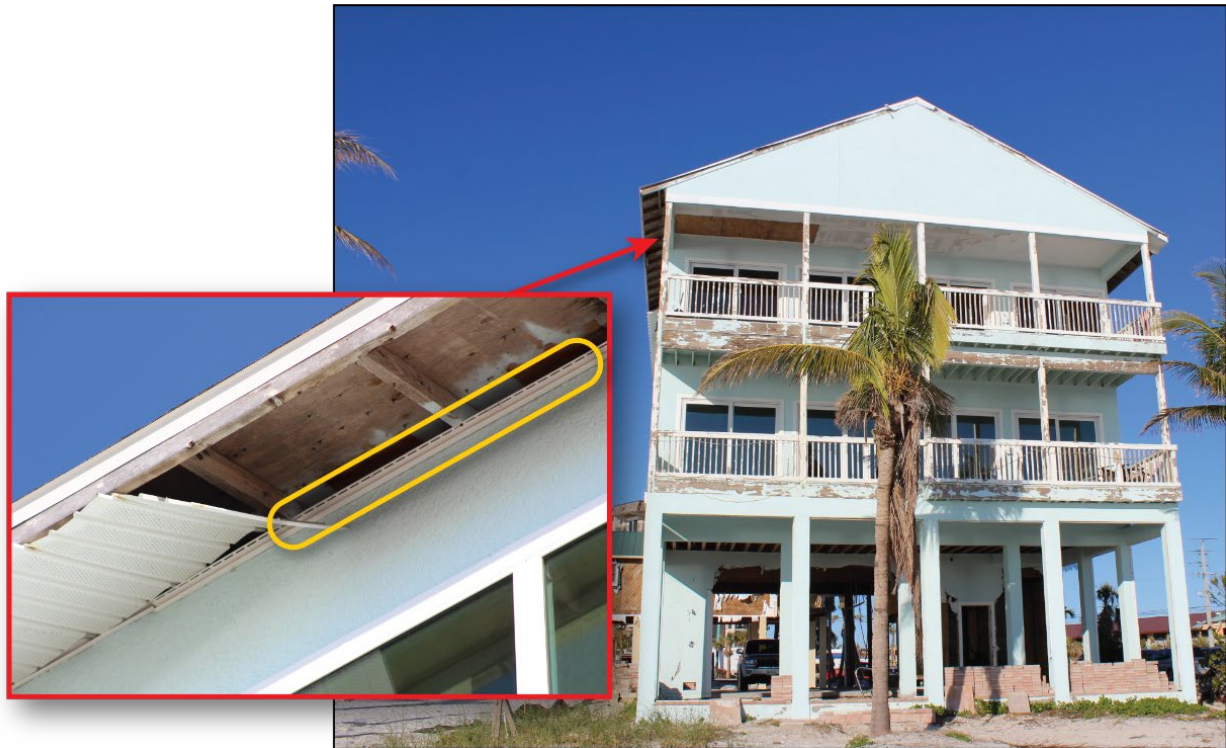
Figure 4-2: House built in 2015 with roof covering and vinyl soffit damage (estimated wind speed [EWS] = 103 mph; design wind speed [DWS] = 159 mph) (Fort Myers Beach)
