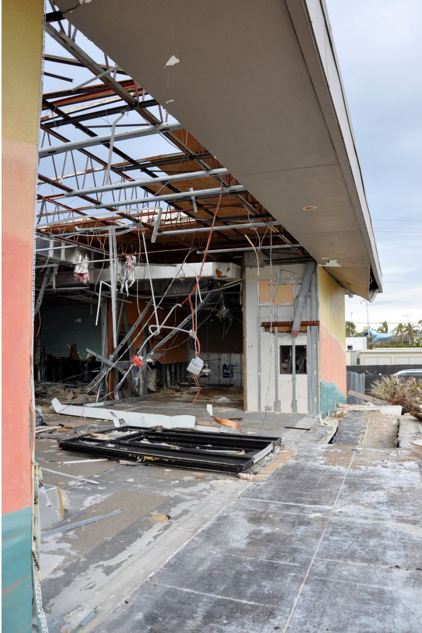
Figure 3-76: Fort Myers Beach Town Hall south-facing wall following Hurricane Ian (Lee County, Zone AE)
