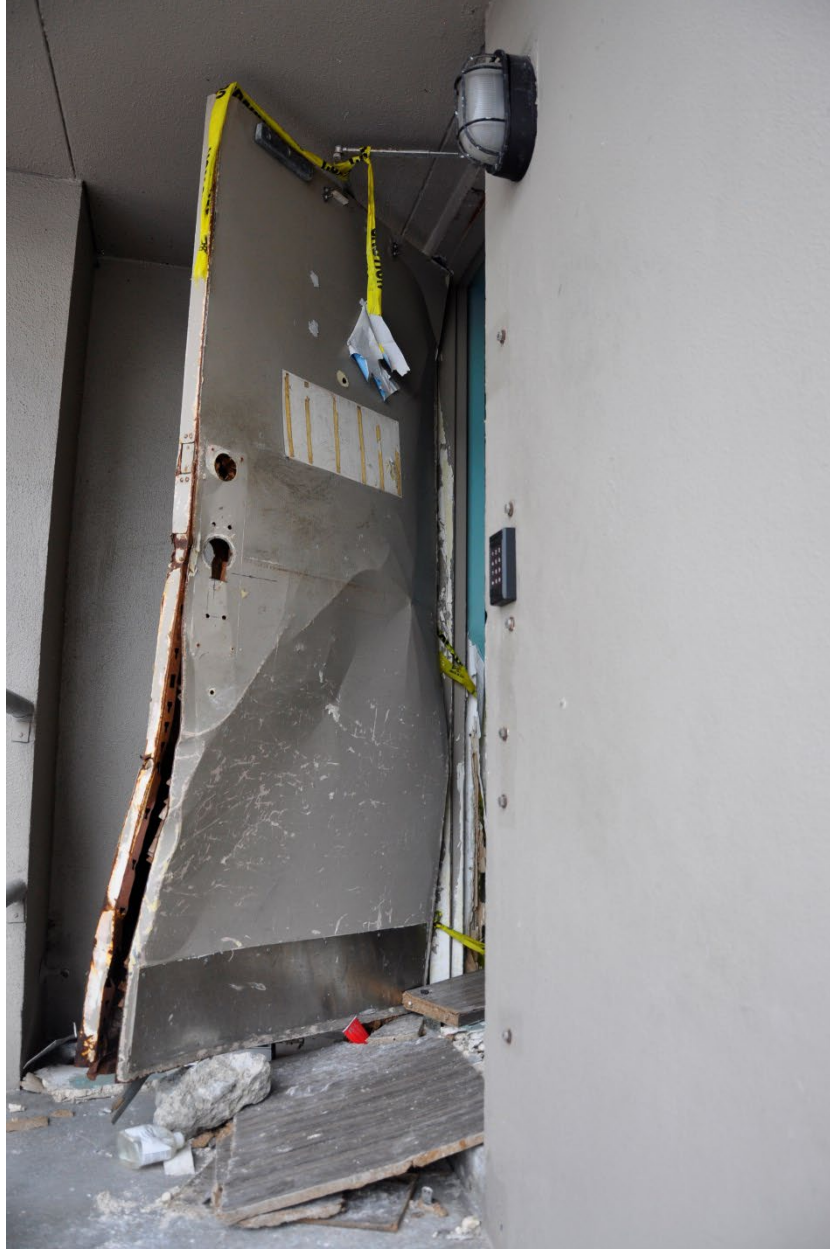
Figure 3-80: Employee entrance door blown out by flood loads at Fort Myers Beach Town Hall (Lee County, Zone AE)
