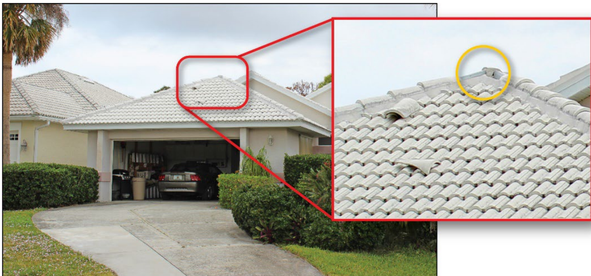
Figure 4-42: Roof tile damage to a roof in Placida that was replaced in September 2019 (EWS = 126 mph)
