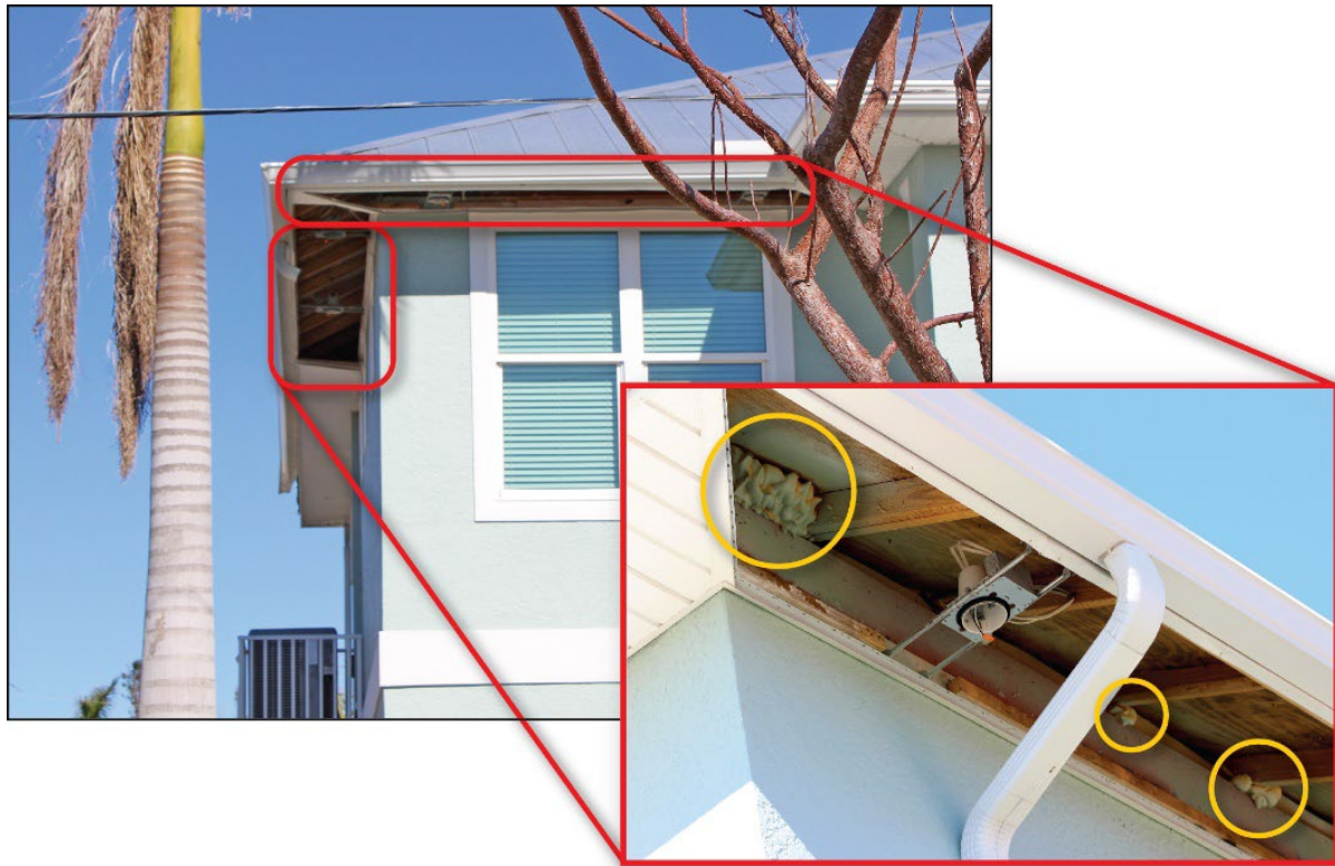
Figure 4-3: Post-FBC house (built in 2021) with vinyl soffit damage exposing the sprayed foam insulation in the attic (EWS = 109 mph; DWS = 161 mph) (Sanibel)
