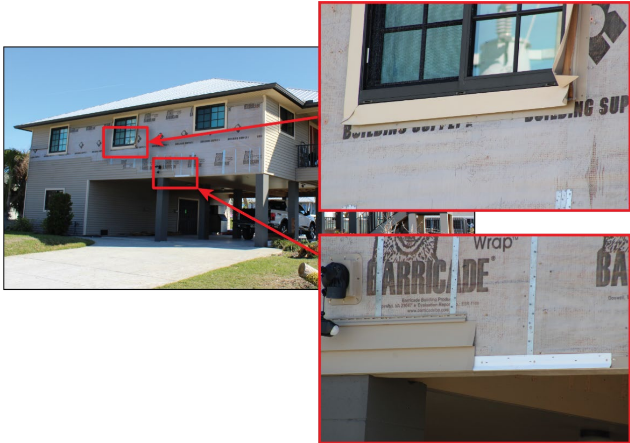
Figure 4-5: A house built in 2014 with significant damage to the vinyl siding on the west side (EWS = 114 mph; DWS = 160 mph) (St. James City)
