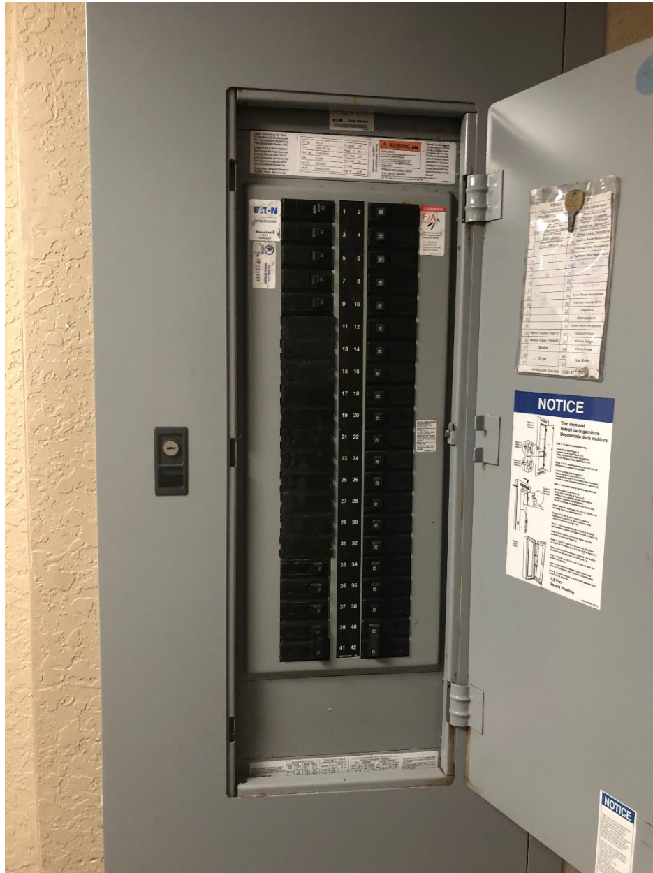
Figure 5-64: Third-floor panelboard that experienced water entry during Hurricane Ian (Lee County)
