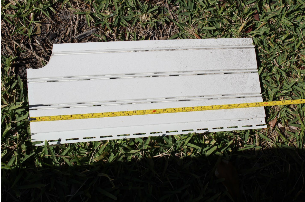
Figure 4-4: A vinyl soffit panel spanning approximately 24 inches that blew off the 2021 residence in Figure 4-3 (EWS = 109 mph; DWS = 161 mph) (Sanibel)
