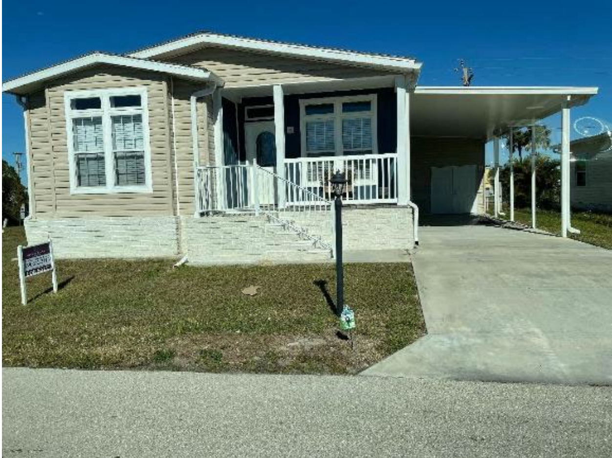
Figure 3-118: 2019 Elevated manufactured home in the Old Bridge Village with no foundation damage and primary flood damage limited to crawlspace and storage unit (Lee County, Zone AE)
