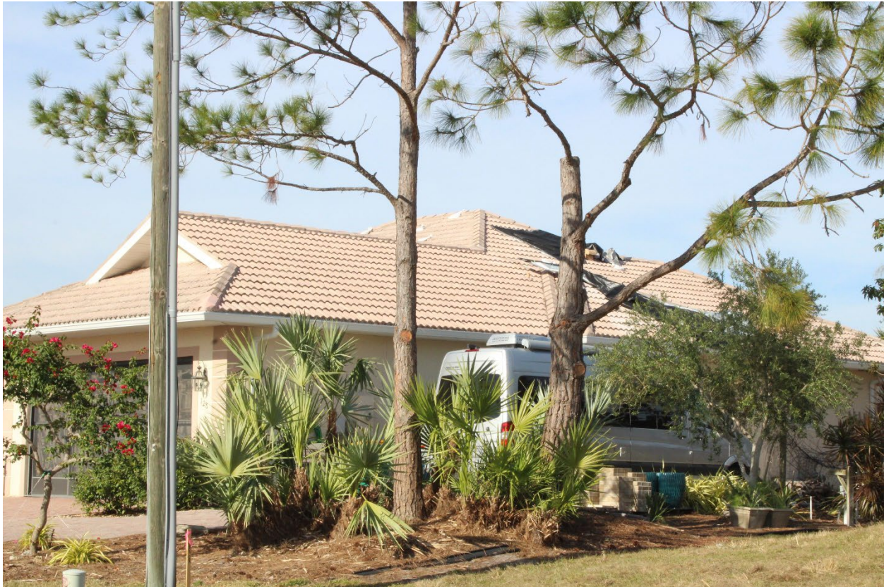
Figure 4-38: A house built in 2001 with a tile roof (tile damage as indicated by black tarp on the roof) (EWS = 128 mph) (Port Charlotte)
