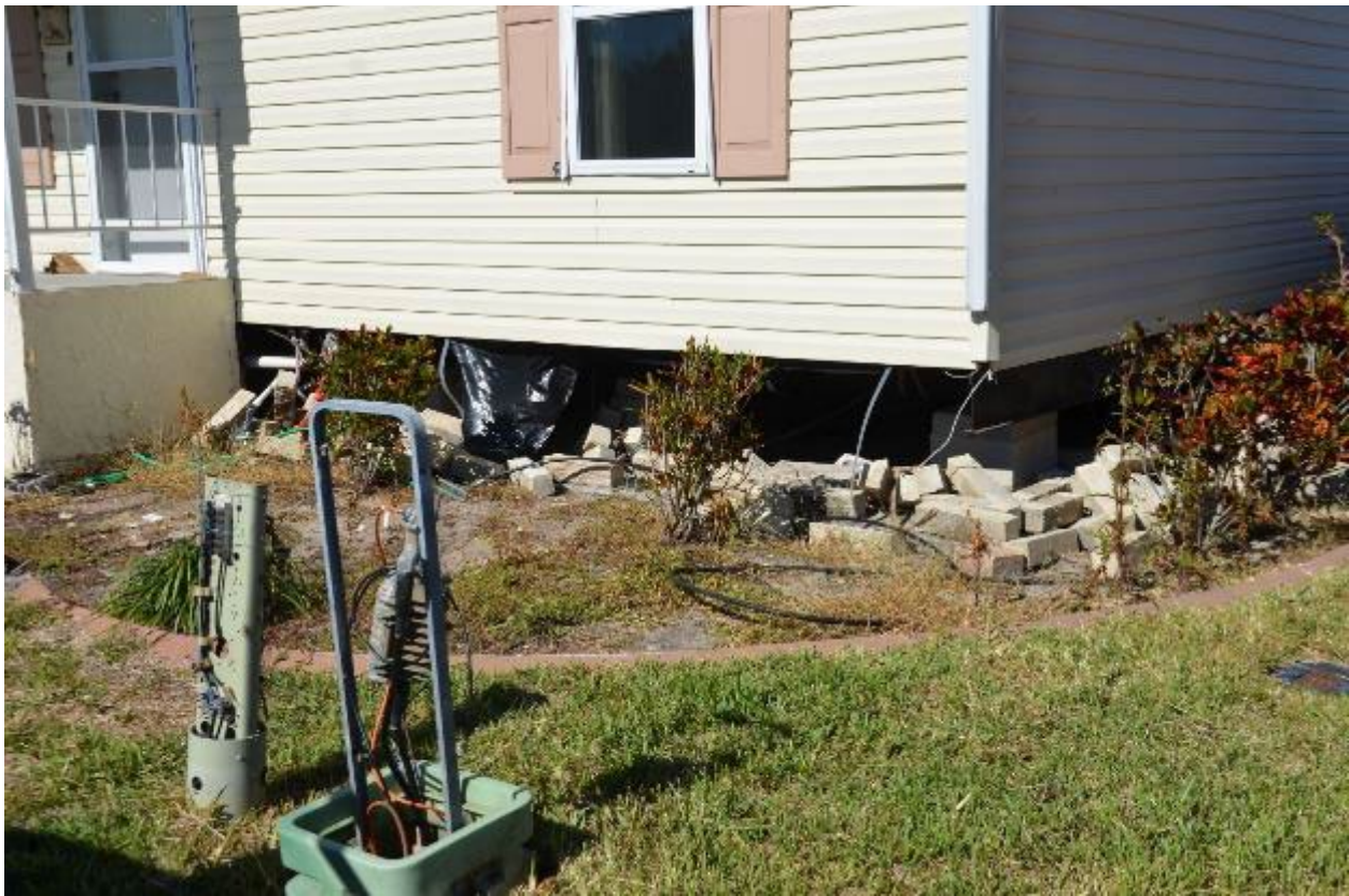
Figure 3-114: Typical manufactured home damage observed in Old Bridge Village (Lee County, Zone AE)
