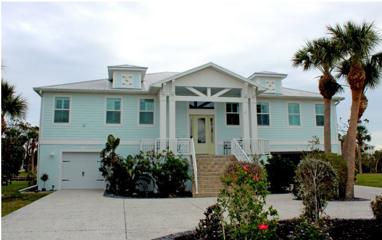
Figure 4-26: A house built in 2015 with a through-fastened metal roof with no damage observed (EWS = 120 mph; DWS = 160 mph) (Placida)
