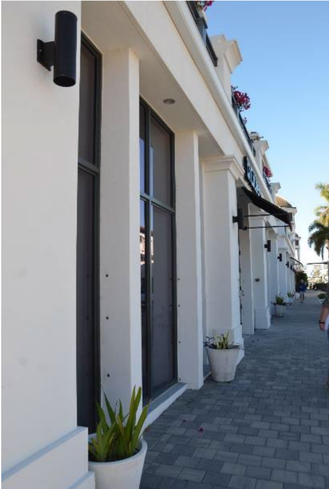
Figure 3-69: Dry floodproofed retail building; note anchors on each side of the window frame to support opening barriers (Collier County, Zone AE)
