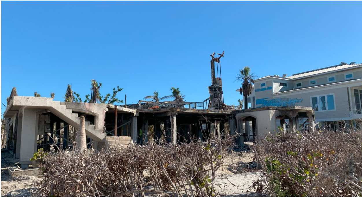
Figure 3-6: House destroyed by fire spread from an EV fire in a neighboring house (Lee County, Zone AE and VE)
