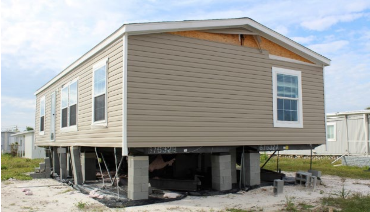
Figure 4-58: Manufactured home with shifted, unstable dry-stack pier foundation; observations included a HWM approximately 6 inches above the top of the finished floor (Lee County)
