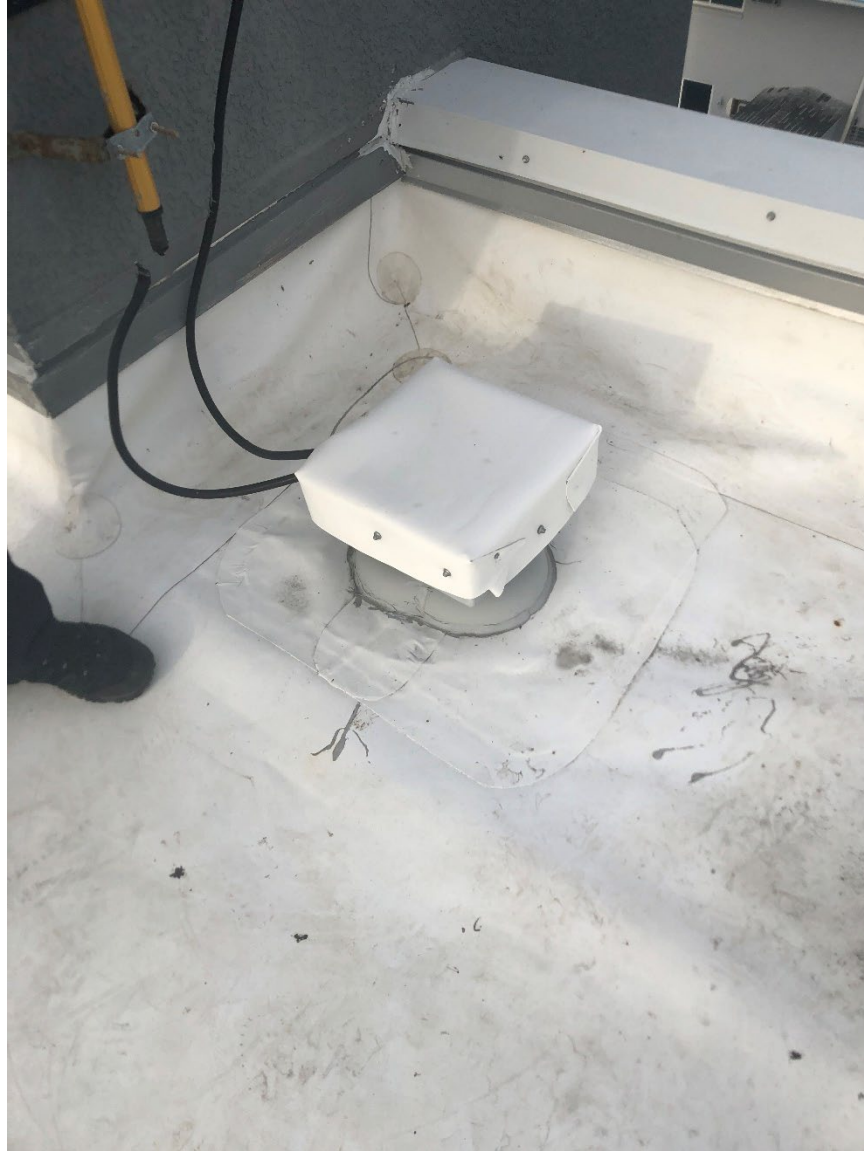
Figure 5-65: Roof cap for communication cables that was dislodged during Hurricane Ian (Lee County)
