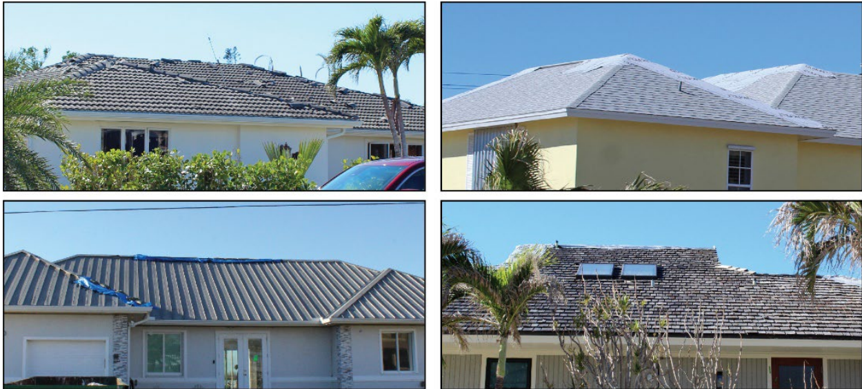
Figure 4-11: Hip and ridge damage on four residences with different roof types: a tile roof (top left), asphalt shingle roof (top right), metal panel roof (bottom left), and cedar shake roof (bottom right)
