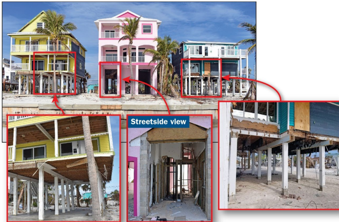
Figure 3-59: Examples of damage observed for each of the three remaining waterfront structures
