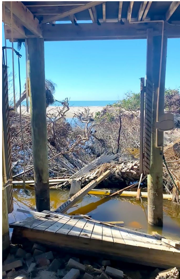
Figure 3-22: Scour channel and debris near deep pile foundation (Lee County, Zone VE, Seaward of CCCL)
