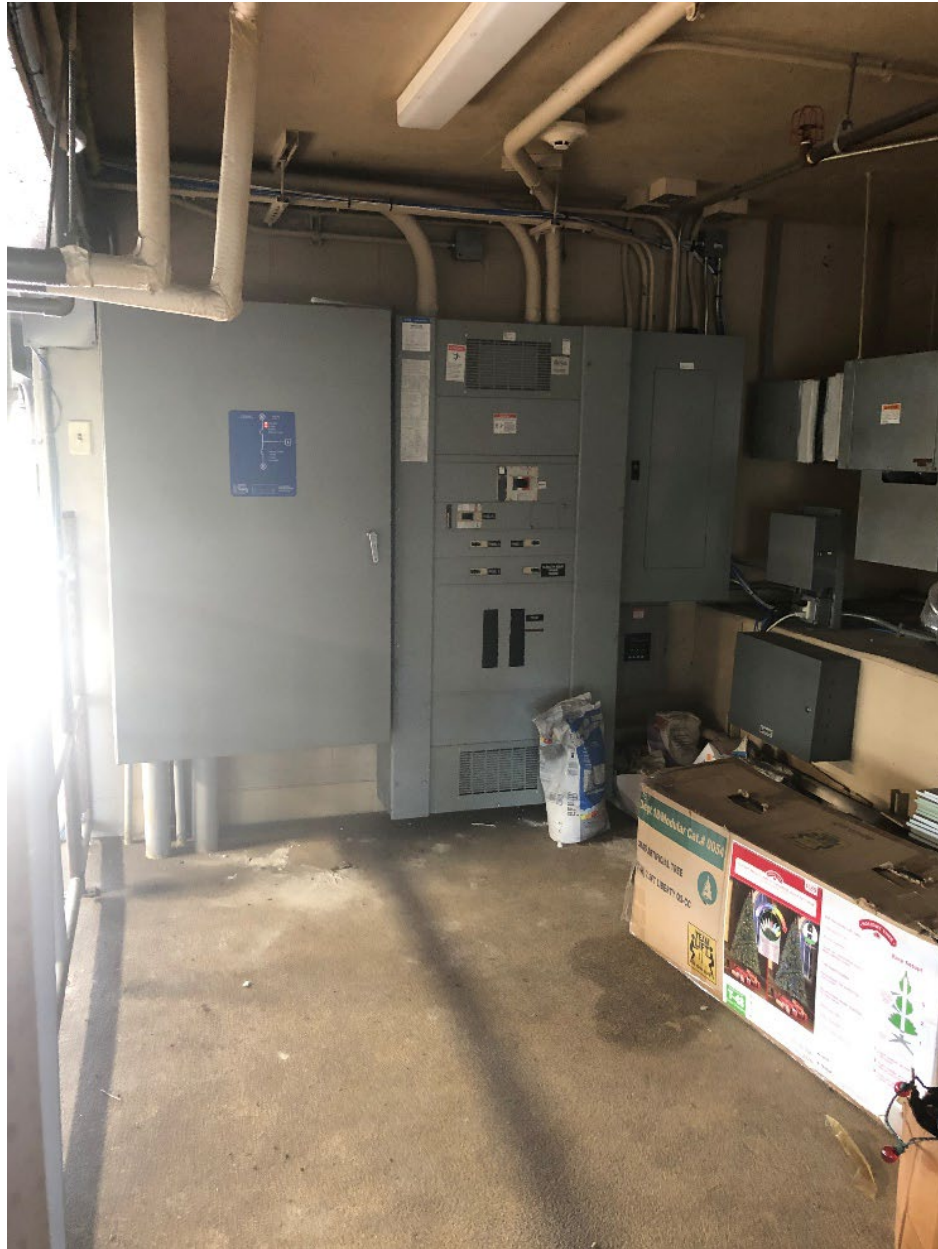
Figure 5-38: Elevated electrical service and distribution equipment on the mezzanine above the apparatus bay (Lee County, Zone AE)
