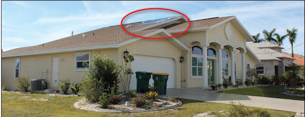
Figure 4-15: An asphalt shingle roof that was replaced in 2022 with minor damage near the ridge (EWS = 128 mph; DWS = 150 mph) (Port Charlotte)
