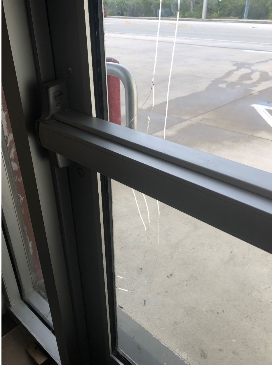
Figure 5-43: Front door glazing damaged by floodwater (Lee County, Zone AE)
