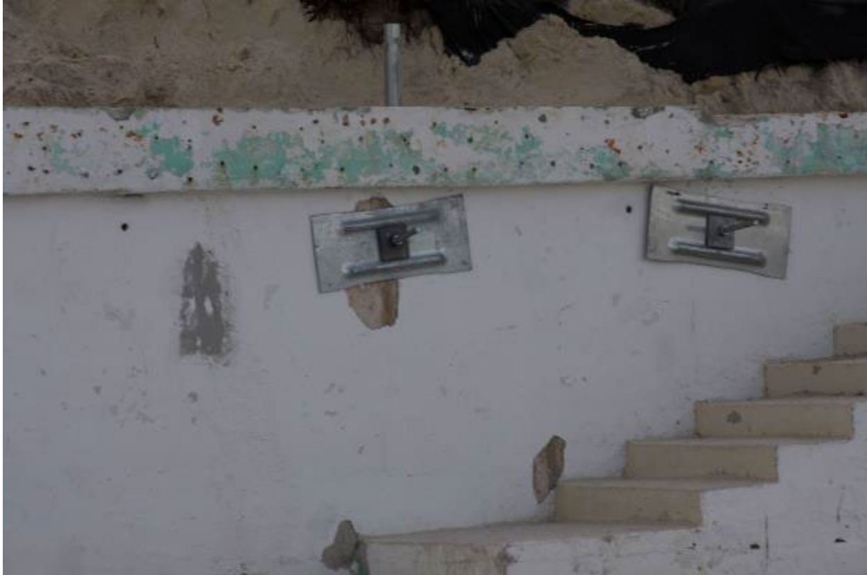
Figure 3-38: Emergency repairs to account for corroded tie-backs (Lee County, Zone VE)
