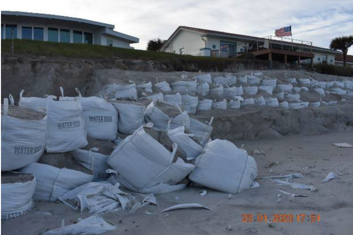
Figure 3-41: Sediment-filled bags used to counteract further coastal erosion in an area of Port Orange where seawalls were destroyed (Volusia County)
