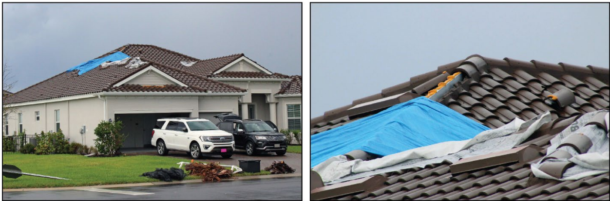
Figure 4-43: Roof tile damage (EWS = 126 mph; DWS = 153 mph) (Port Charlotte)
