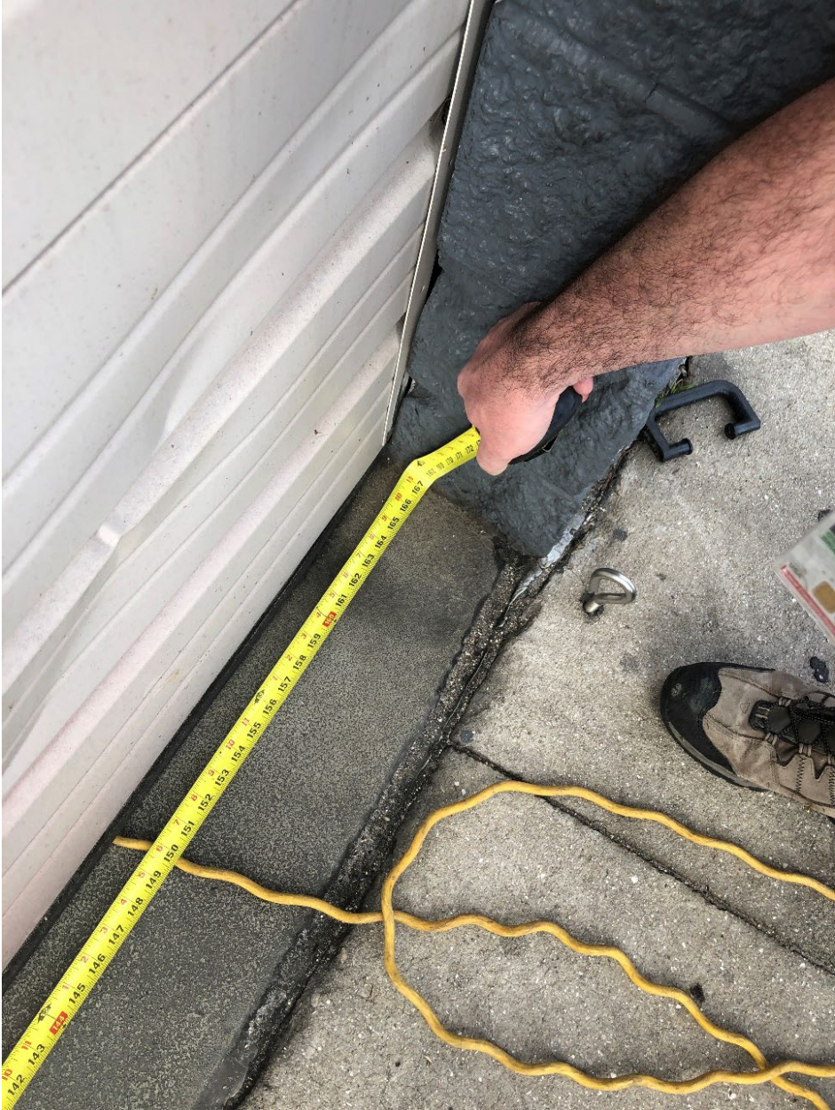
Figure 5-70: Damage to apparatus bay door (Charlotte County)
