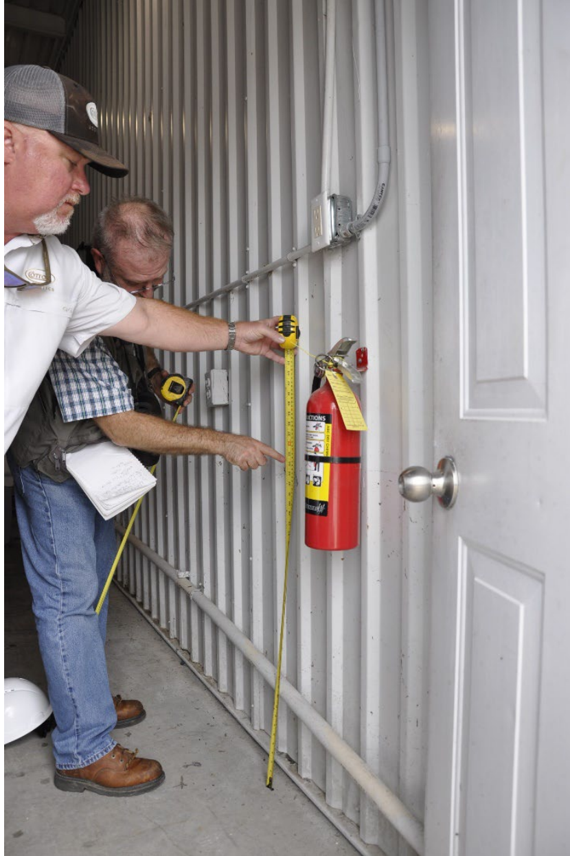
Figure 5-54: Everglades City Fire Station #60 with HWM (Collier County, Zone AE)
