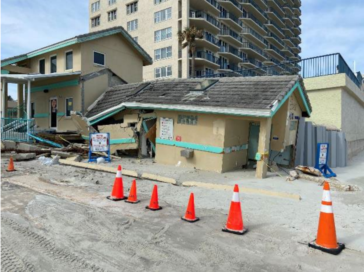
Figure 3-108: Destroyed public restroom in Daytona Beach Shores (Volusia County, Zone VE, Seaward of CCCL)
