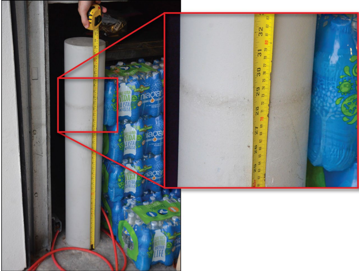
Figure 5-46: 28-inch HWM at City of Naples Fire Station #1 (Collier County, Zone AE)
