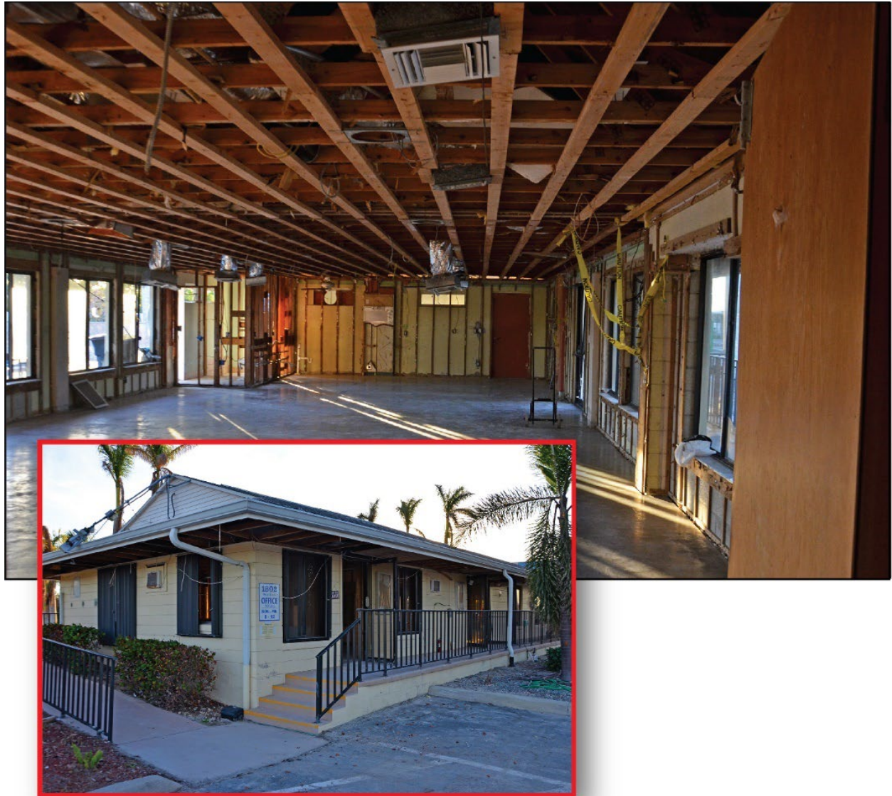
Figure 3-126: Representative interior damage in the office building for Port Carlos Cove (Lee County, Zone VE)
