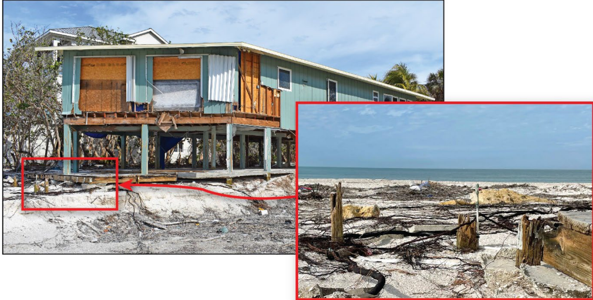
Figure 3-44: Deteriorated wood supports in Bonita Springs that failed during Hurricane Ian
