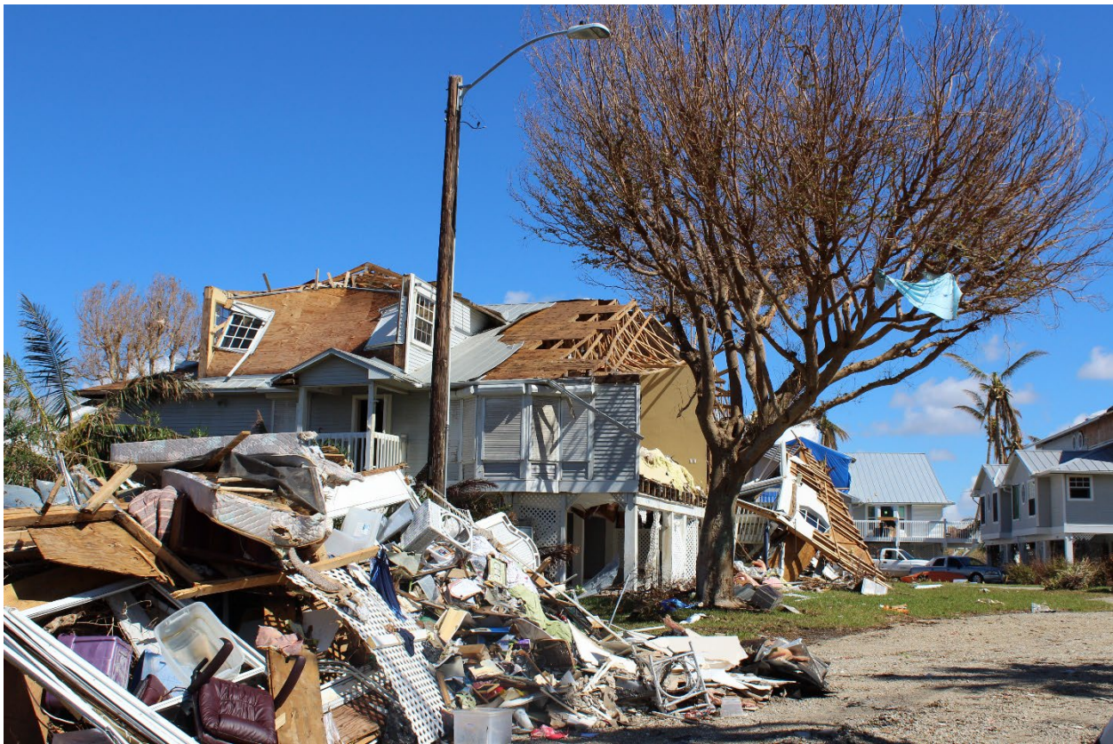
Figure 4-46: A Pre-FBC two-family home (built in 1990) with severe structural damage from wind (EWS = 113 mph) (St. James City)
