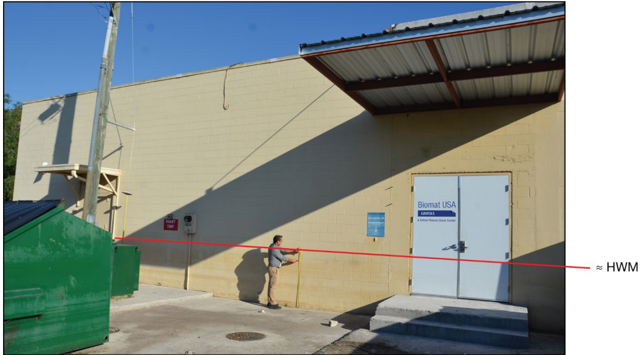
Figure 3-102: Rear of shopping center where a 42-inch HWM was identified (Orange County, Zone AE)
