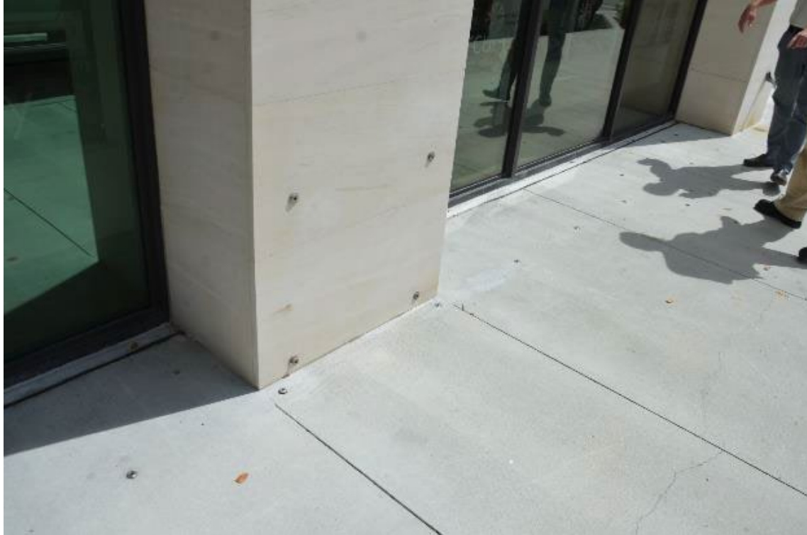
Figure 3-65: Anchors for active dry floodproofing measures on building in downtown Naples (Collier County, Zone AE)
