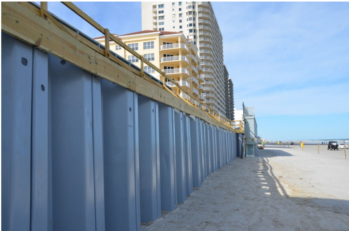
Figure 3-42: Vertical vinyl sheet wall piles installed along Daytona Beach to replace destroyed seawalls (Volusia County)
