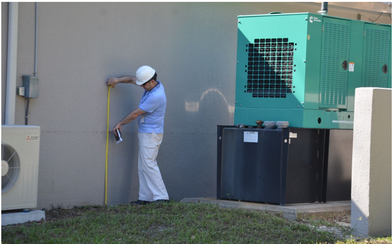
Figure 5-50: Volusia County Fire Station #12 with generator on right, elevated above Hurricane Ian floodwaters (Volusia County)
