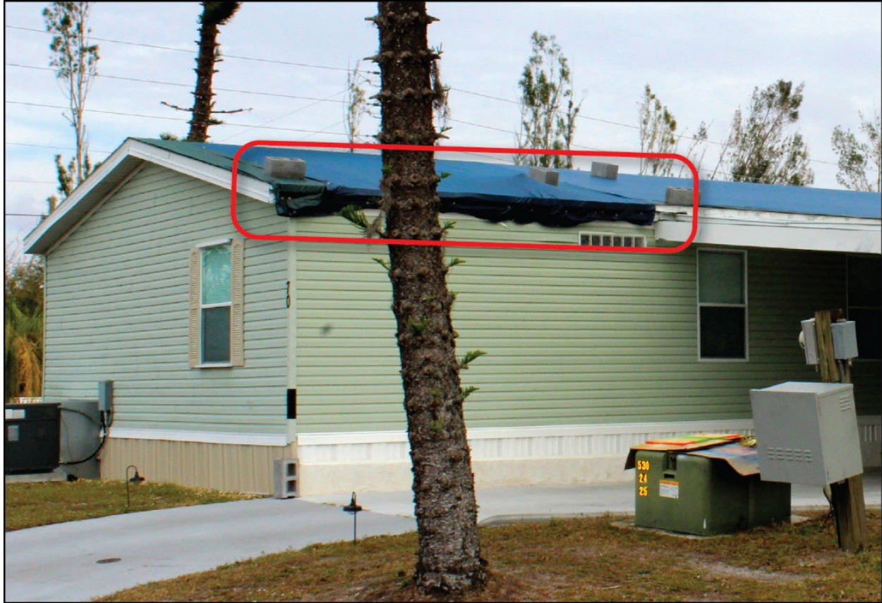
Figure 4-55: 1999 manufactured home; damage to main unit from loss of the front section of the attached carport, as indicated by the red rectangle (EWS = 129 mph) (Charlotte County)
