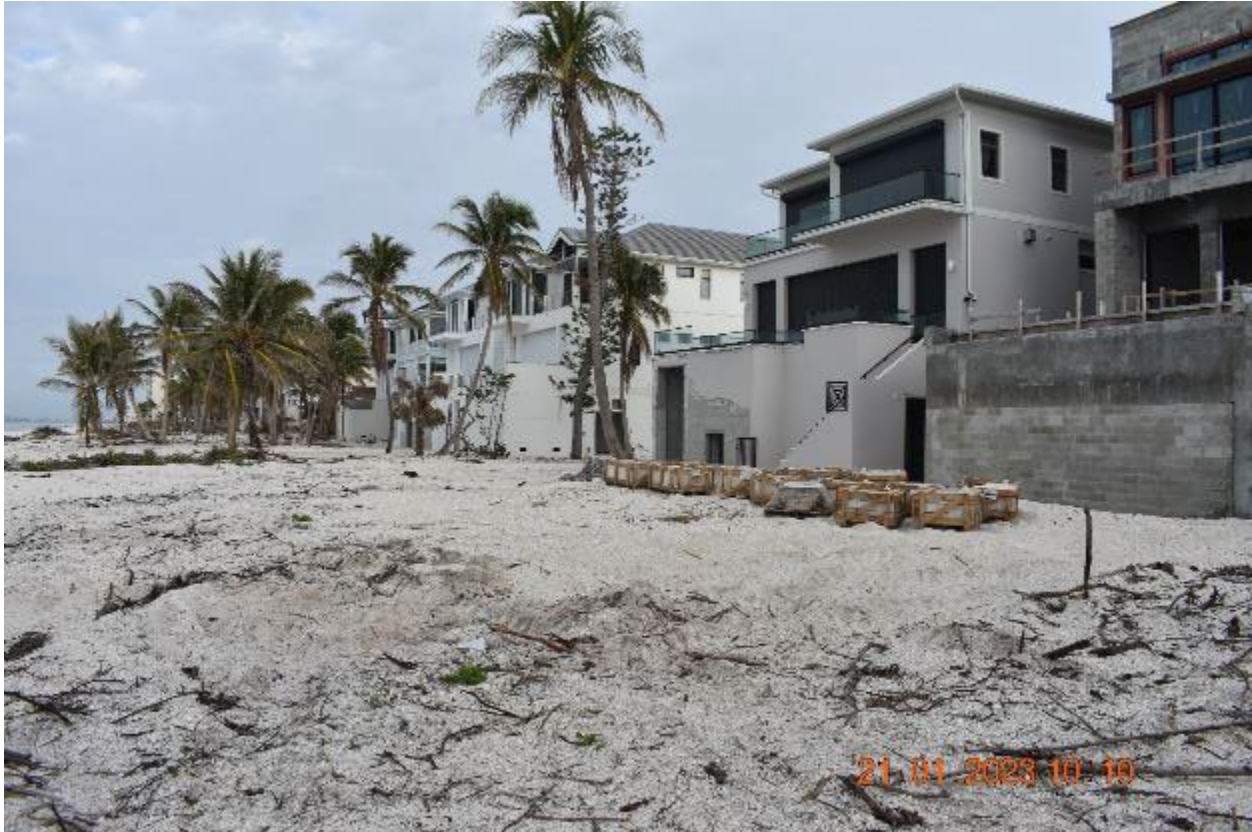
Figure 3-11: Large CMU structures on Bonita Beach (Lee County, Zone VE, Seaward of CCCL)
