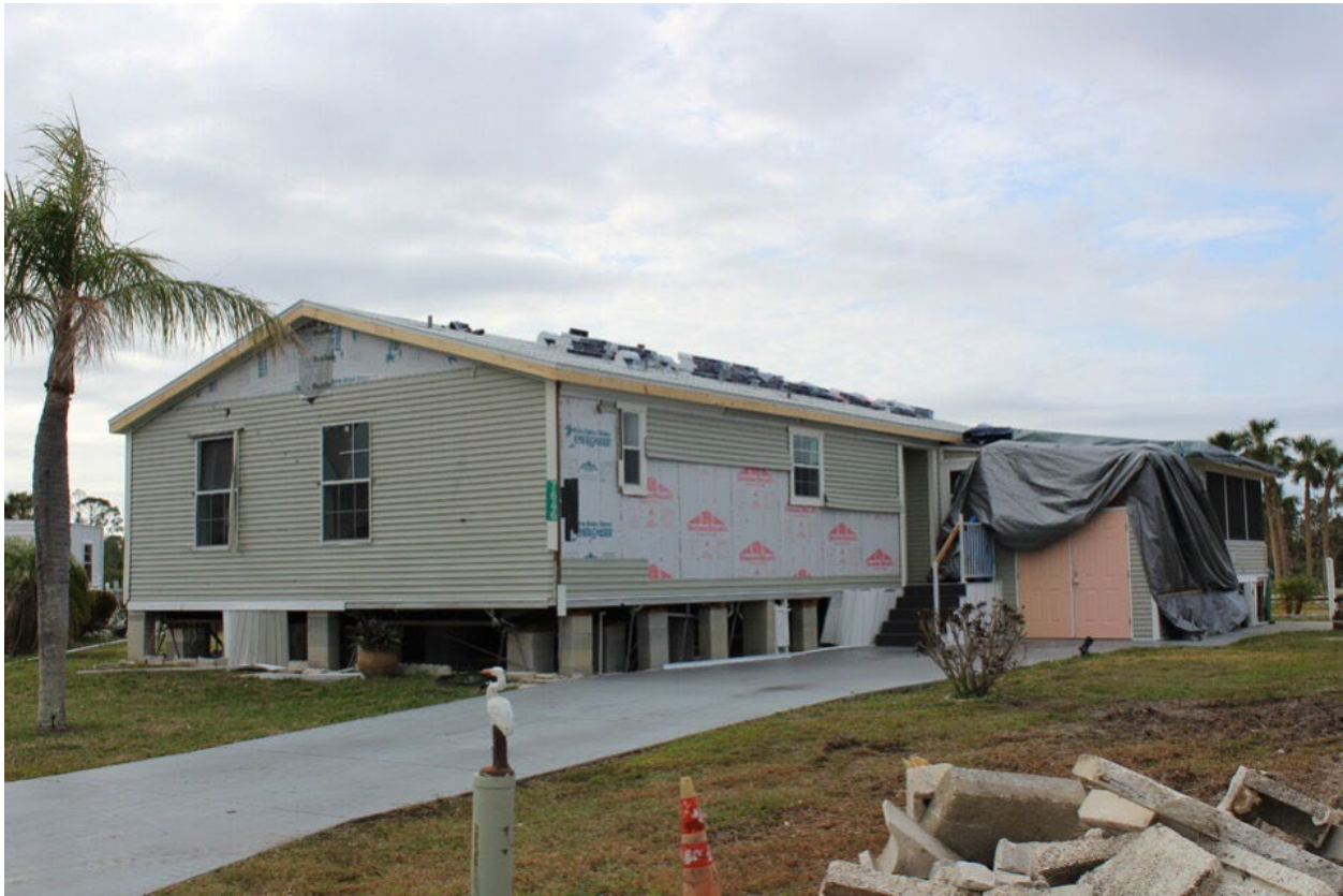
Figure 4-51: Roof covering, wall covering, and fascia damage to post-HUD manufactured home (EWS = 126 mph) (Charlotte County)
