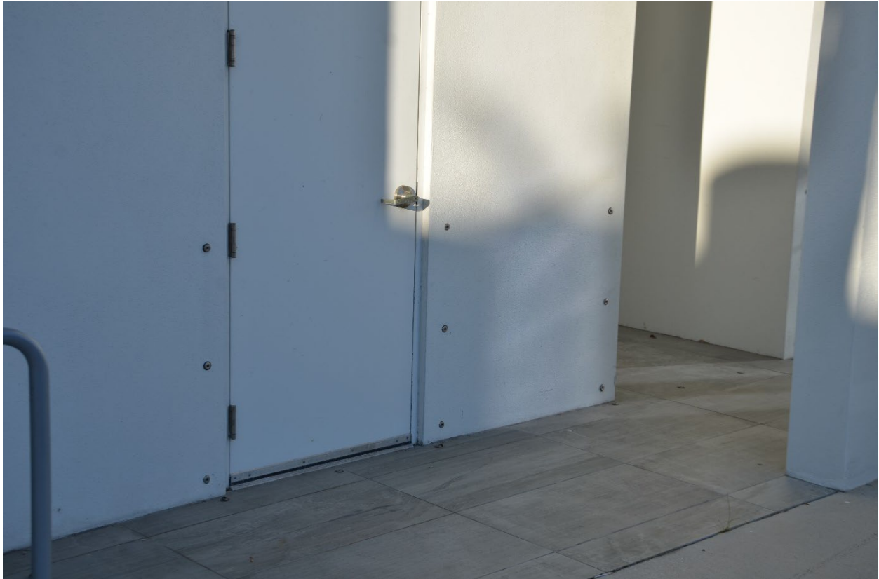
Figure 3-68: Dry floodproofed office building; note anchors on each side of door frame to support opening barriers (Collier County, Zone AE)
