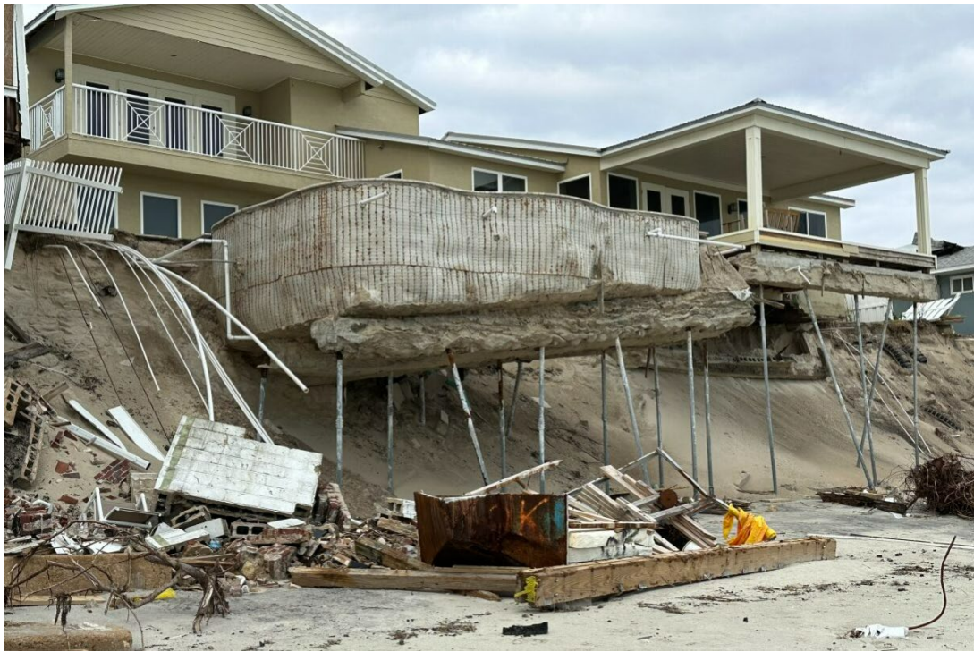
Figure 3-31: Dune erosion in Wilbur-by-the-Sea resulting in exposed foundation micropiles
