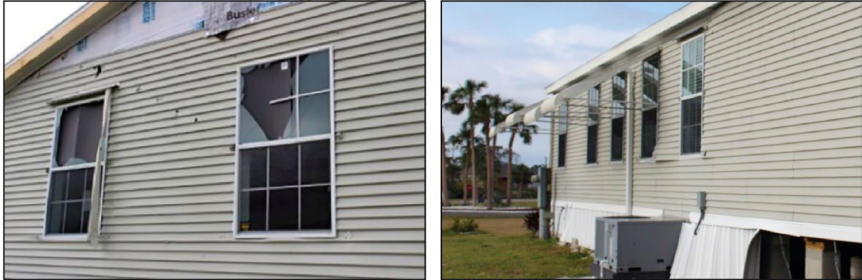
Figure 4-52: Wind-borne debris damage to glazing and non-rated impact protective system (left); aluminum clamshell shutters remain in place on adjacent wall of same post-HUD manufactured home (right) (EWS = 126 mph) (Charlotte County)
