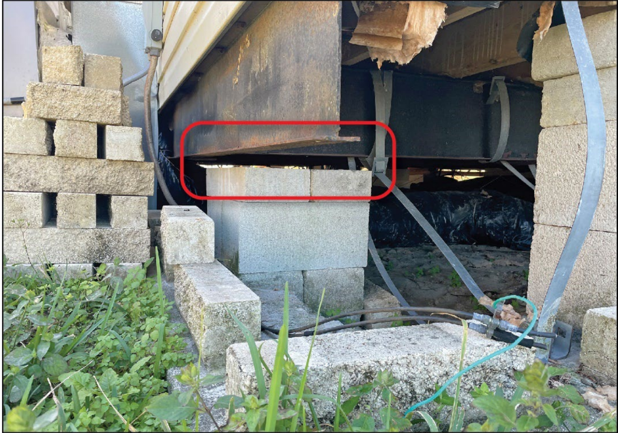
Figure 3-116: Manufactured home unreinforced pier (dry-stacked block) wedges displaced (red circle) during Hurricane Ian flooding (Lee County, Zone AE)
