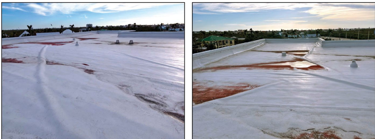
Figure 5-63: Displaced and rippled roof membrane (Lee County)
