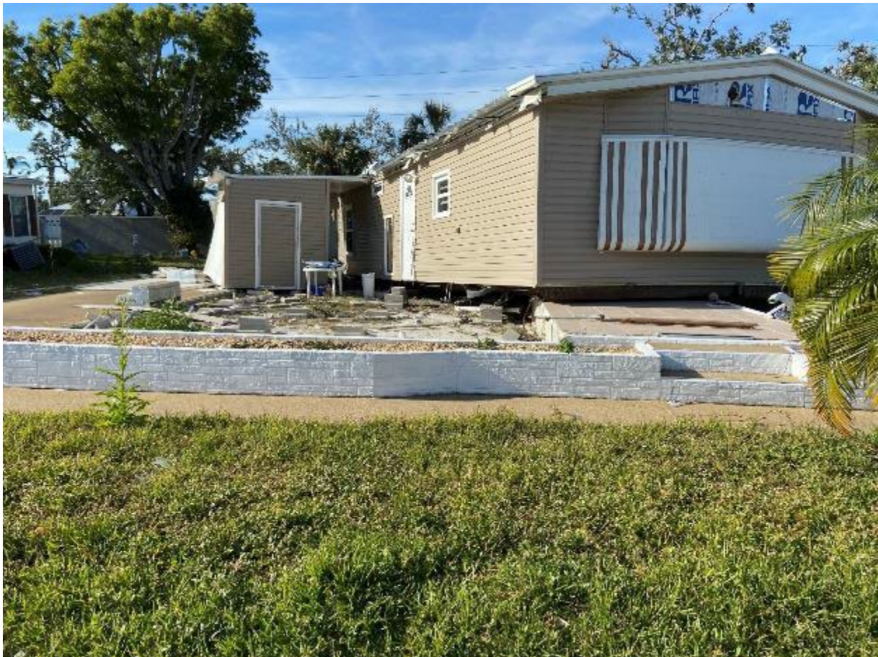
Figure 3-110: Manufactured home displaced from its foundation by flood loads (Lee County, Zone AE)
