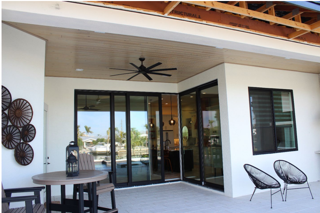
Figure 4-9: A house built in 2021 with two- and three-panel sliding glass doors that experienced significant water intrusion (EWS = 130 mph; DWS = 151 mph) (Punta Gorda)
