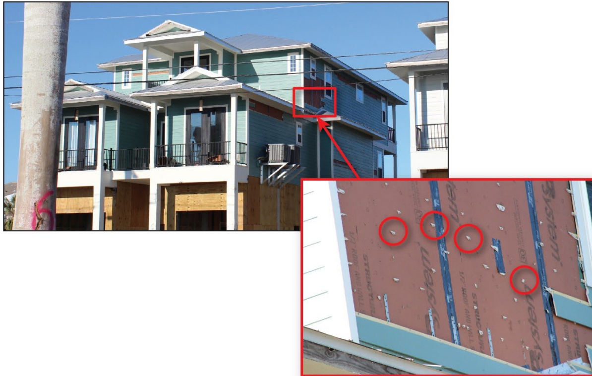
Figure 4-6: A house under construction with fiber cement siding failure (EWS = 104 mph; DWS = 160 mph) (Fort Myers Beach)
