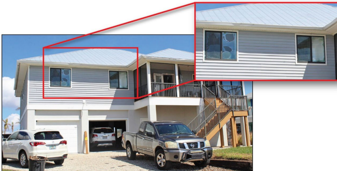
Figure 4-8: A house built in 2016 with glazed opening damage (EWS = 114 mph; DWS = 161 mph) (St. James City)
