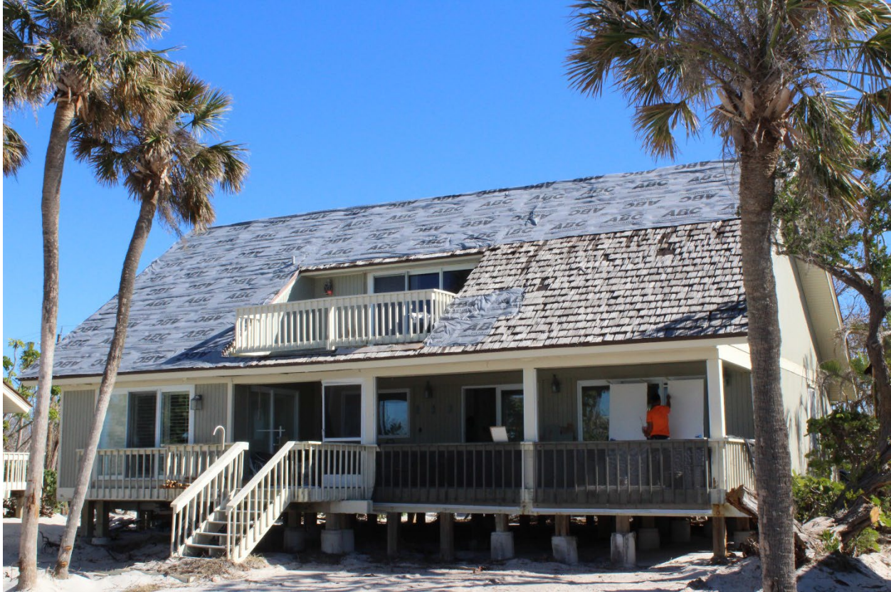
Figure 4-18: A house built in 1974 with an older roof covering with significant shake damage; large areas of the roof were covered with a synthetic underlayment to prevent further water intrusion (EWS = 123 mph) (Captiva)
