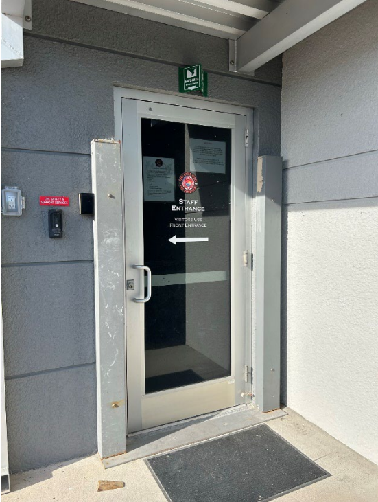
Figure 5-35: Stop logs/flood barriers for the Main Entrance (Lee County, Zone AE)
