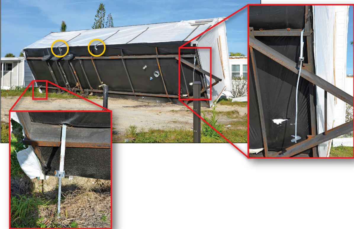
Figure 4-59: Overturned manufactured home that appeared to have been delivered but not yet permanently installed prior to the storm (EWS = 129 mph) (Lee County)
