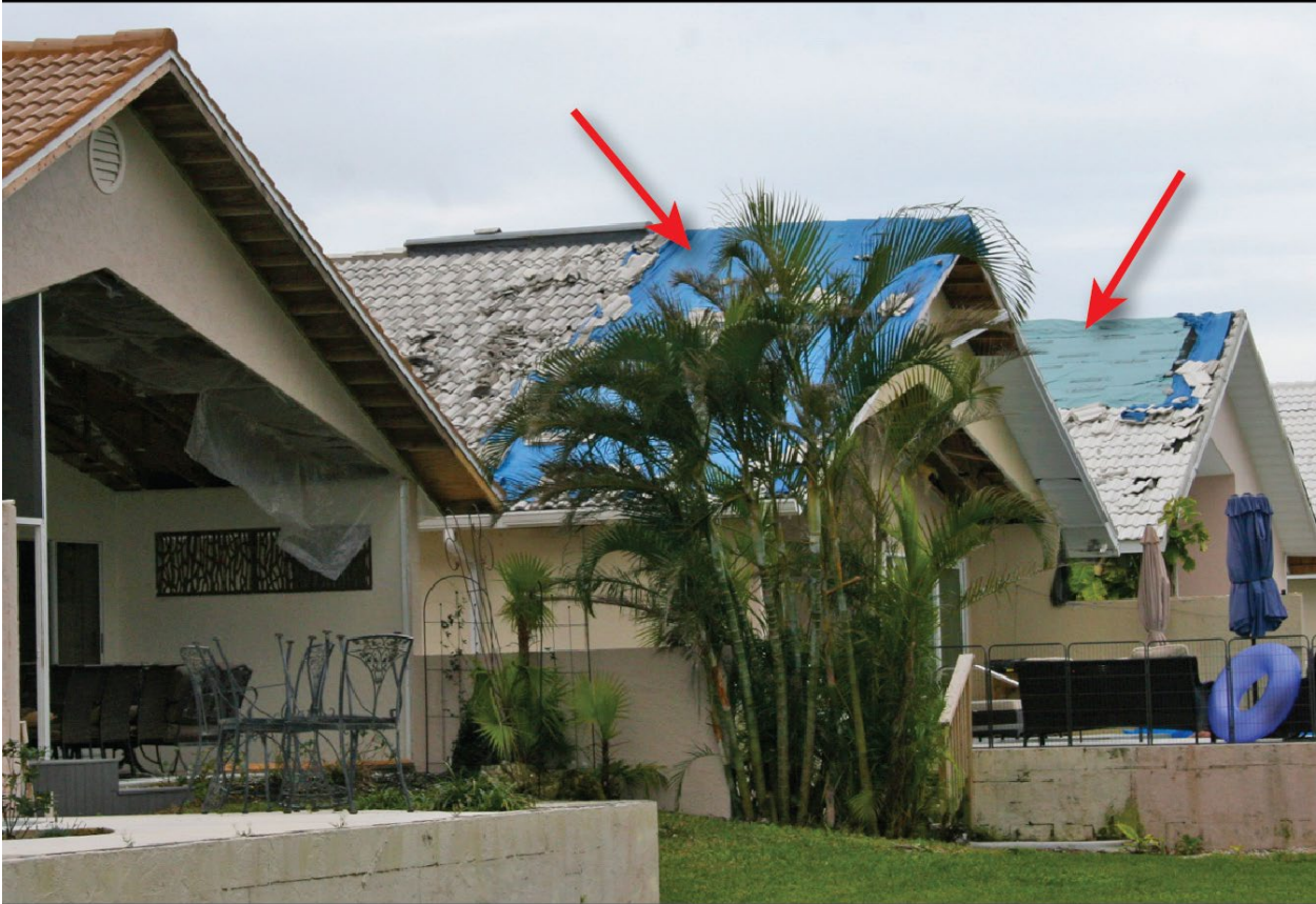
Figure 4-22: Roof tile damage to houses built in 1991/1992 with their original roof covering (EWS: 126 mph) (Placida)
