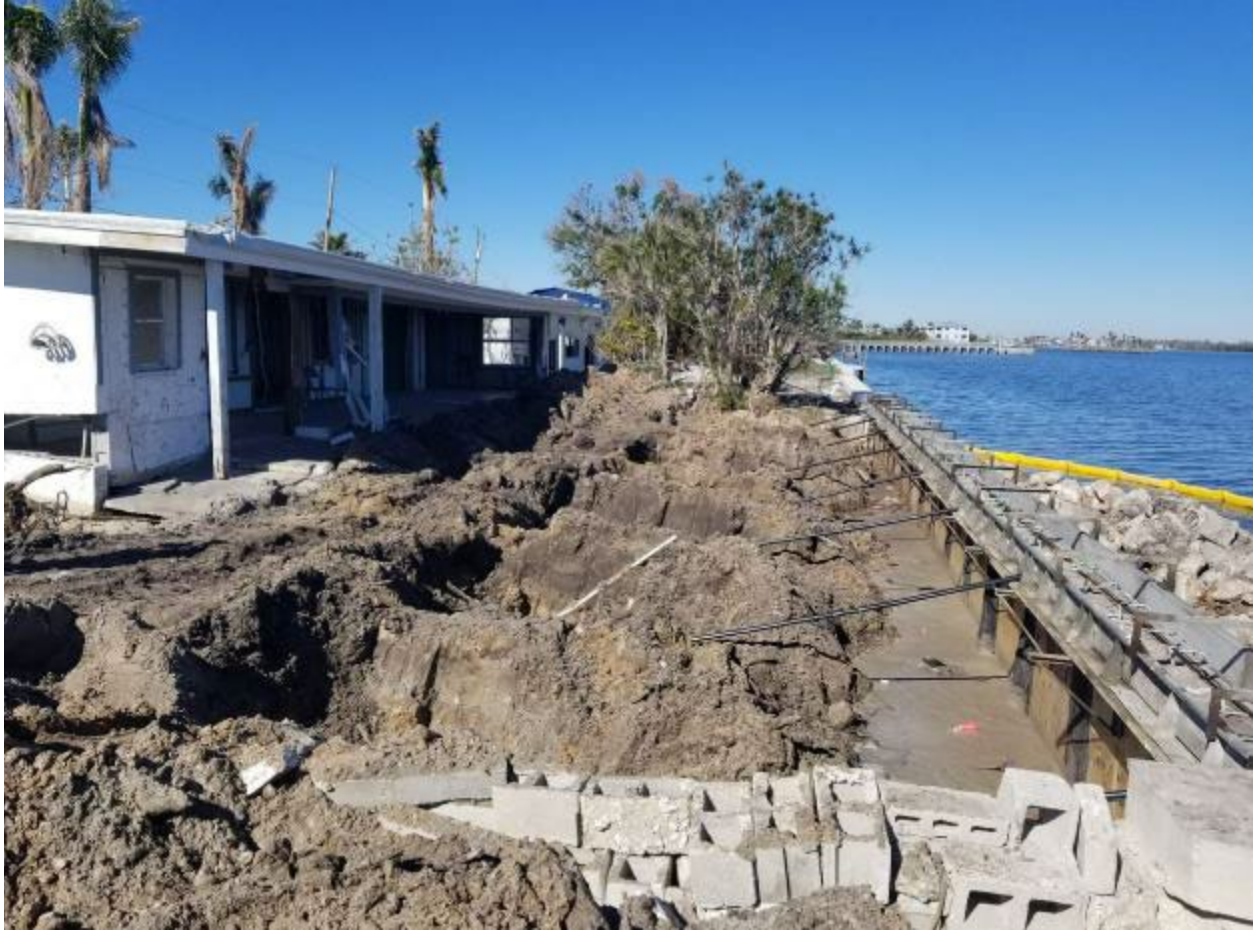
Figure 3-37: New seawall under construction after Hurricane Ian on Matlacha Isle (Lee County, Zone VE)
