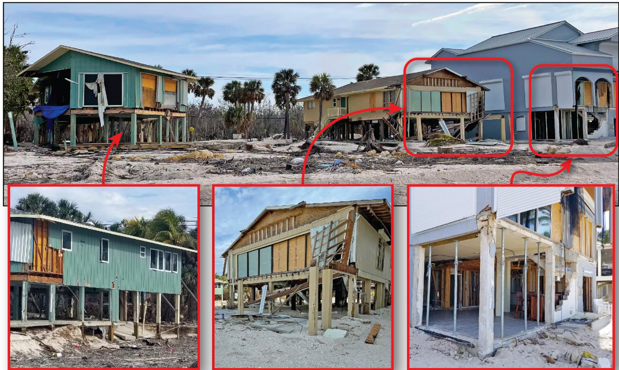
Figure 2: Image (top) shows waterfront houses damaged by coastal flood effects such as waves and velocity in Bonita Springs, Florida. Image (bottom left) shows siding damage above the lowest floor and significant scour, image (bottom center) shows complete loss of a deck as well as damage to glass doors, image (bottom right) shows structural damage to a concrete column and complete loss of a porch.
