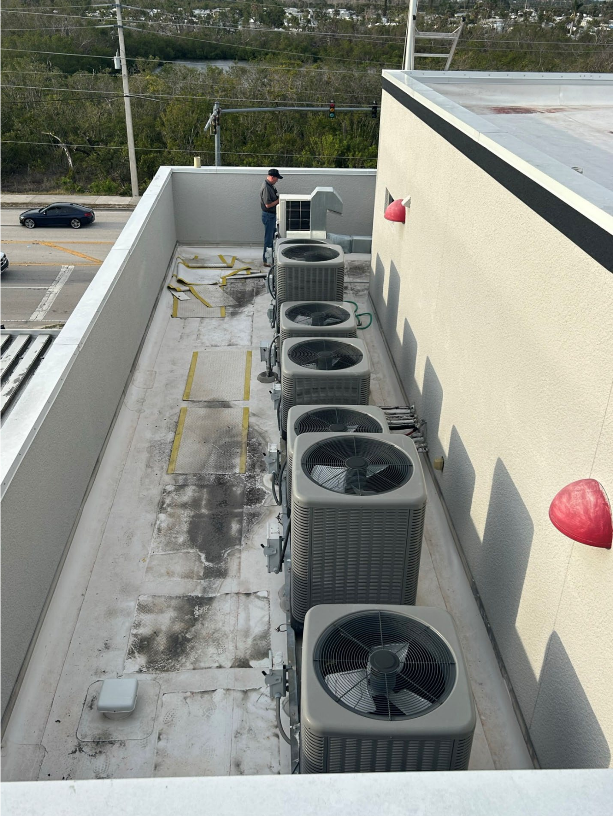
Figure 5-40: Elevated HVAC condensing units (Lee County, Zone AE)
