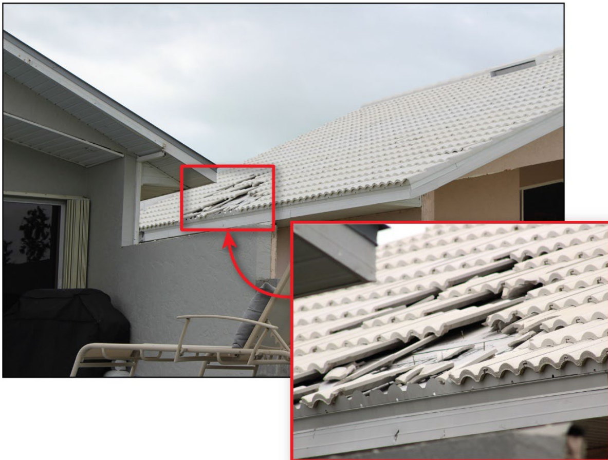
Figure 4-21: A house with a tile roof that was replaced in August 2021 with minor damage near the eave (EWS = 126 mph; DWS = 155 mph) (Placida)
