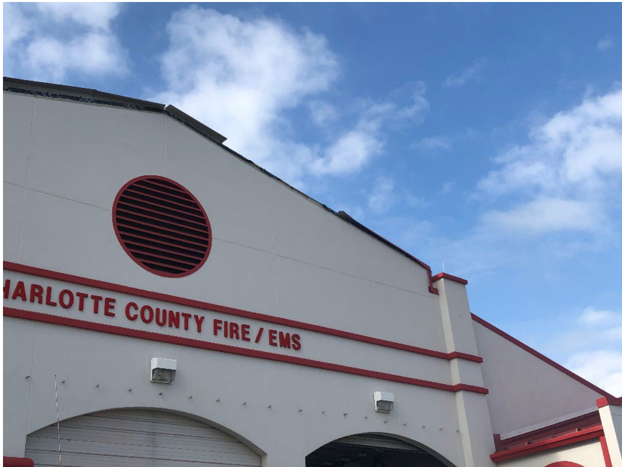
Figure 5-68: Damaged coping above the apparatus bays (Charlotte County)
