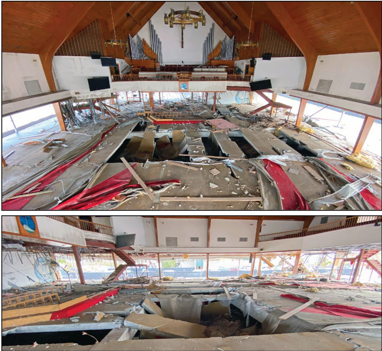
Figure 3-100: Damaged precast concrete floor panels at Chapel by the Sea
