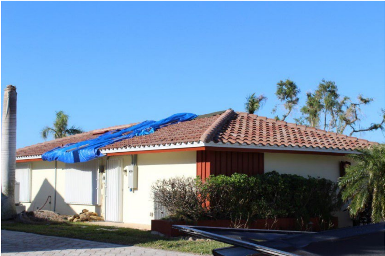
Figure 4-23: A house constructed in 1973 with a tile roof that was replaced in August 2022 with minor damage (EWS = 120 mph) (Pine Island)
