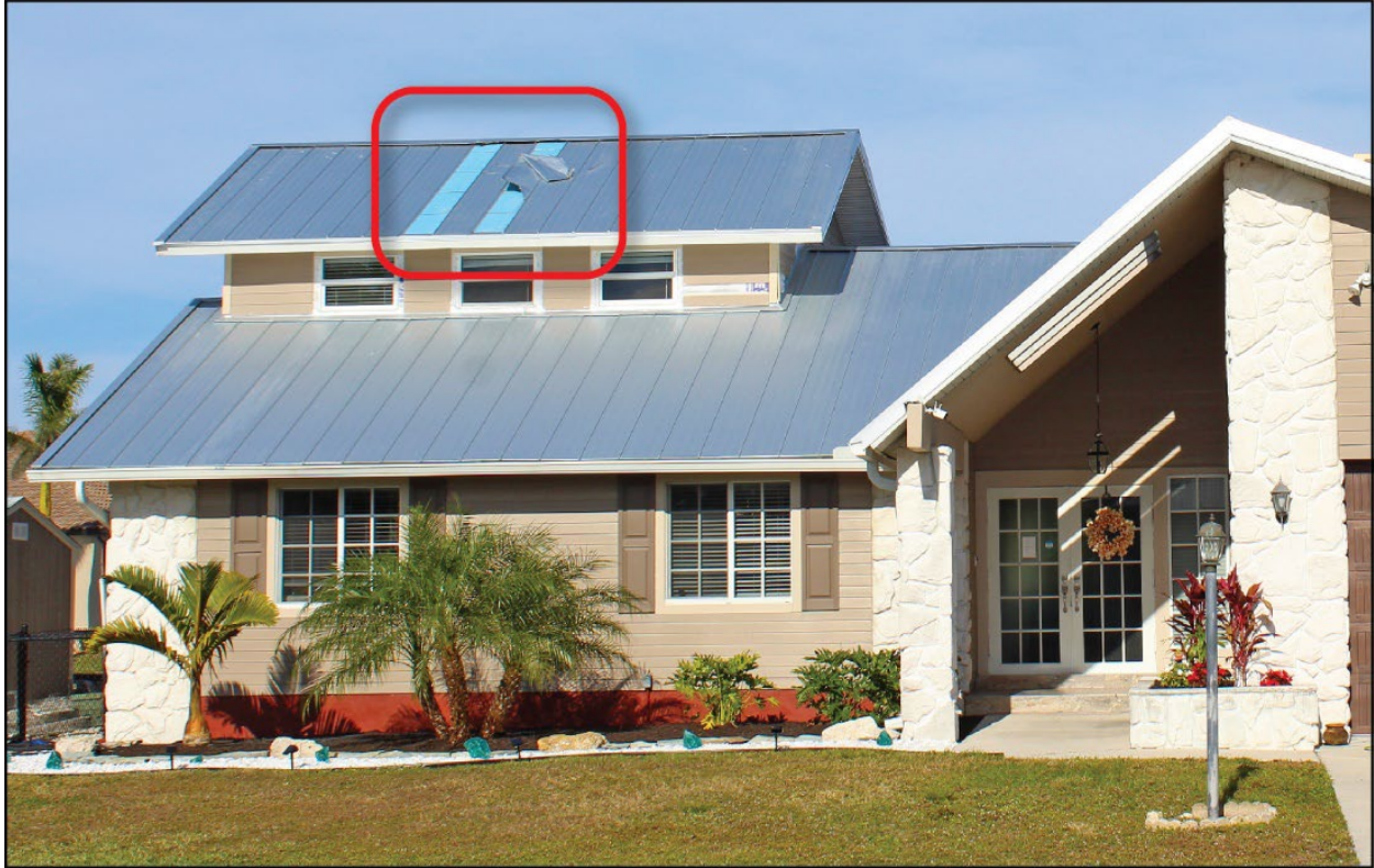
Figure 4-36: A house with metal roof; built in 1984 and reroofed in May 2022 (damage to a few metal panels) (EWS = 128 mph) (Port Charlotte)
