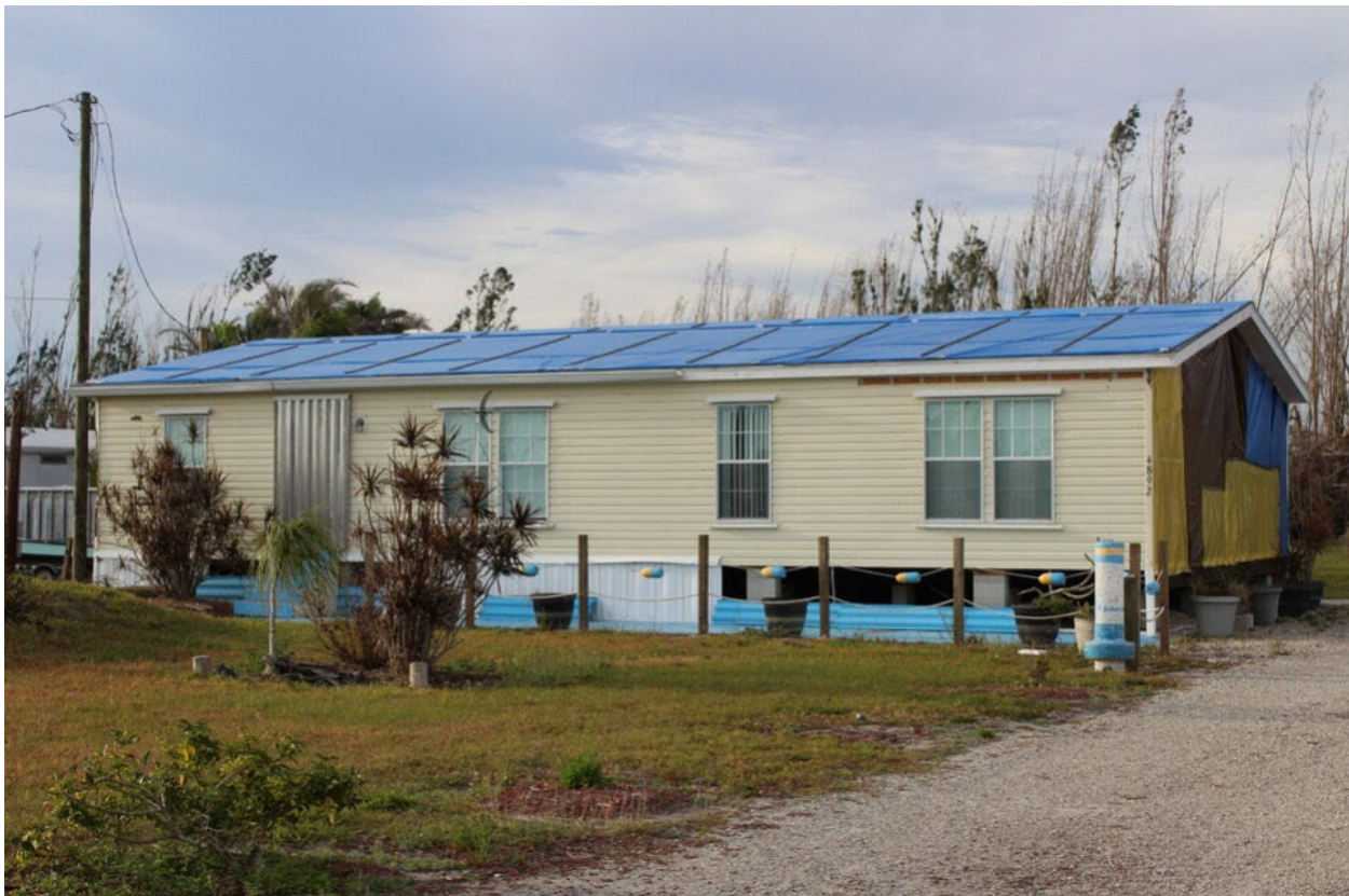
Figure 4-53: Post-HUD manufactured home with roof and wall covering damage (EWS = 118 mph) (Lee County)
