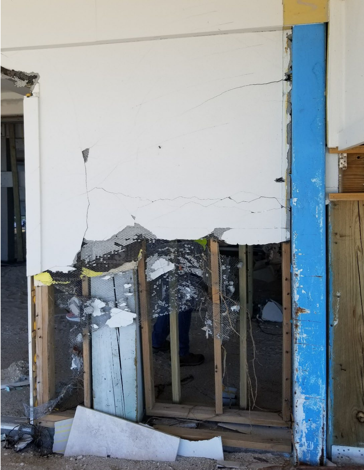
Figure 3-14: Partial failure of shore-parallel breakaway wall on Sanibel Island (Lee County, Zone VE, Seaward of CCCL)
