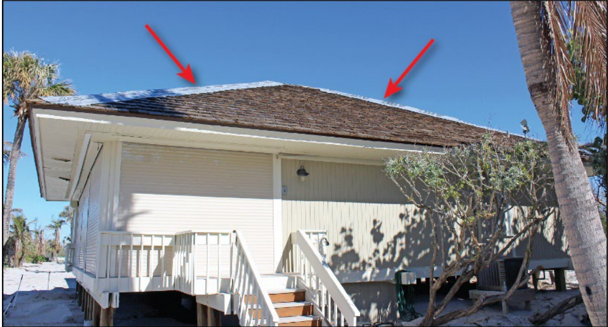
Figure 4-19: A house built in 1974 with a roof replacement in December 2021 with minor shake damage at hips (EWS = 123 mph; DWS = 162 mph) (Captiva)
