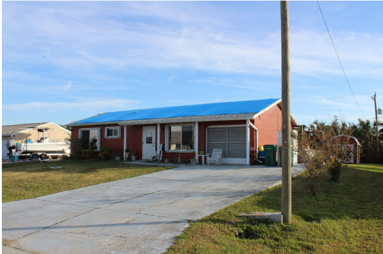
Figure 4-34: A house with asphalt shingle roof damage and tarp to help temporarily prevent water infiltration); built 1984 and reroofed in April 2022 (located in the Port Charlotte neighborhood in Figure 4-31) (EWS = 127 mph)
