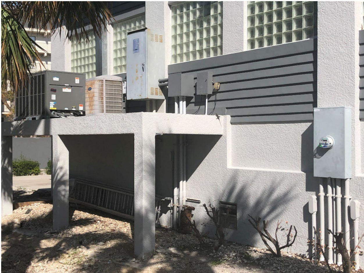
Figure 5-31: Equipment elevated on a platform (Lee County, Zone AE)
