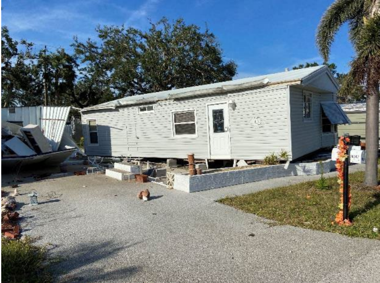
Figure 3-111: Manufactured home displaced from its foundation by flood loads (Lee County, Zone AE)
