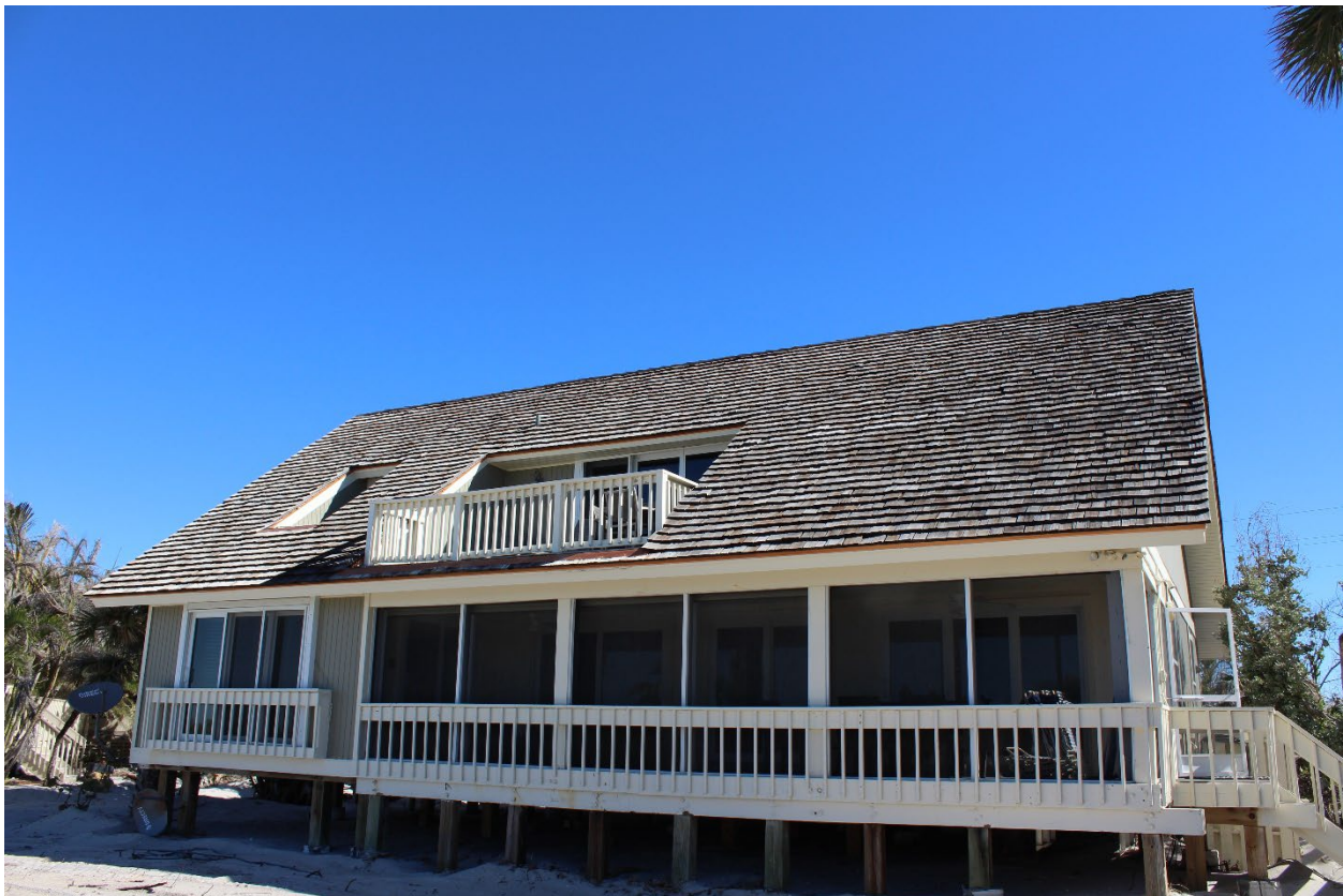
Figure 4-17: A house built in 1974 with a roof replacement in October 2019 with minor shake damage below the balcony (EWS = 123 mph; DWS = 162 mph) (Captiva)
