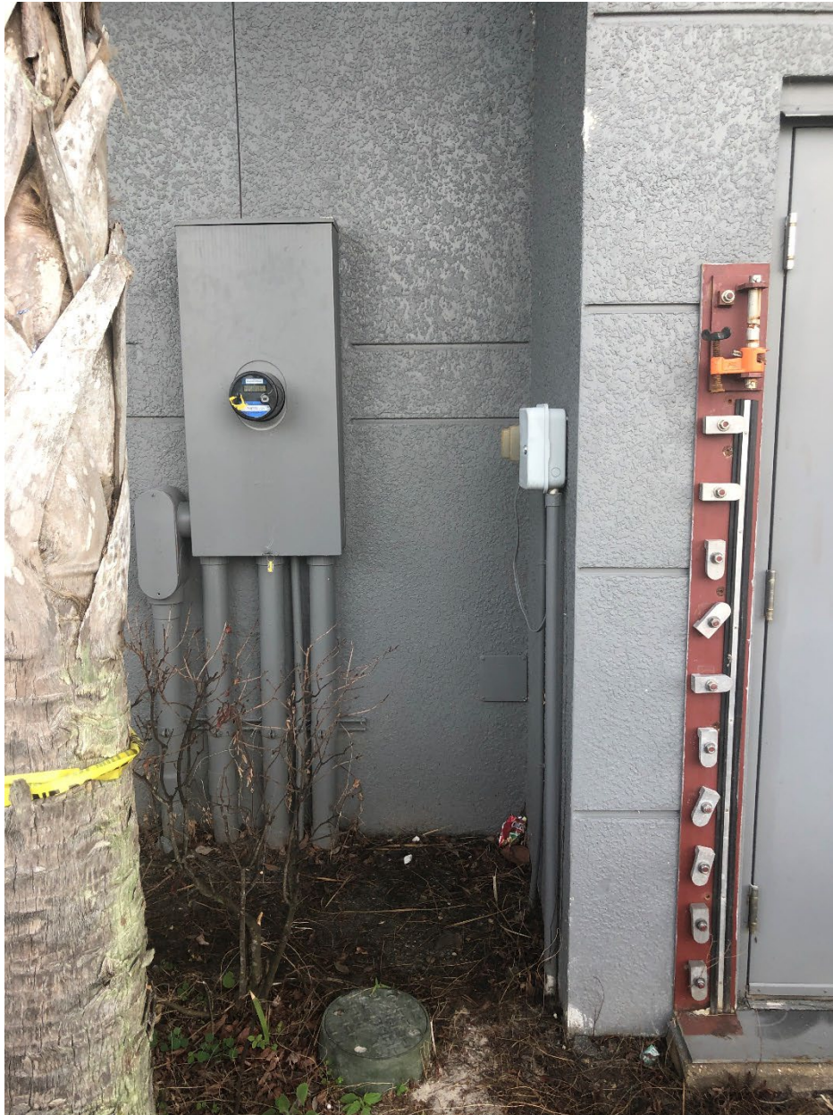
Figure 5-41: Electrical utility meter that is not elevated nor protected by dry floodproofing (Lee County, Zone AE)
