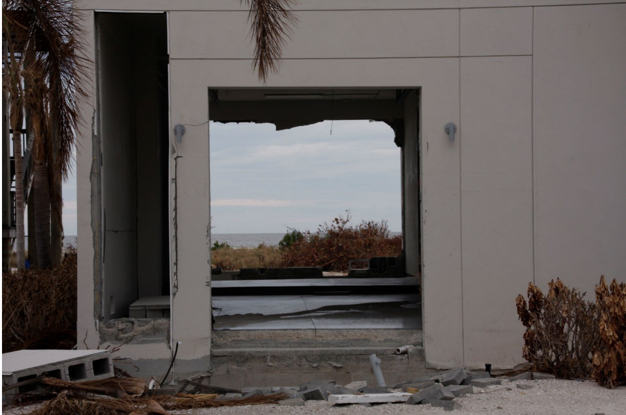
Figure 3-12: CMU breakaway wall in Fort Myers Beach (Lee County, Zone VE, Seaward of CCCL)
