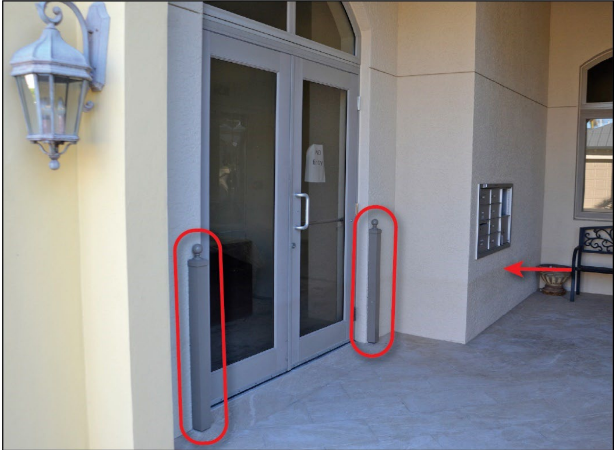
Figure 3-70: Office building where dry floodproofing measures were not deployed; note HWM (arrow) and posts for dry floodproofing measures (circled) (Collier County, Zone AE)
