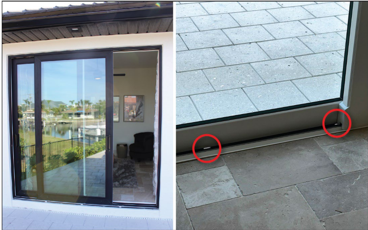
Figure 4-10: A house built in 2021 with a two-panel sliding glass door that experienced significant water intrusion due to wind-driven rain (the two red circles identify weepholes that enable water to exit) (EWS = 130 mph; DWS = 151 mph) (Punta Gorda)
