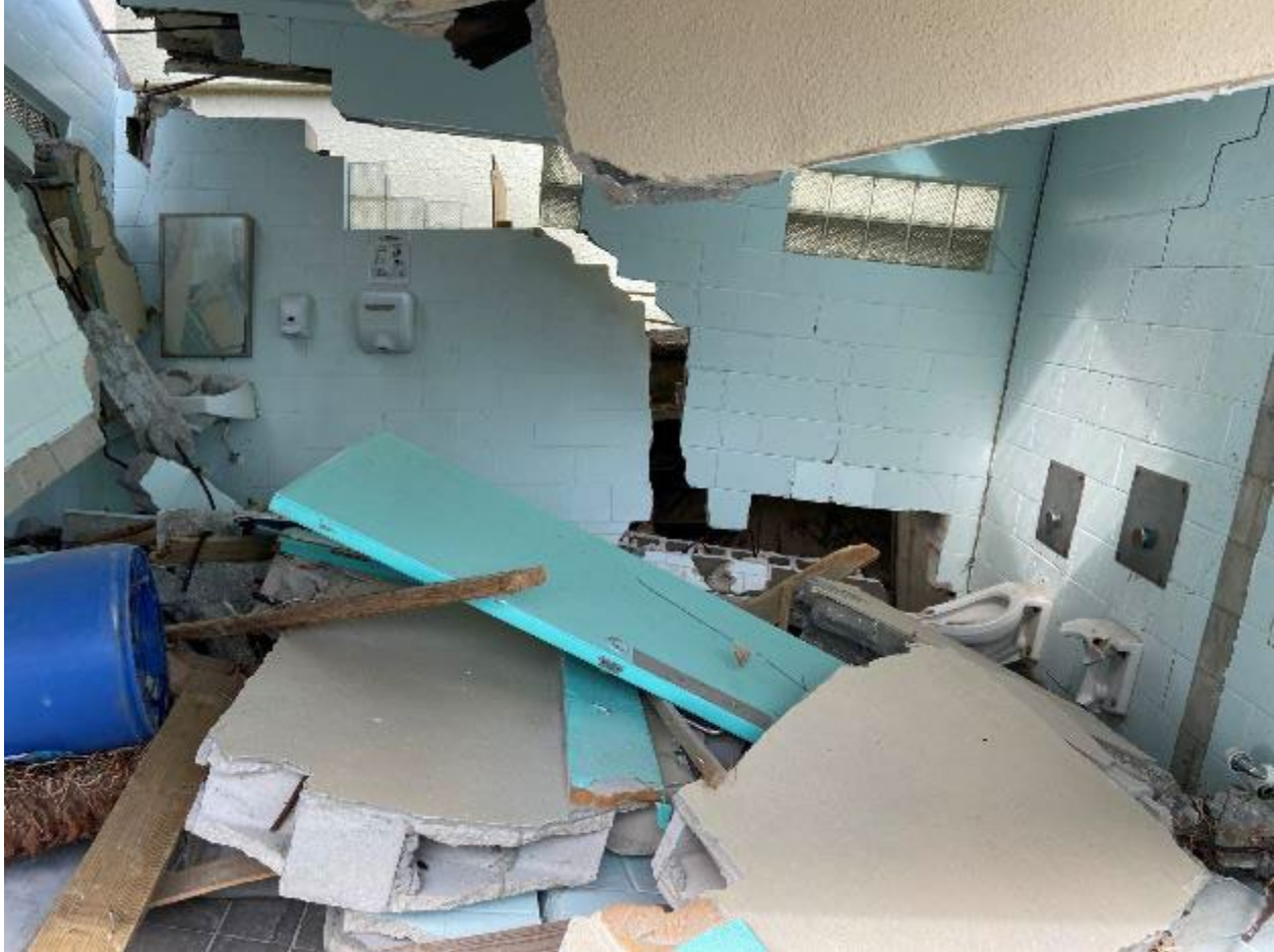
Figure 3-109: Interior of destroyed public restroom in Daytona Beach Shores (Volusia County, Zone VE, Seaward of CCCL)
