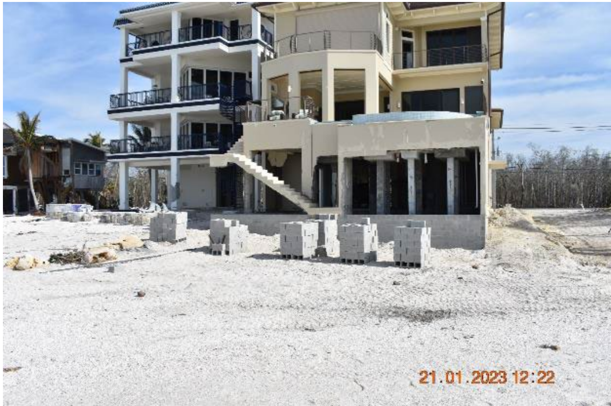
Figure 3-16: Staging of repairs to CMU breakaway walls in Bonita Beach (Lee County, Zone VE, Seaward of CCCL)
