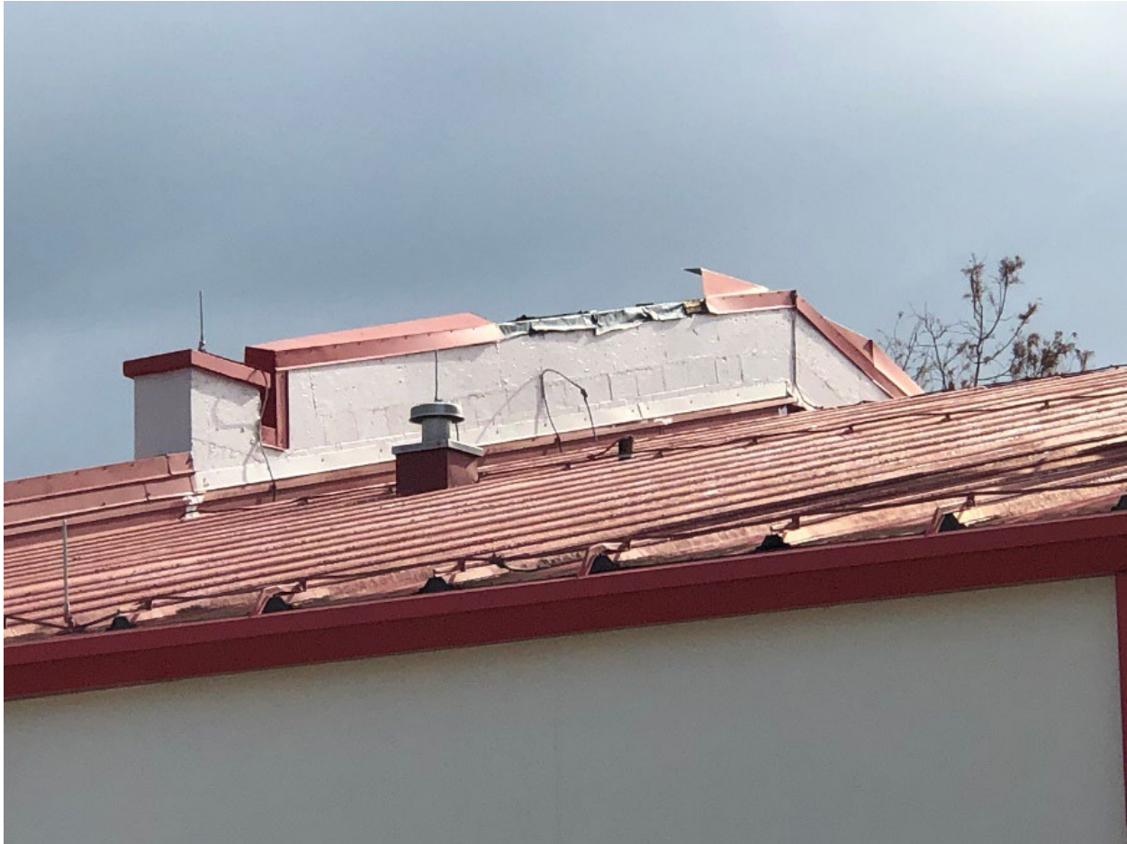
Figure 5-69: Damaged coping above the apparatus bays (Charlotte County)
