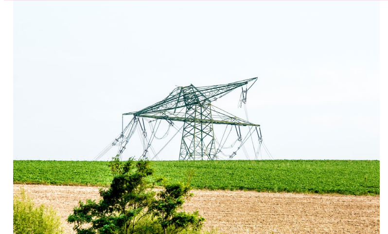
Serious storm damage on a high voltage power line after a strong storm
