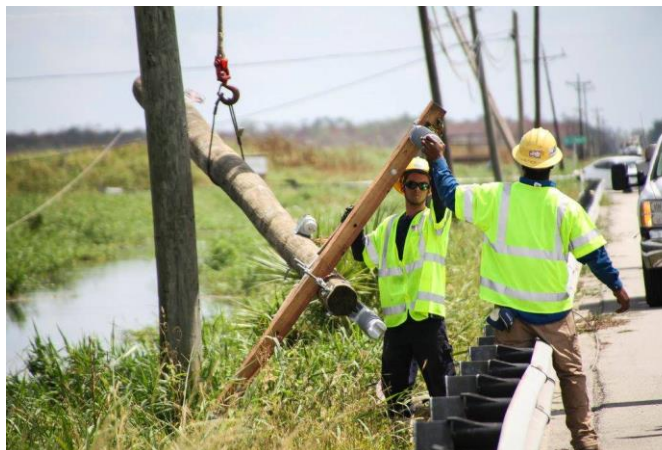
Workers install a new utility pole in Everglades City after Hurricane Irma. (FEMA, 2017)
