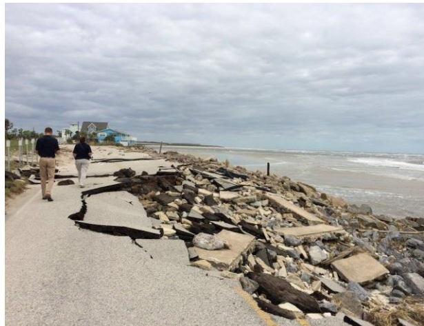
FEMA Officials Survey Damage on Highway A1A near Saint Johns County, Florida (FEMA, 2016)
