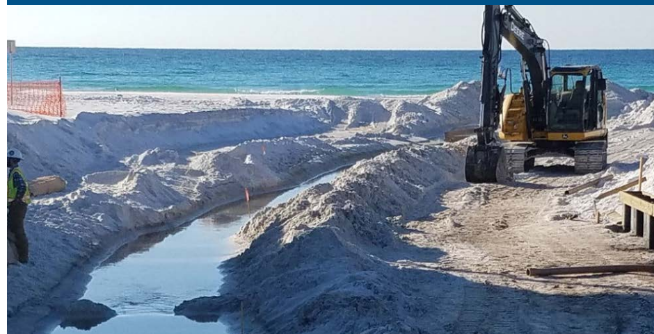
Erosion and sedimentation caused by previous storms and urban growth were straining Oyster Lake's outfall
