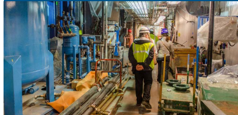
NYU Langone Medical Center Generators Source: FEMA
