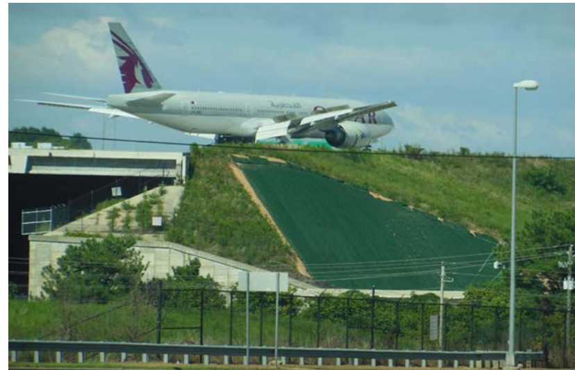
An Engineered Earth Armoring System was used to stabilize the slope and promote vegetation. Source: Propex Geosolutions
