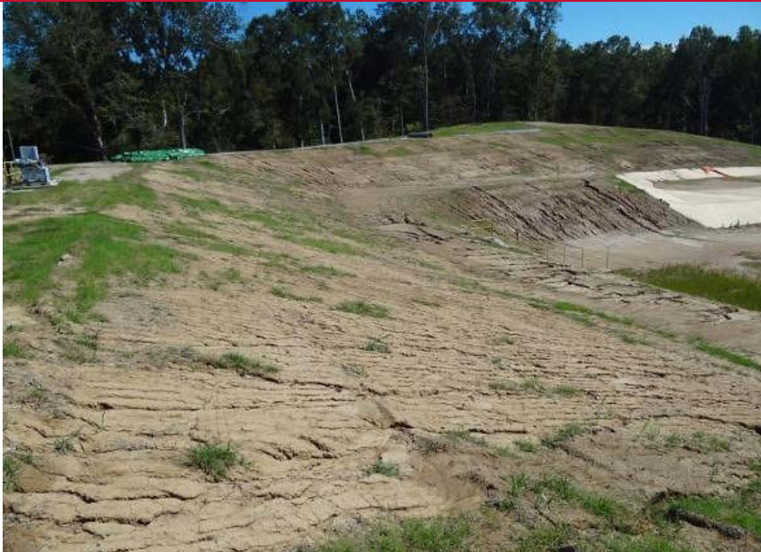
The USACE Rapid Repair Levee Breach facility was experiencing extreme erosion due to heavy rainfall.
