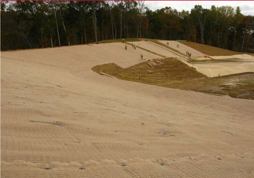
More than 5,000 square yards of an EEAS was installed to provide resilient flood protection.
