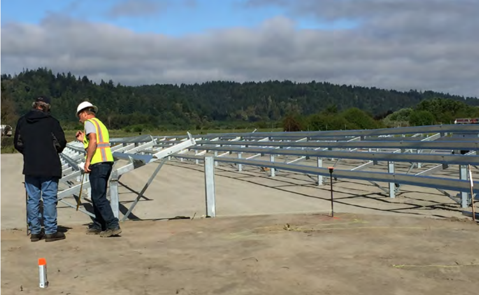
Workers installing the racking for the Blue Lake Rancheria’s 500-kilowatt solar system in June 2016. The solar system is a cornerstone of the tribe’s low-carbon community microgrid project.
