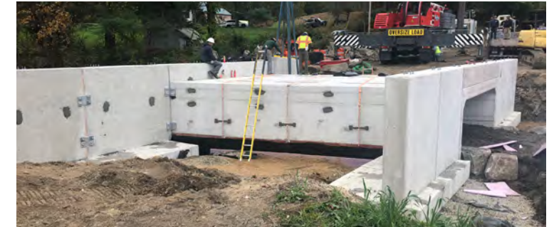
Installation of the last wingwall of the replacement structure Source: Peter Steckler, use by FEMA is permitted
